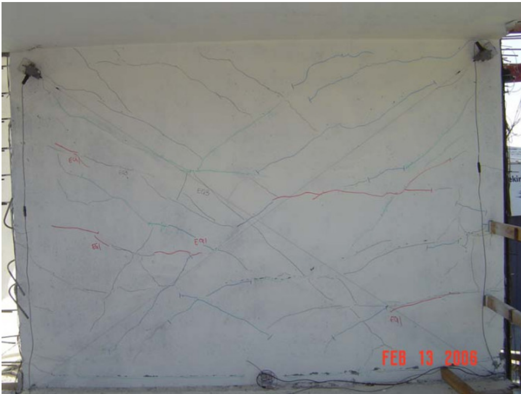
Figure 100 UCSD 7-Story Shake Table Test – Crack pattern after full protocol – Level 2
