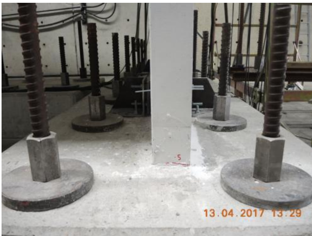
Figure 182. Crack pattern at the base of lateral wall W1L3 – North side, external edge.
