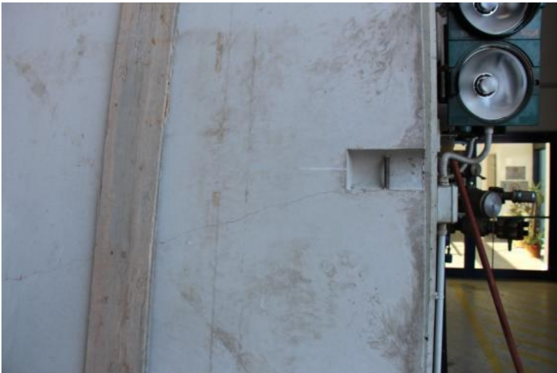
Figure 21. Detail of pre-cracked stability wall – crack running through the entire wall width and depth.
