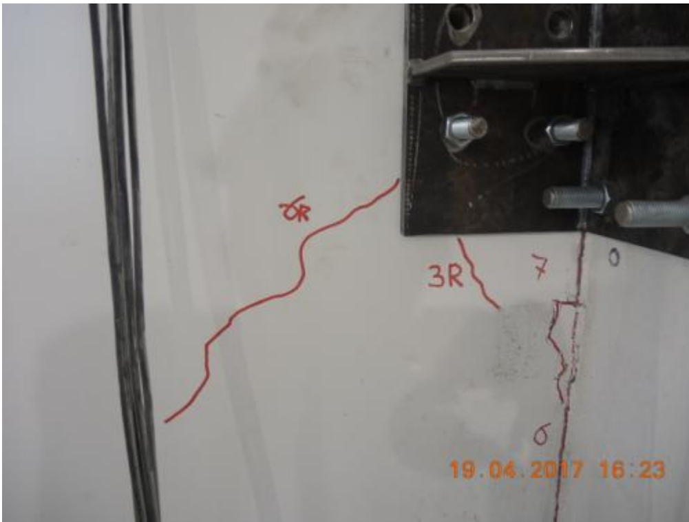
Figure 269. New crack in one of the transversal walls (internal face) – Below the steel angle.
