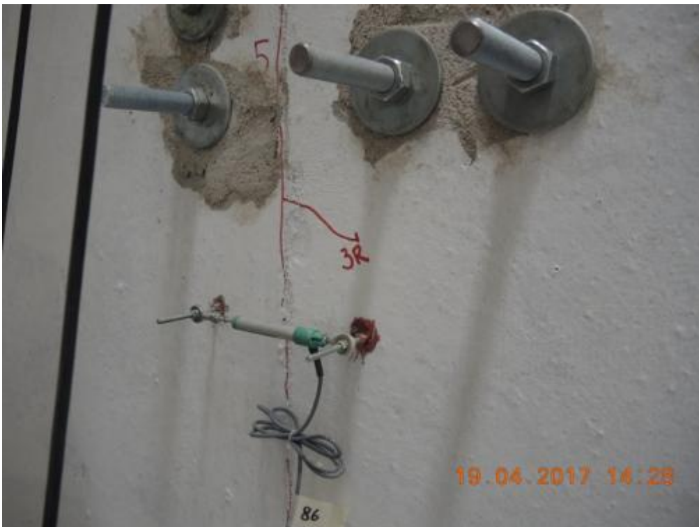
Figure 263. Crack pattern of the transversal walls (external/South face) – Below the high-strength rods.
