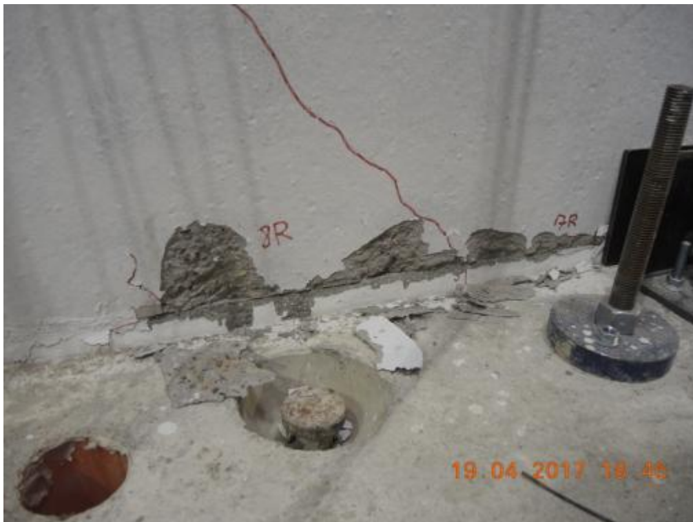
Figure 308. Detail of the base of lateral wall W1L1 after removal of crushed concrete – West side, South face.
