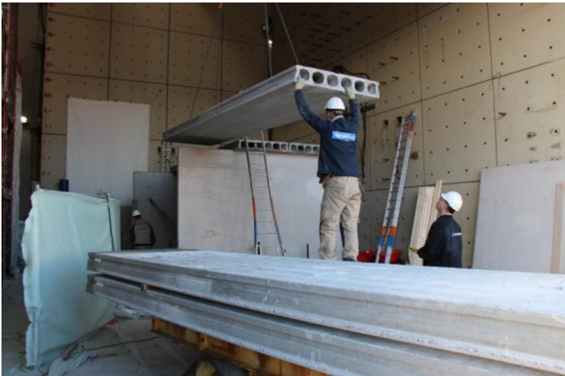
Figure 23. Uplift and installation of precast hollow core slabs composing the first floor.
