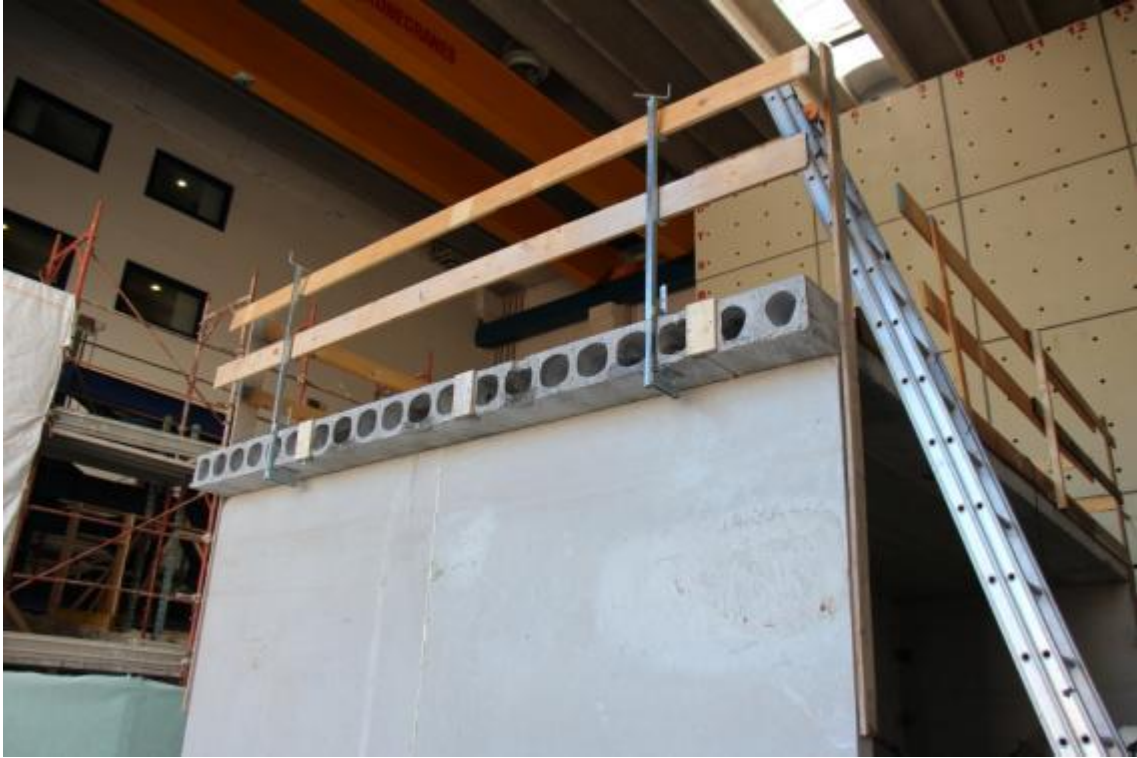
Figure 38. Installation of safety measures and preparation of mock-up for assemblage of second storey.
