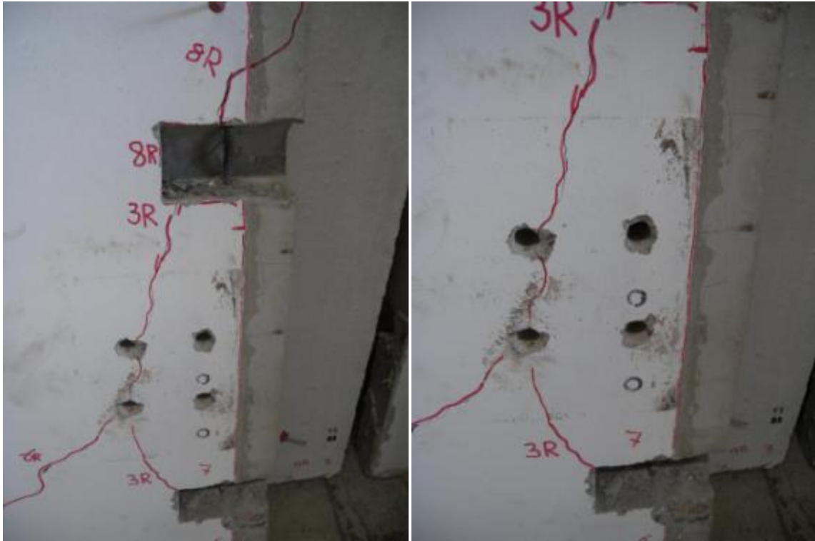
Figure 369. Global and enlarged view of cracks beneath the steel plate of a clip angle.
