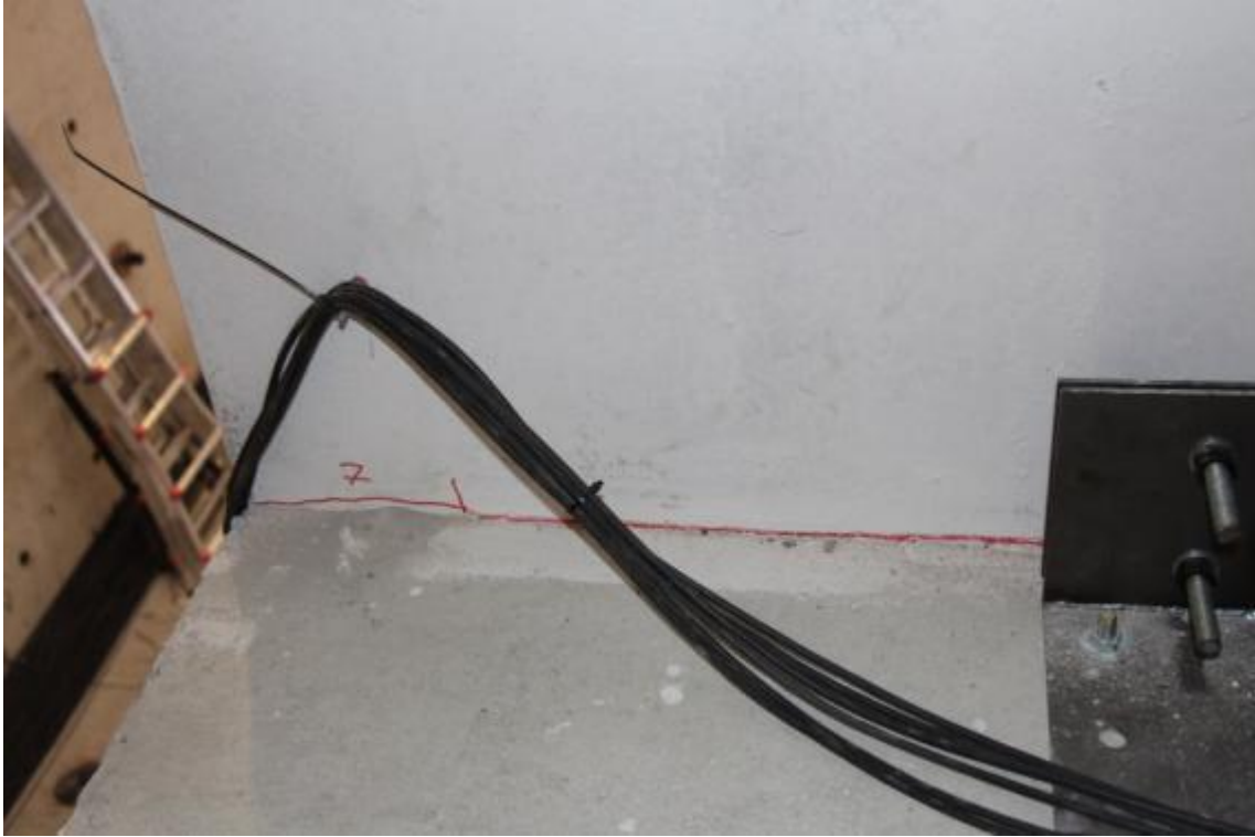
Figure 208. Crack pattern at the base of the transversal walls – North side, second floor, internal face.
