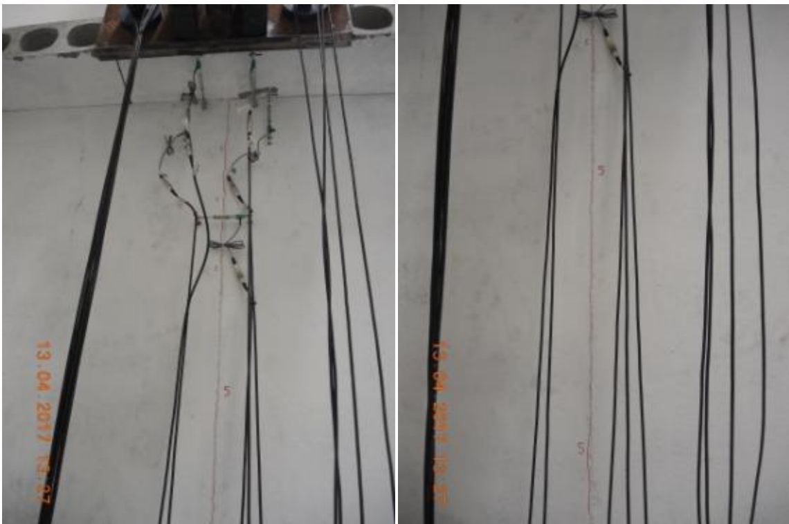
Figure 184. Three-way connection: development of a new crack at the two adjacent lateral walls.
