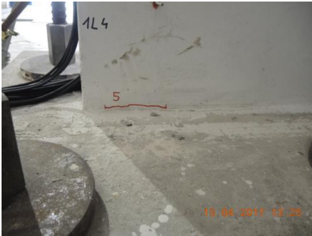
Figure 181. Crack pattern at the base of lateral wall W1L4 – North side, internal edge.
