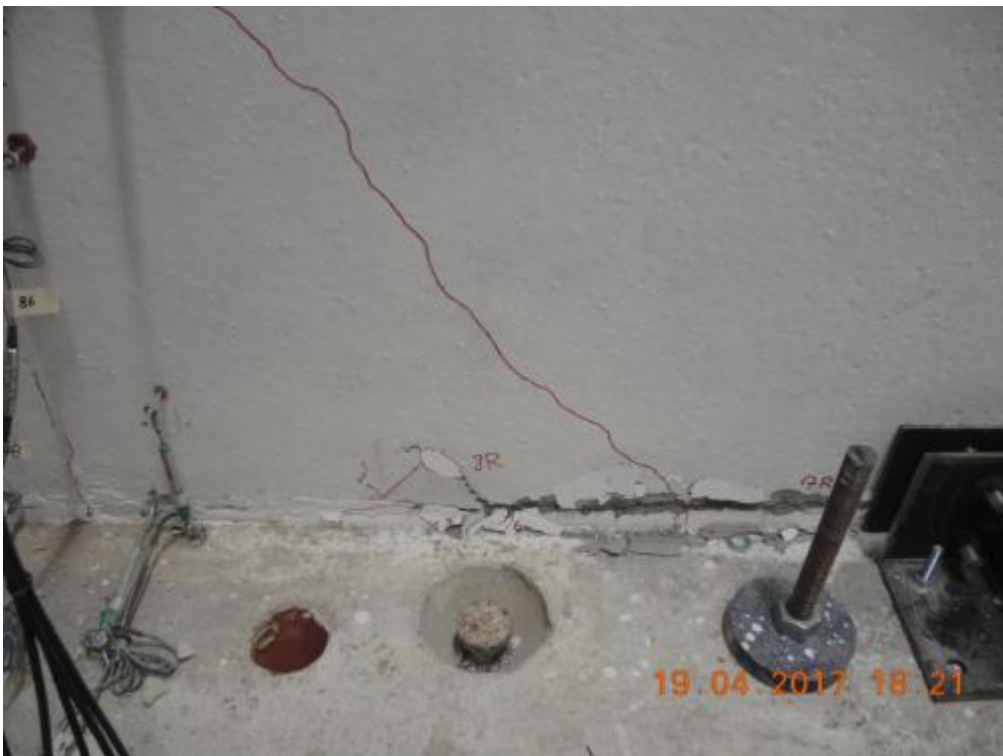
Figure 298. Detail of inclined crack in the transversal wall W1L1 – West side, South face, base.
