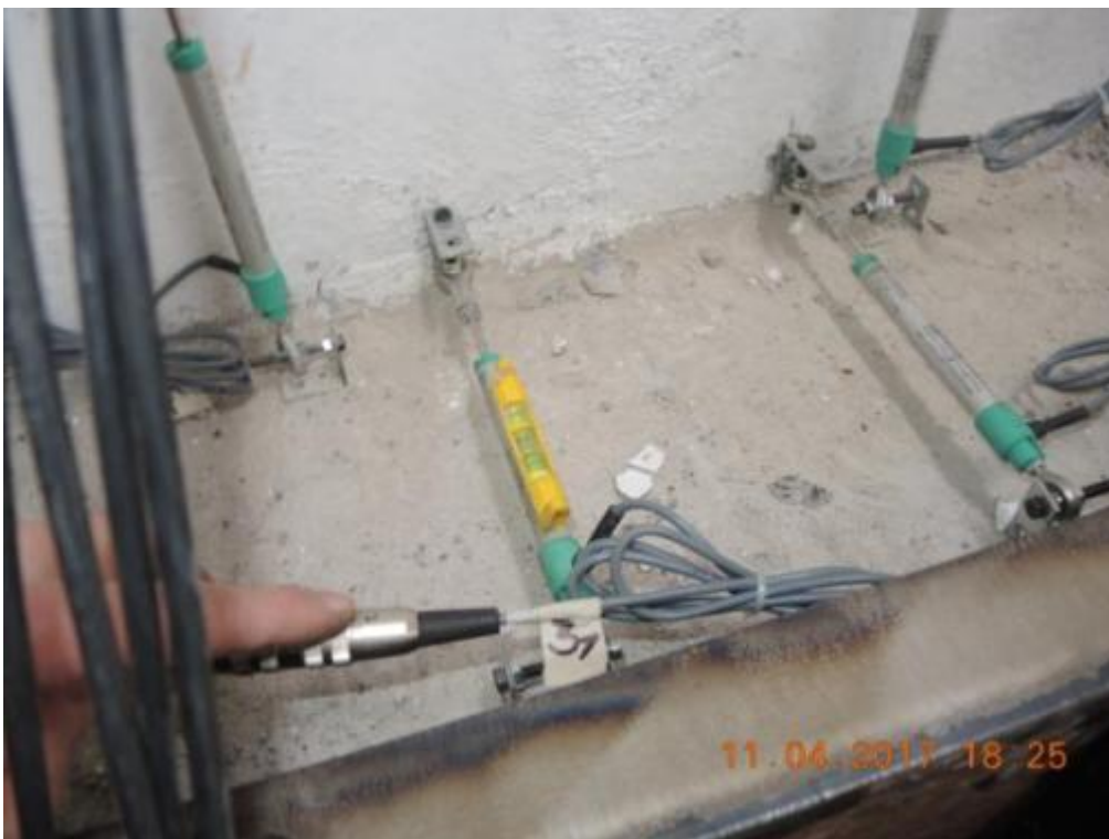
Figure 116. Instrumentation at the base of the lateral walls – Central zone, second storey, adjacent panel.
