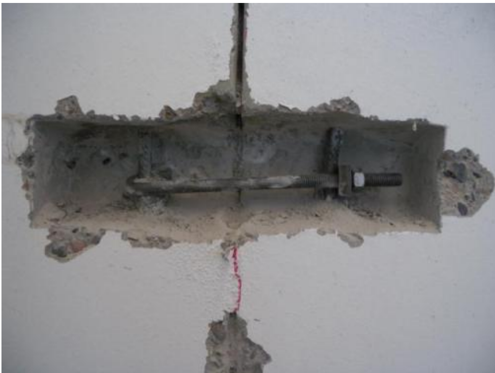
Figure 345. Detail of hook reinforcement after removal of grout around it – Lateral walls, first storey.
