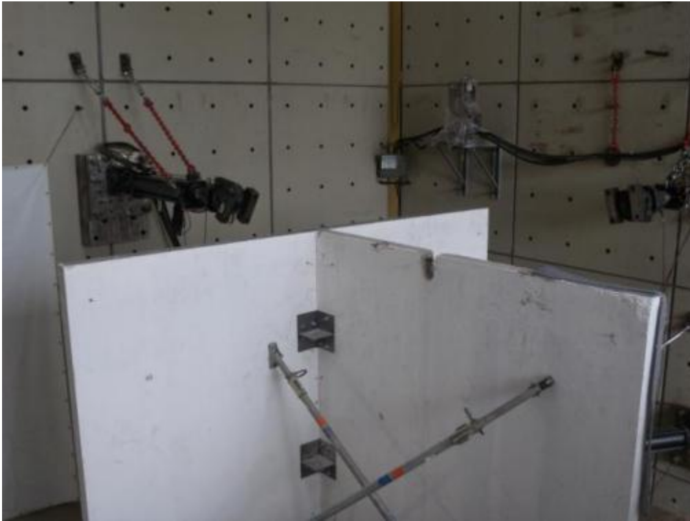
Figure 333. Detail of fabric felt underneath the second-floor slab – Stability wall, North side.
