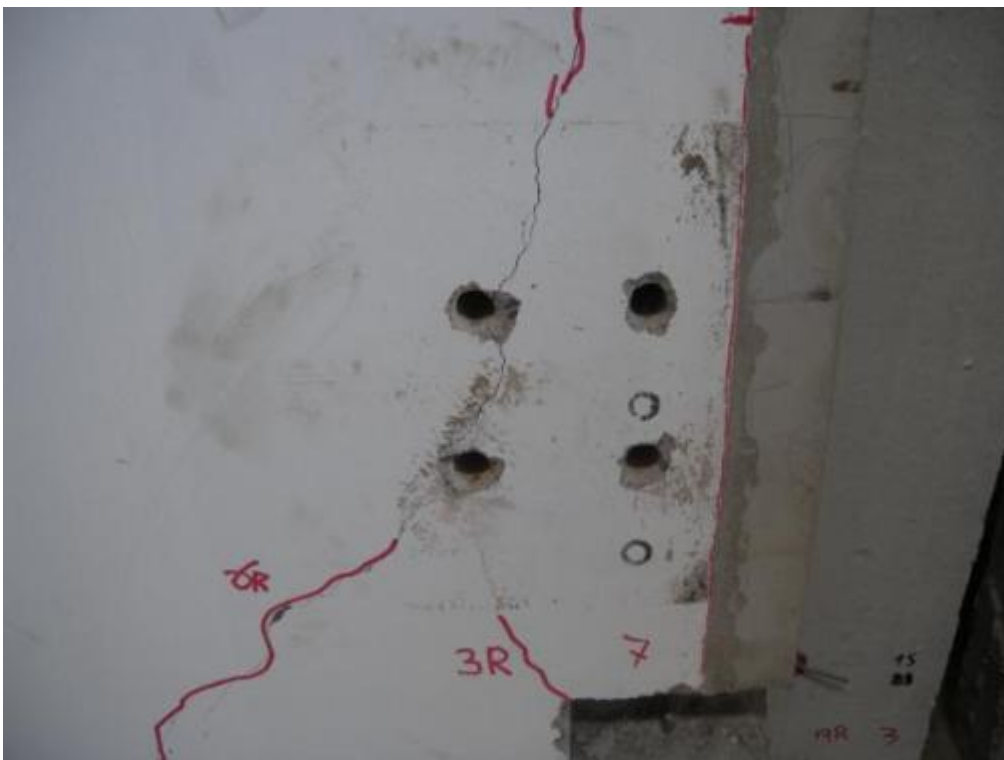
Figure 368. Detail of crack pattern after dismantling of steel angles.
