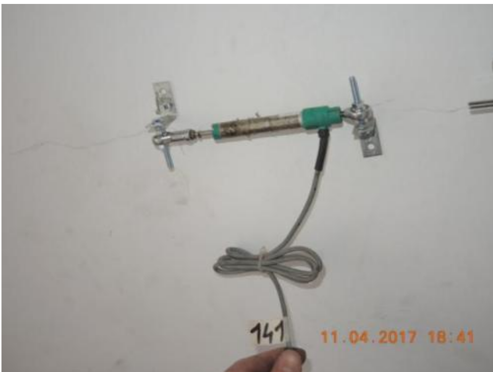
Figure 130. Potentiometer for monitoring of crack opening – 25 mm-stroke instrument.
