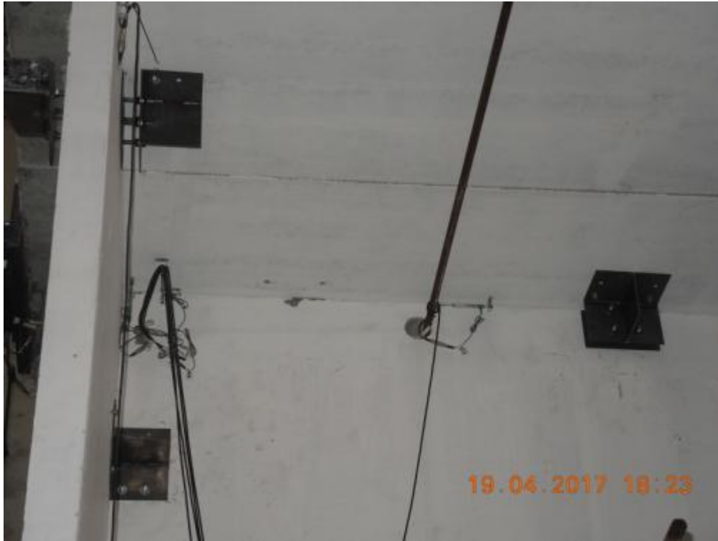
Figure 301. Detail of post-tensioned bar at the top of the second-storey stability wall – East side.
