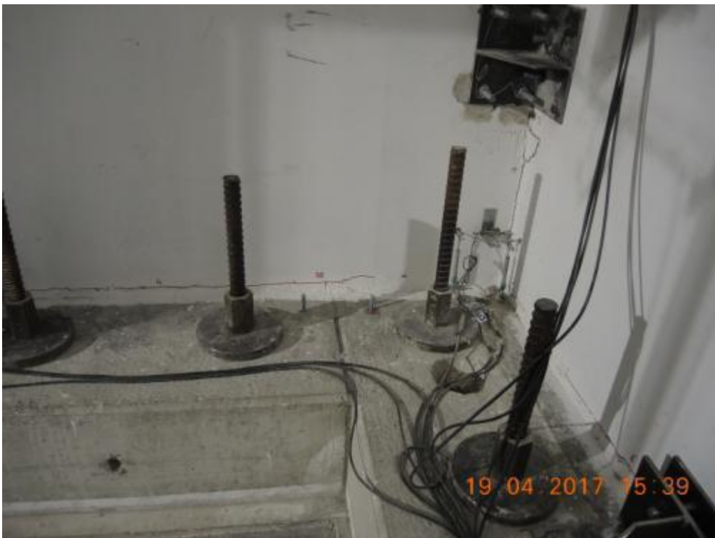
Figure 267. Propagation of crack pattern at the base of the ground-floor stability wall – West side.
