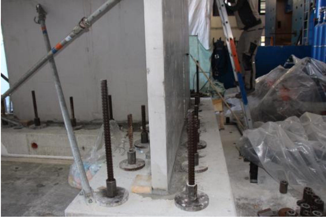
Figure 32. Detail of the mortar joint at the base of the opposite lateral wall – global view.
