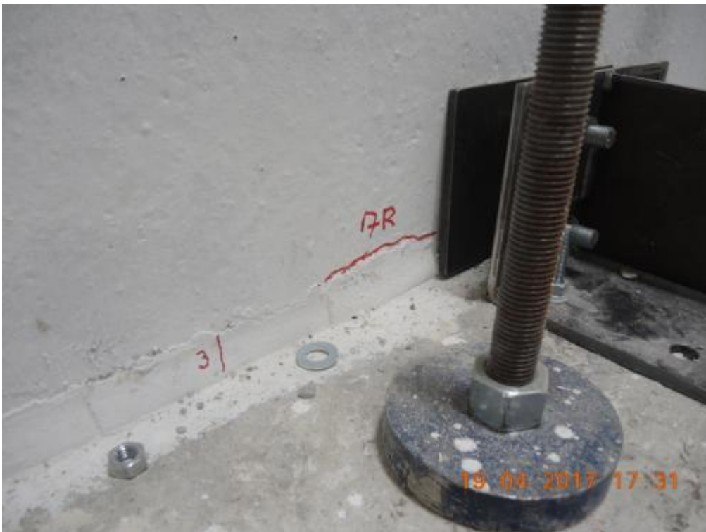
Figure 285. Detail of a minor crack close to one of the sliding restrainers – South side, lateral wall.
