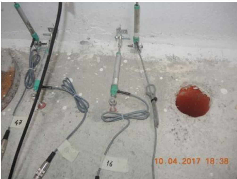
Figure 106. Instrumentation at the base of lateral walls – Central zone.
