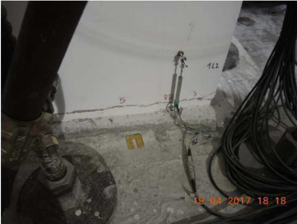
Figure 291. Damage at the base of lateral wall W1L2 – East side, first floor.
