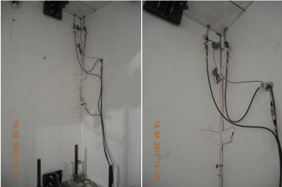
Figure 190. Detachment of stability wall with respect to lateral walls – global view and detail at the top.
