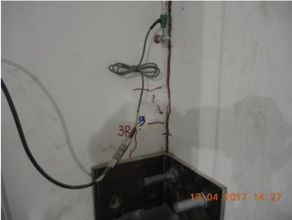
Figure 262. Development of new cracks in the transversal walls (internal face) – Above the steel angle.
