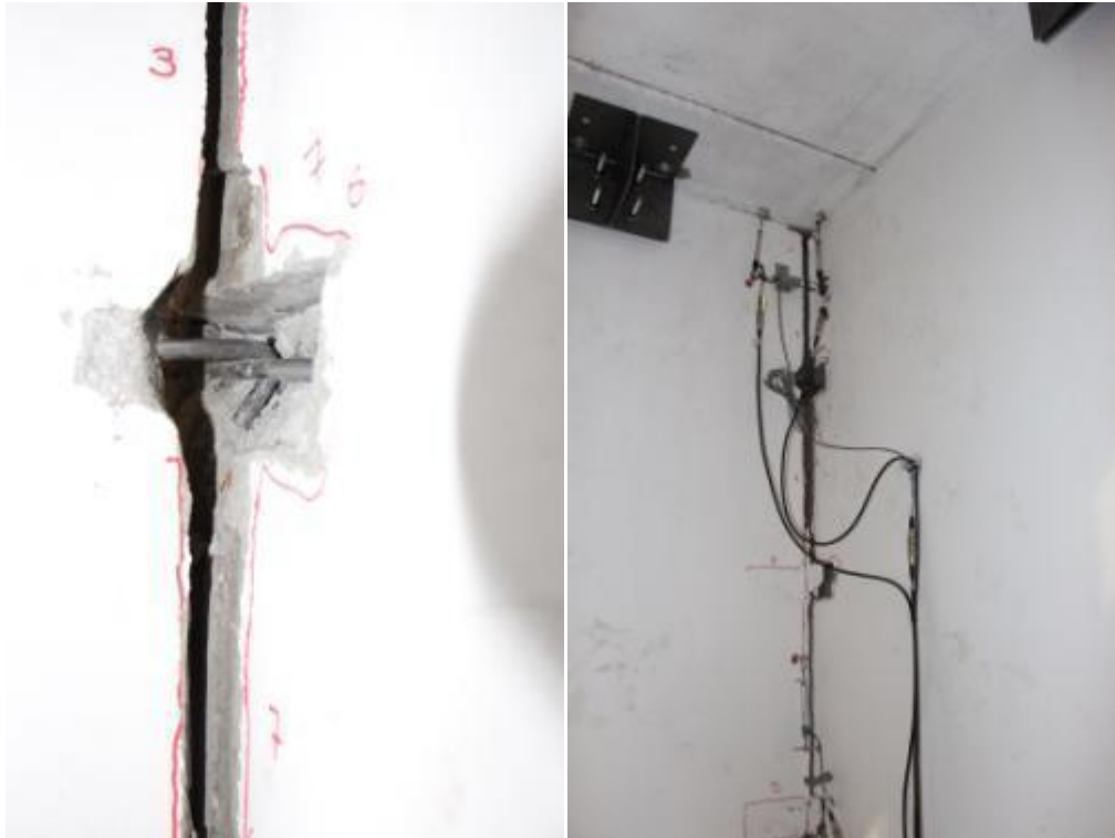
Figure 212. Damage of the three-way joint at the end of testing – Global and enlarged views.
