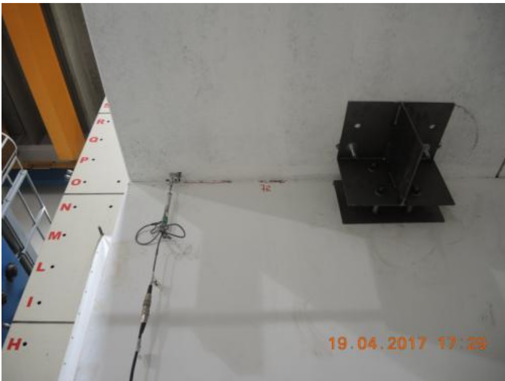
Figure 279. Minor friction-induced concrete chipping at the top of the first-storey transversal wall.
