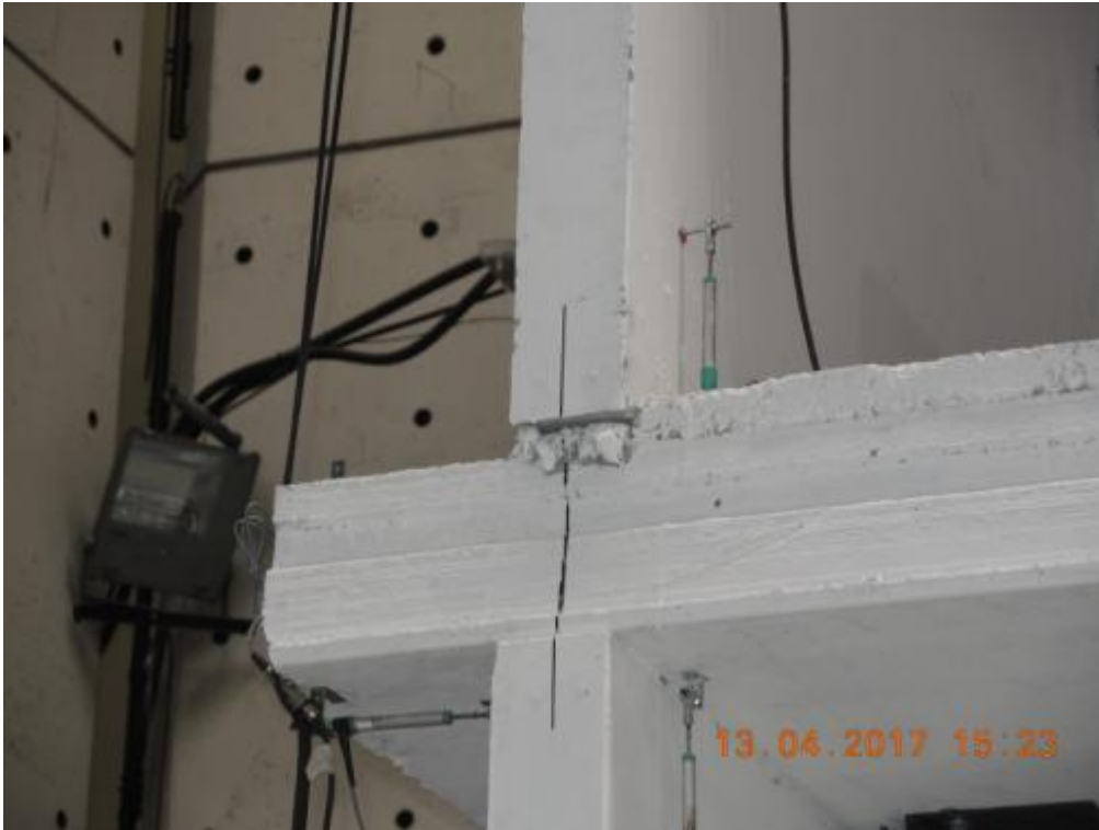
Figure 198. Detail of the first-storey floor slab after Test run #7 – top displacement = 16.8 mm.
