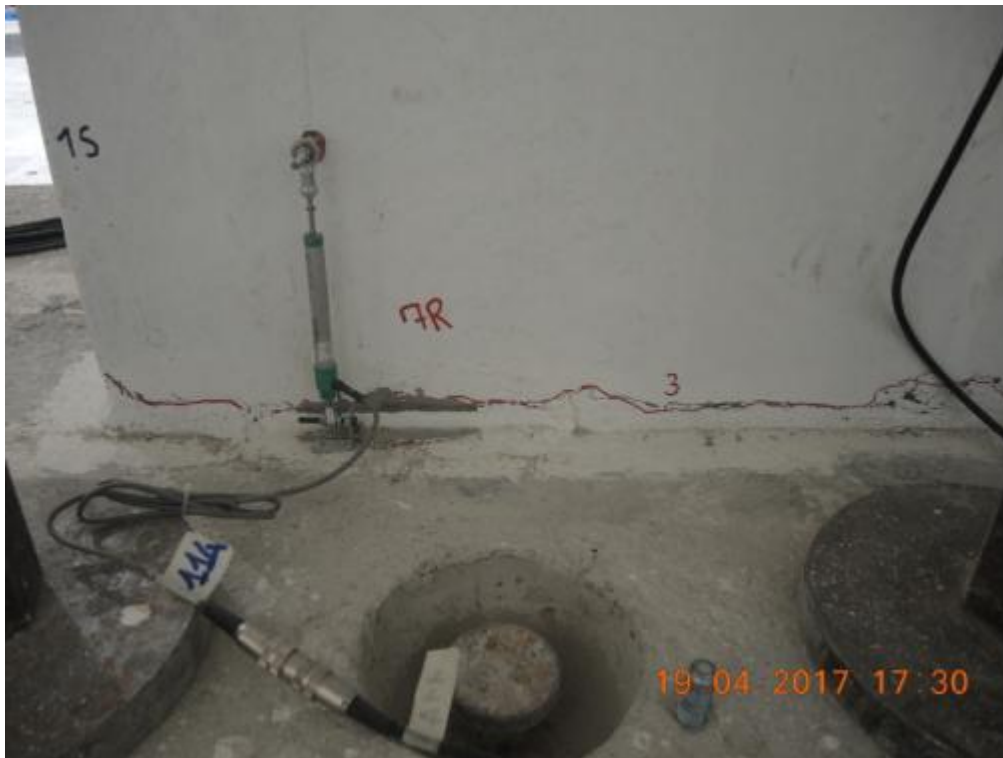
Figure 280. Crack pattern at the base of the ground-floor stability wall – West side, edge.
