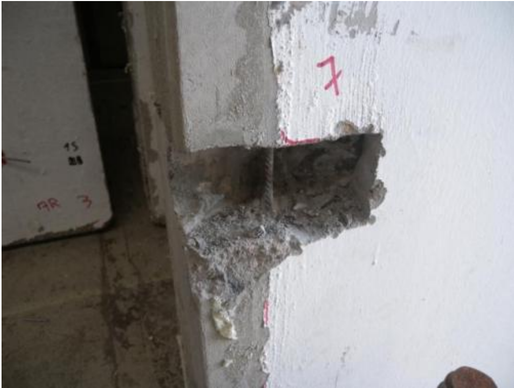
Figure 367. Detail of panel reinforcement passing through the niche of a panel-to-panel connection.
