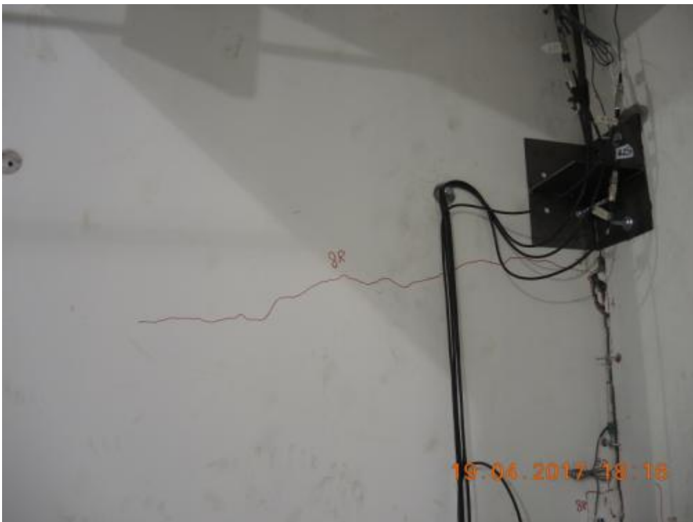
Figure 288. Full-width/mid-height horizontal crack in the transverse wall – Top steel angle, East side.
