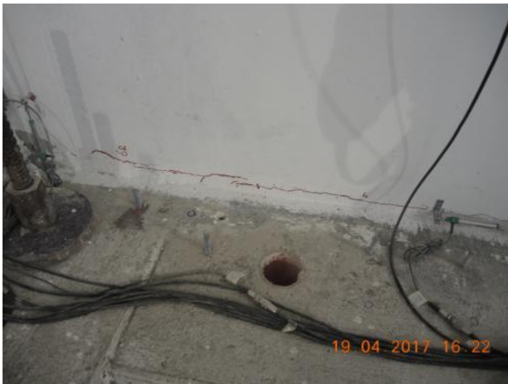
Figure 268. Propagation of crack pattern at the base of the ground-floor stability wall – East side.
