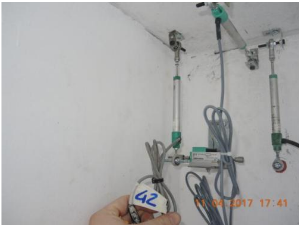
Figure 118. Instrumentation in correspondence to lateral wall-to-stability wall connection – Top of the walls.
