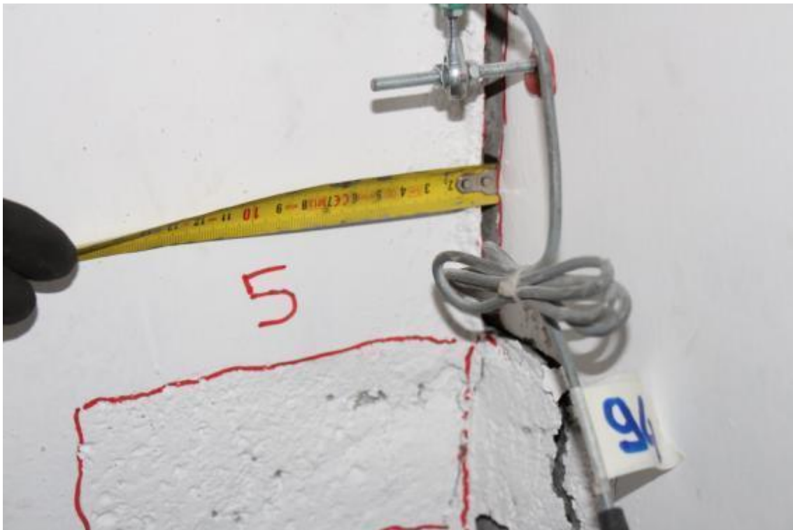
Figure 205. Detail of gap opening between the stability and lateral walls – Mid-height, West side.
