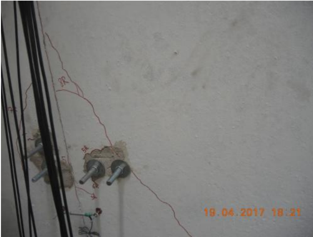
Figure 297. Detail of inclined crack in the transversal wall W1L1 – West side, South face, mid-height.
