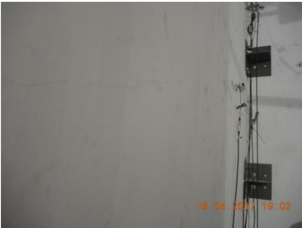
Figure 316. Detail of pre-existing full-depth/full-width/mid-height crack in the second-storey stability wall.
