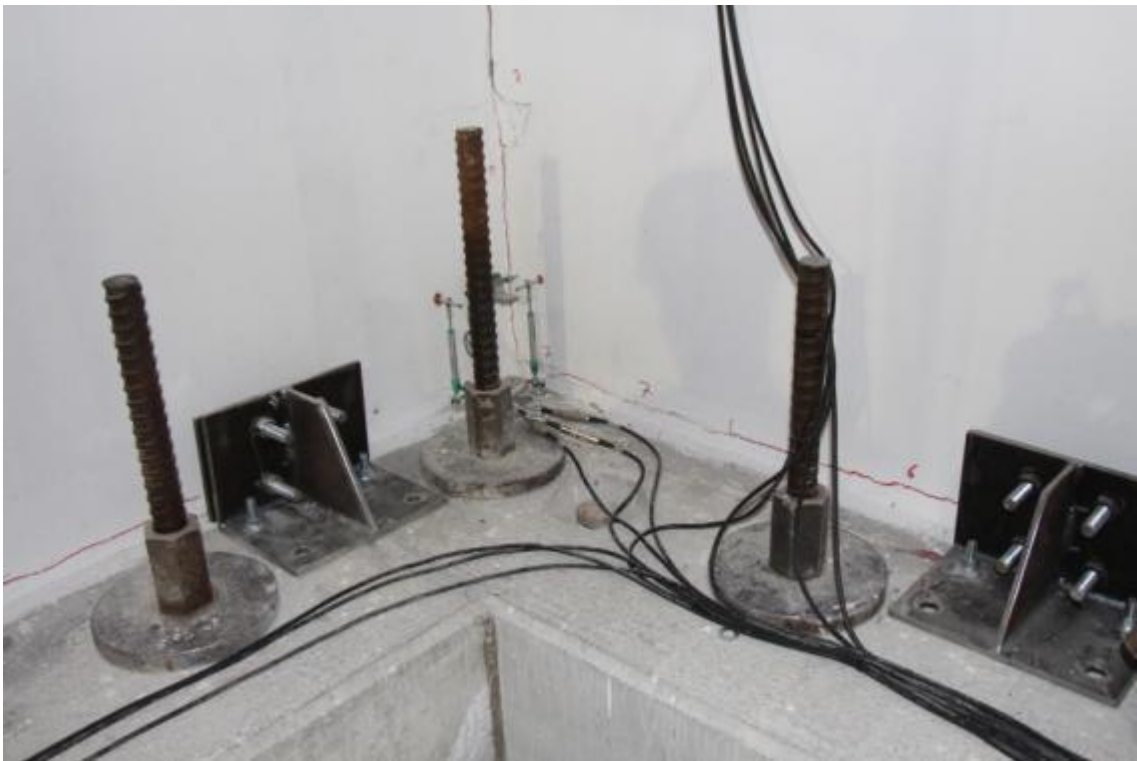
Figure 203. Damage pattern at the base of the ground-floor stability wall – East face.
