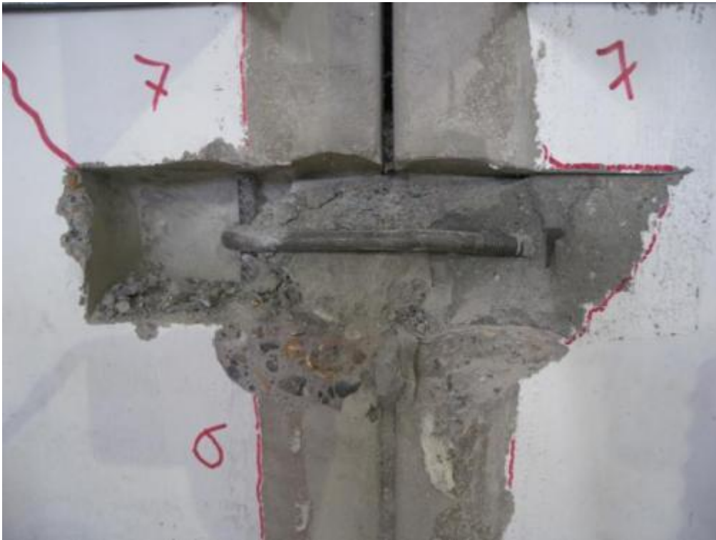
Figure 360. Detail of flexural failure mechanism of a hooked connector – Below the bottom down clip.
