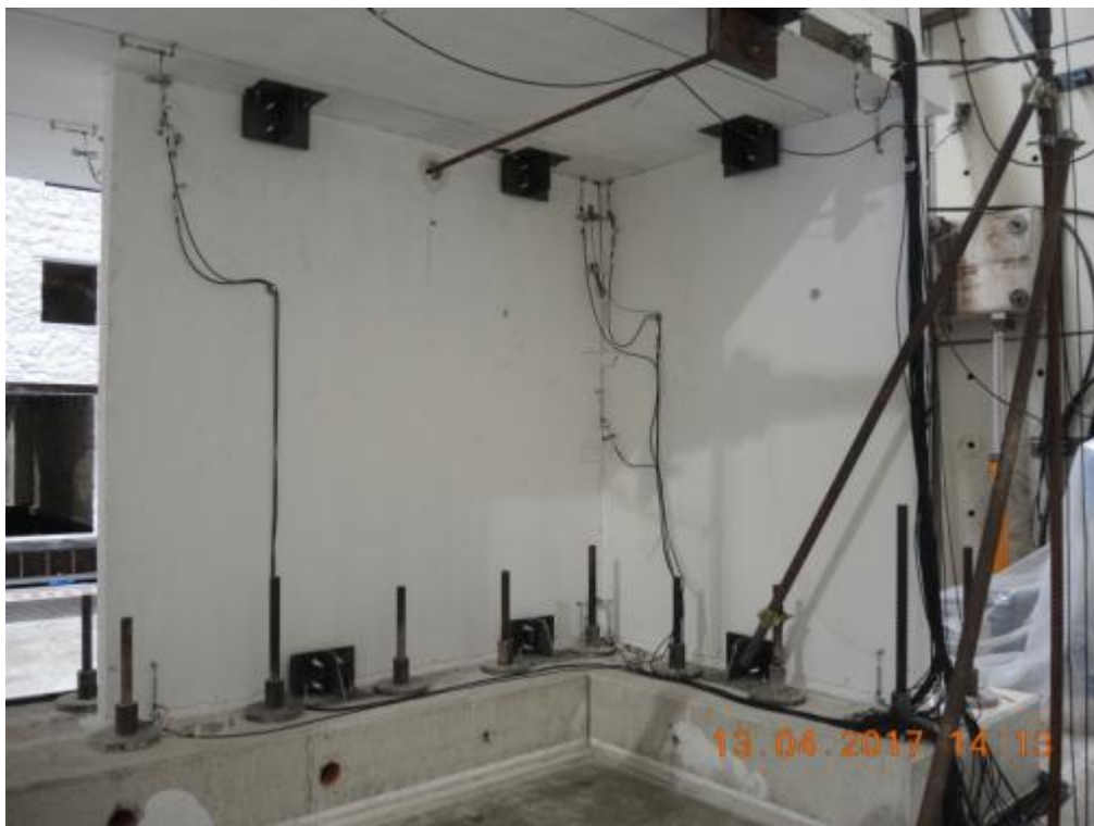
Figure 189. Three-way connection: propagation of crack along the entire wall height – Opposite side.
