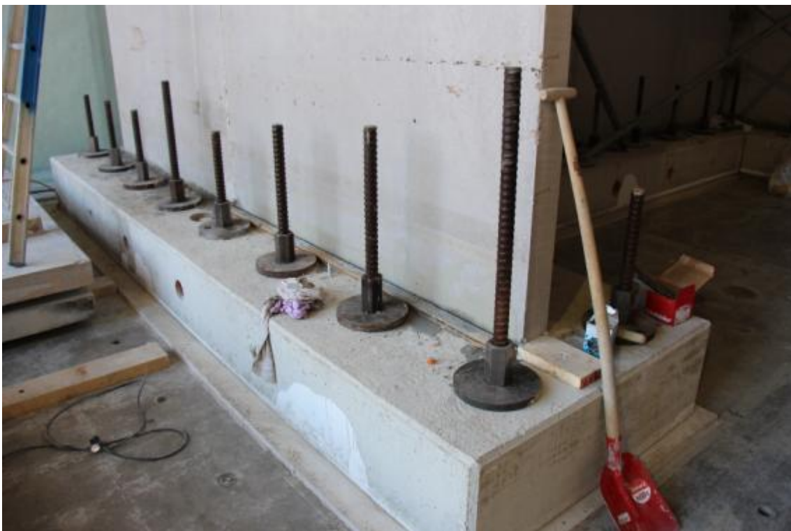
Figure 25. Execution of a mortar joint at the base of EUC-BUILD4 specimen – lateral wall.
