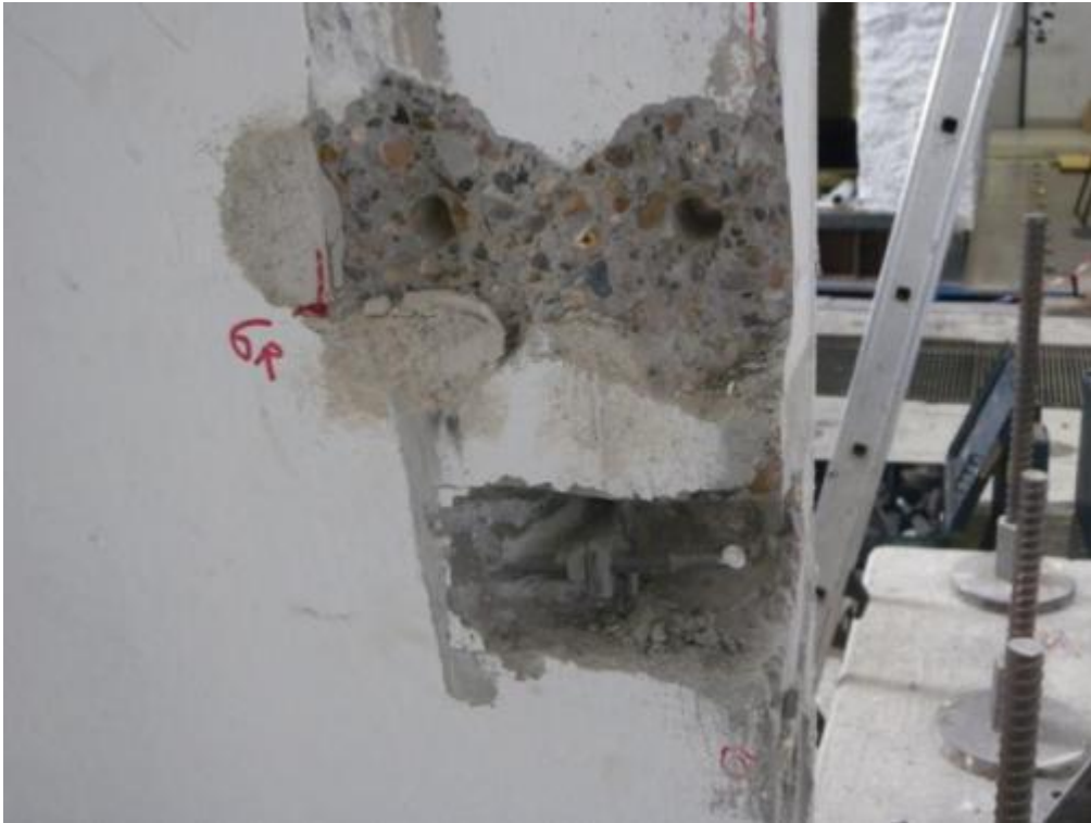
Figure 358. Ground-floor stability wall panel – Detail of cut hooked anchors and chipping of panel concrete.
