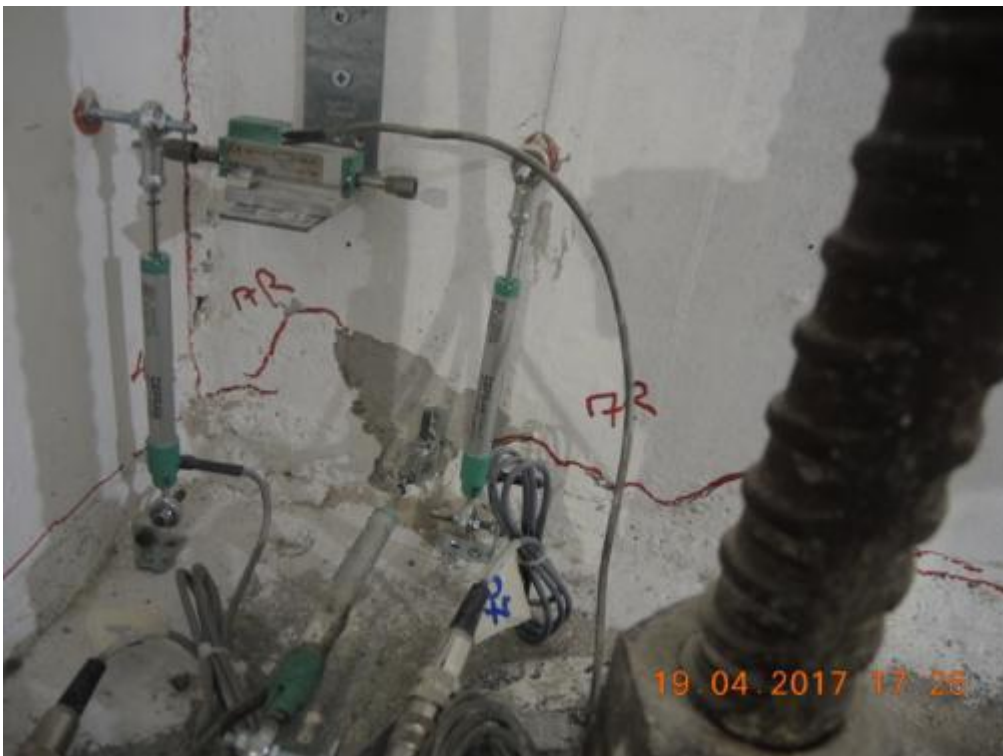
Figure 275. Damage/crack pattern at the base of the ground-floor stability wall – South side.
