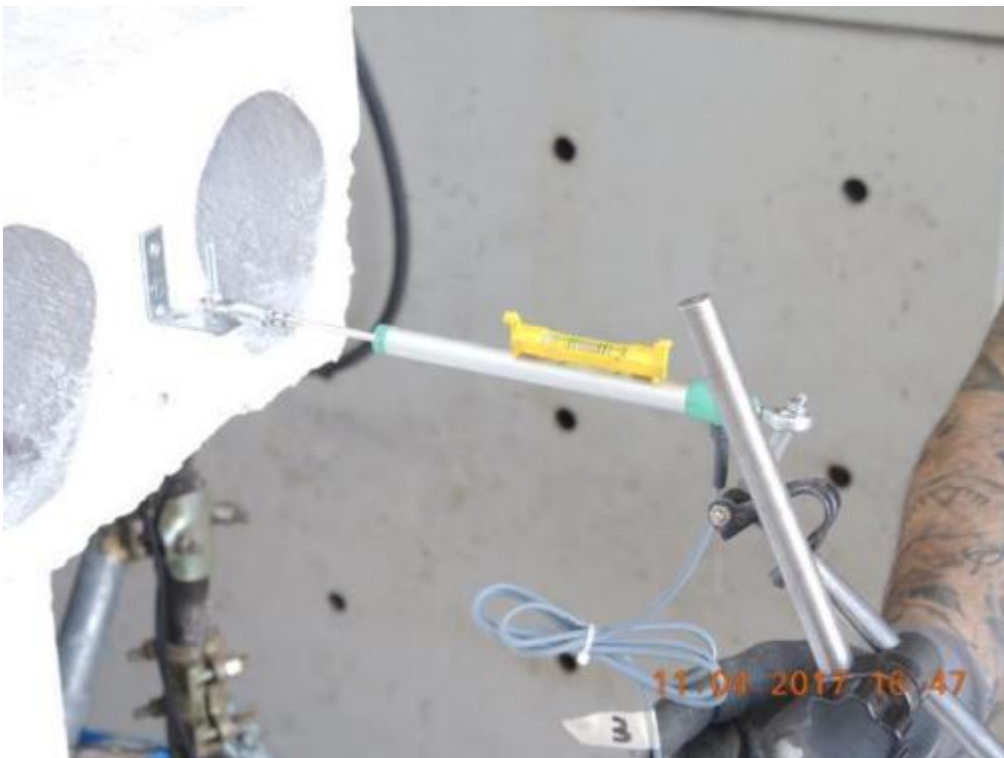
Figure 96. Detail of instrumentation for global displacement of the first storey – Lateral slab panel.
