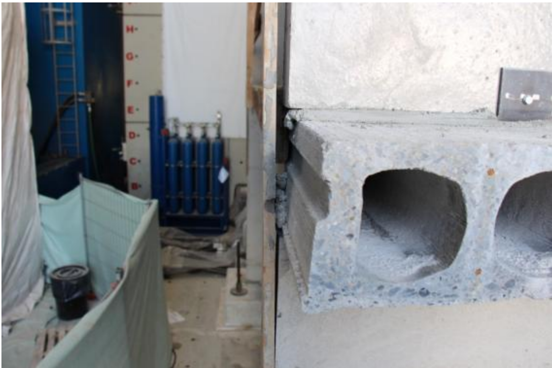
Figure 61. Detail of mortar joint at the base of the lateral wall at the second storey.
