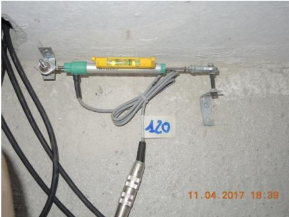
Figure 127. Potentiometer for monitoring of slab-to-stability wall sliding – Second floor slab, wall base.
