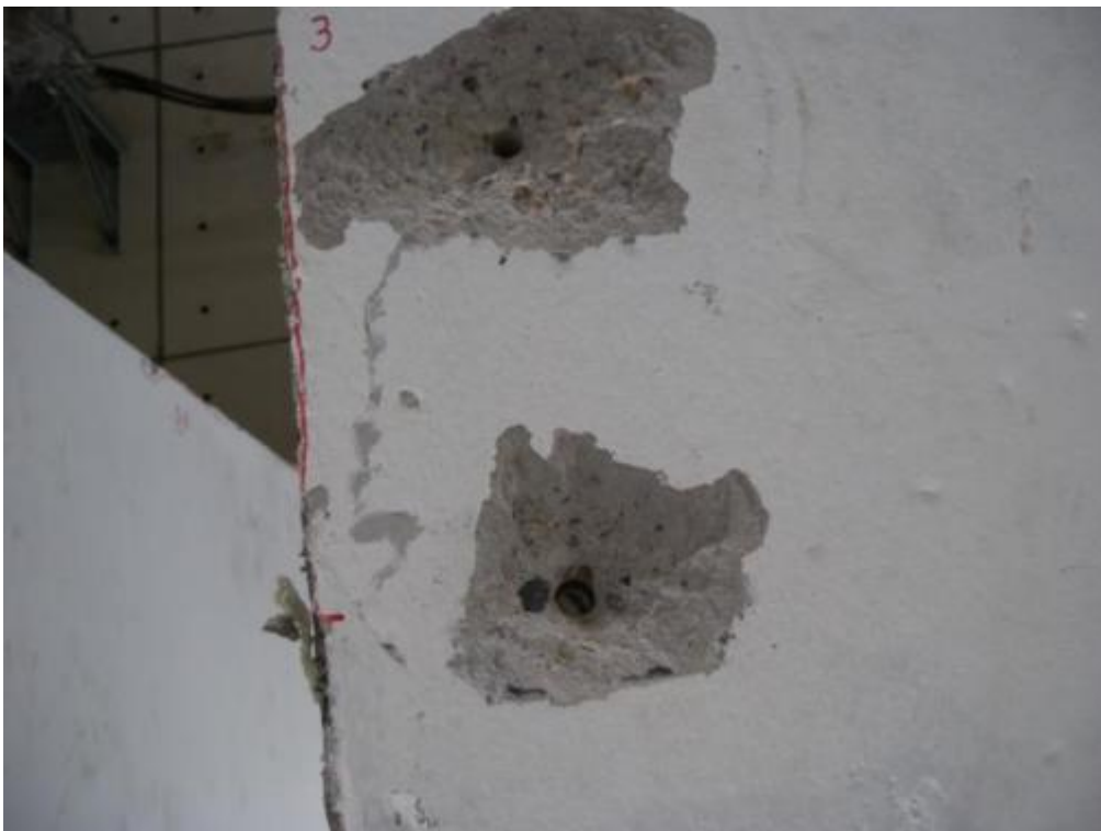
Figure 357. Detail of ground-floor stability wall panel after dismantling of steel clip angles.
