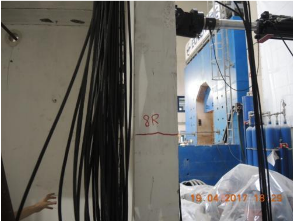
Figure 293. Side view of the full-depth/full-width/mid-height horizontal crack in lateral wall W1L2.
