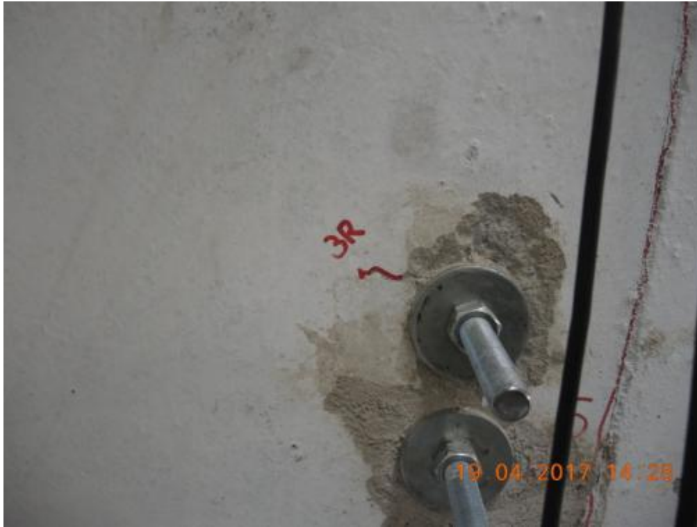
Figure 264. Crack pattern of the transversal walls (external/South face) – Opposite wall panel.
