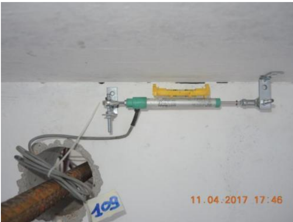
Figure 122. Instrumentation for slab-to-stability wall sliding – First floor slab, top of the wall.
