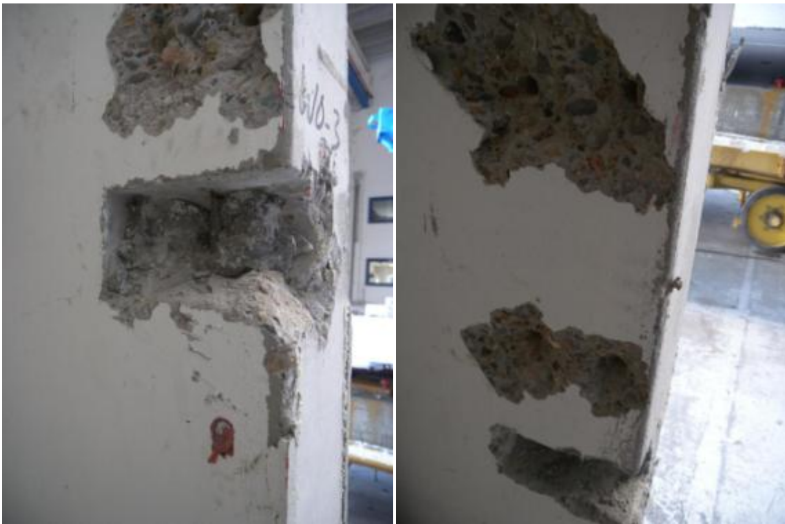
Figure 340. Detail of grout and wall panels after dismantling of steel angles – Second-storey walls.
