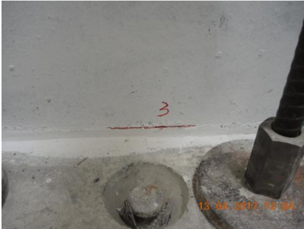
Figure 175. Development of a crack at the base of one of the transversal walls at the South side.
