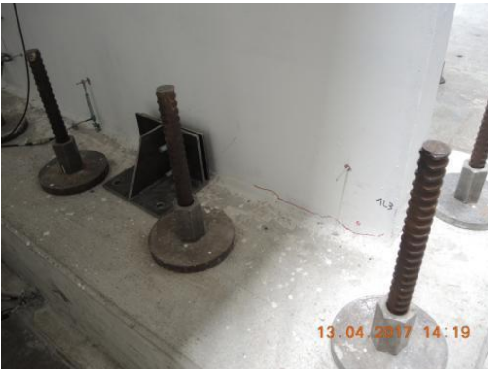
Figure 195. Horizontal cracks at the base of the transversal walls – North side, internal edge.
