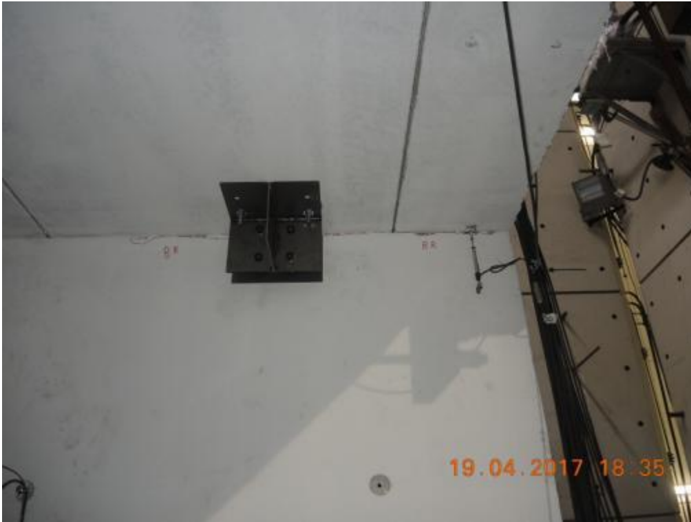
Figure 305. Concrete chipping at the top of lateral wall W1L2 – West side, first storey.
