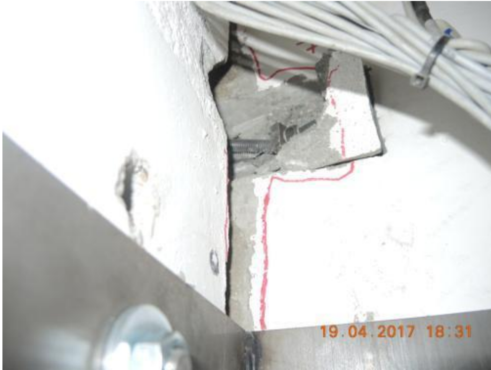
Figure 303. Enlarged view of a three-way connection and bent/failed anchor – West side, first storey.
