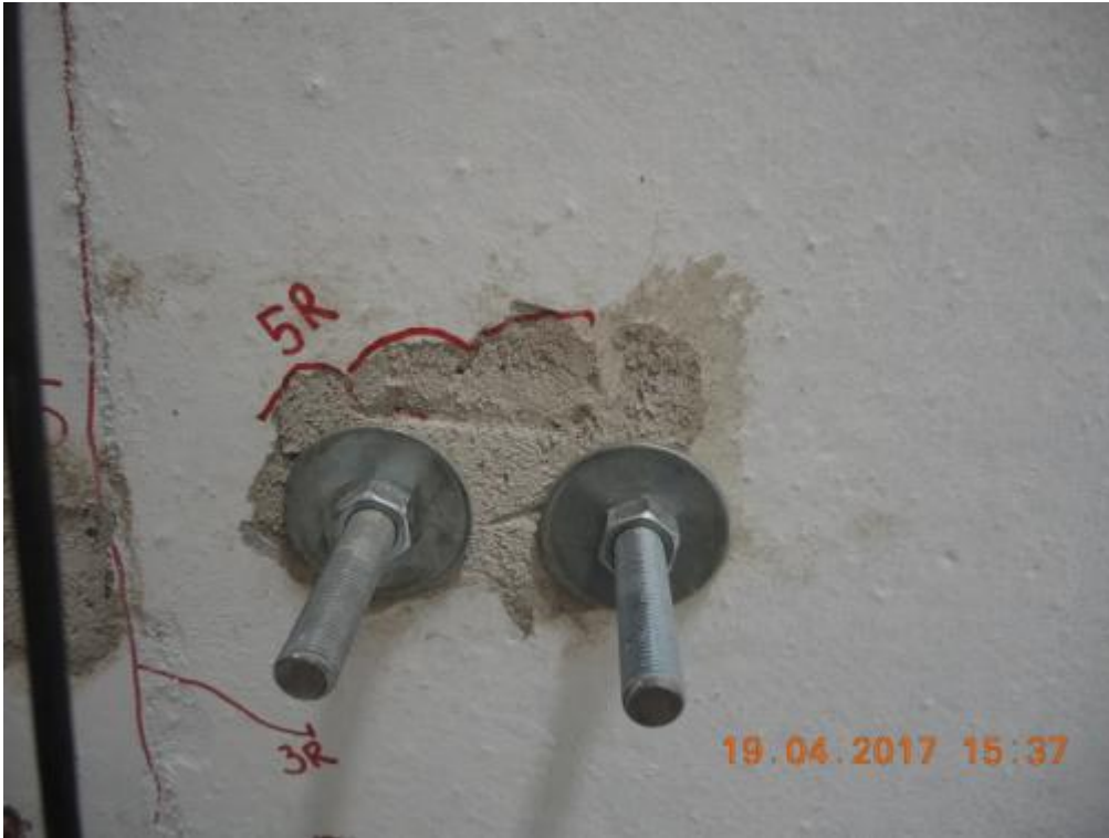
Figure 266. Development of crack pattern in correspondence to the implemented retrofitting intervention.
