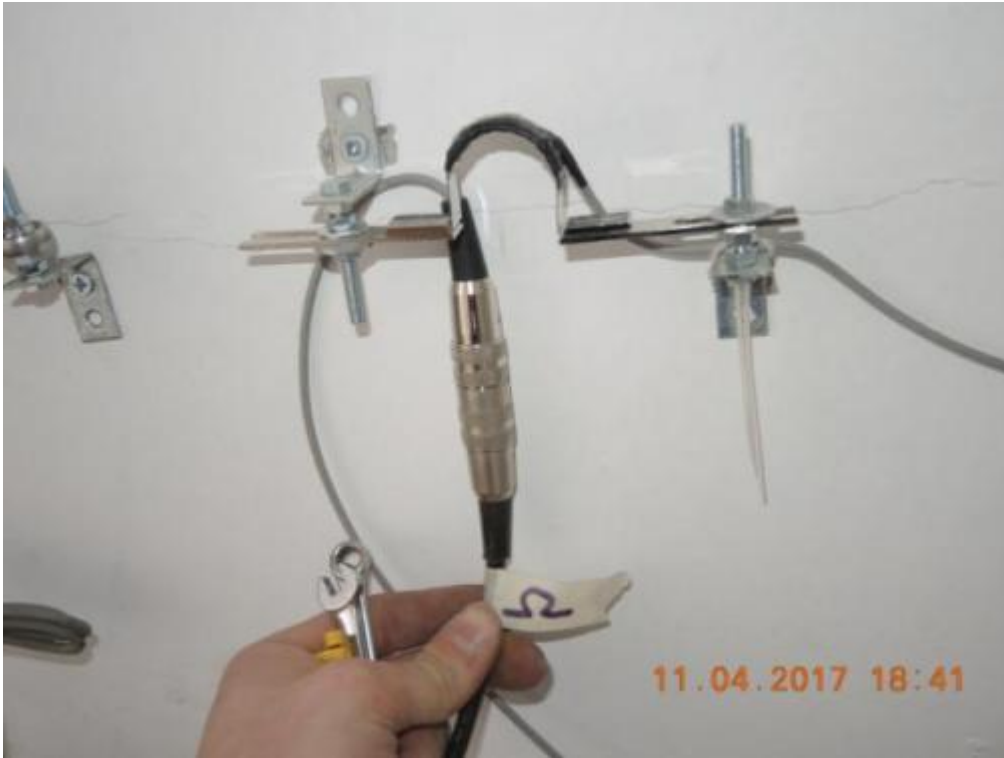
Figure 131. Detail of omega-gage instrument for monitoring of crack opening – 2 mm-stroke instrument.
