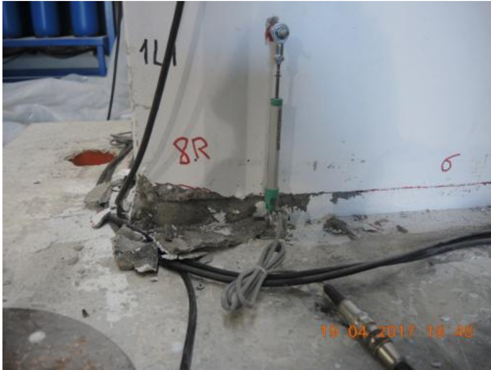
Figure 311. Transversal wall W1L1 after removal of crushed concrete – West side, North face, edge.
