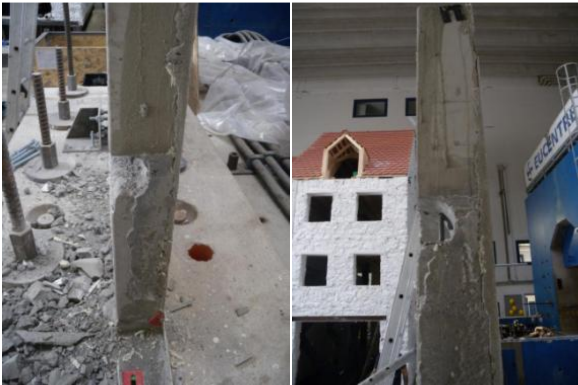
Figure 366. Detail of panel reinforcement and top/bottom niches for panel-to-panel joint – First storey.
