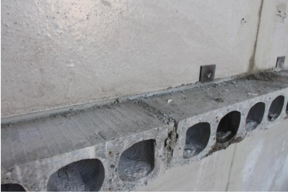
Figure 62. Detail of mortar joint and injection grout between precast hollow core slab members.
