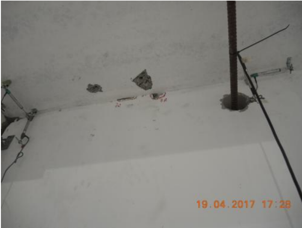
Figure 278. Minor friction-induced concrete chipping at the top of the first-storey stability wall.
