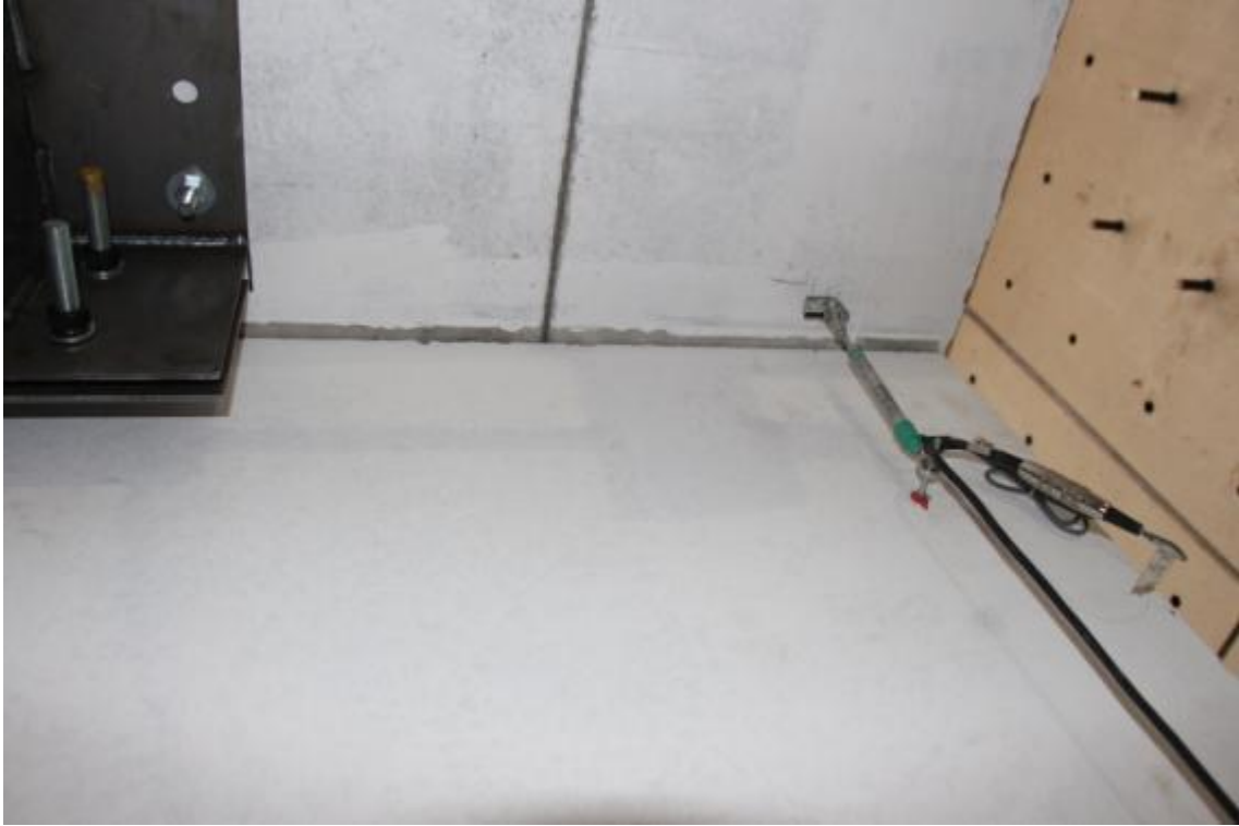
Figure 210. Accumulation of residuals due to sliding of the second-storey slabs – Bottom view.
