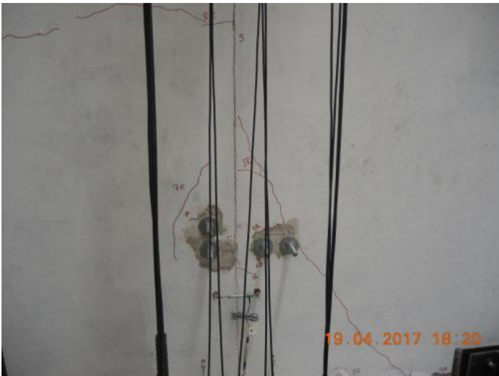
Figure 296. Crack pattern developed in the transversal wall W1L1 – West side, South face, mid-height.
