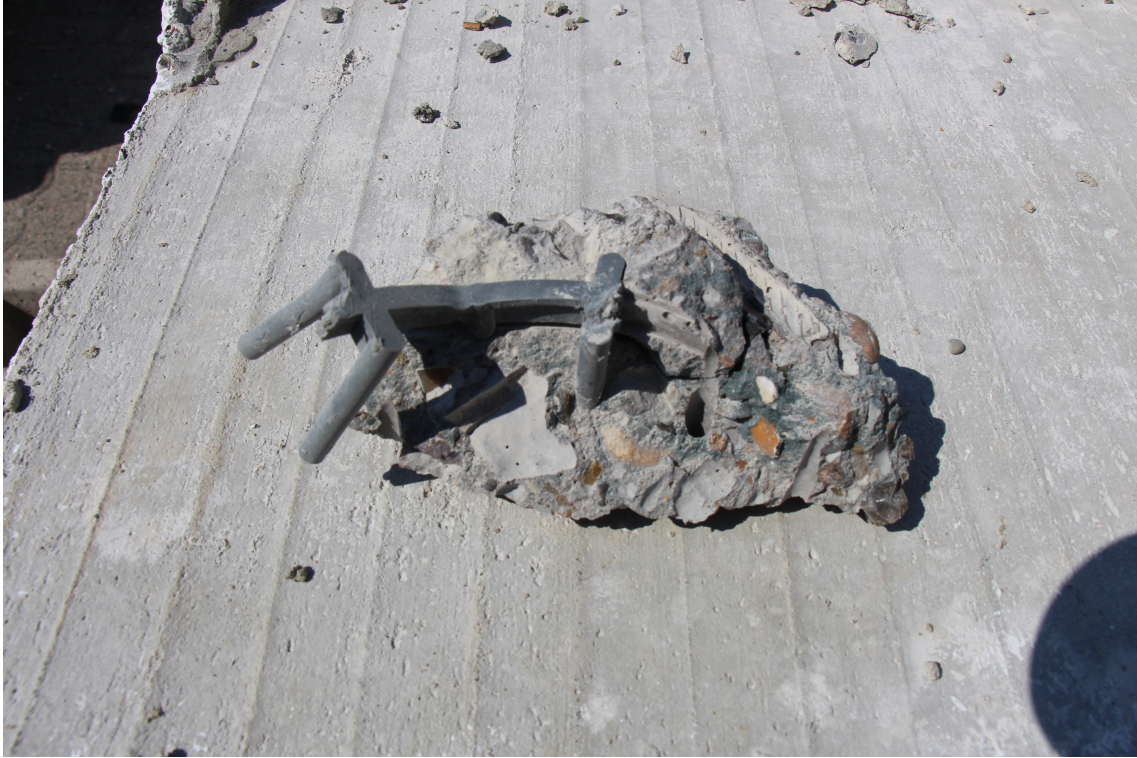
Figure 372. Detail of a 50mm spacer for the arrangement of the steel net.
