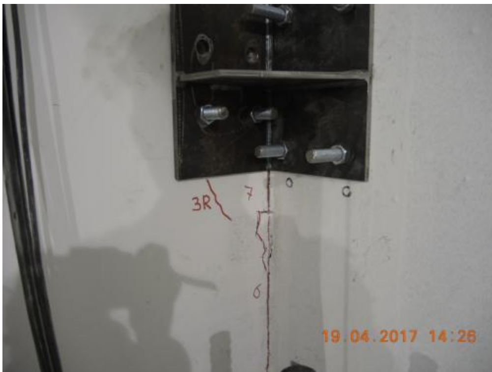
Figure 261. Development of new cracks in the transversal walls (internal face) – Below the steel angle.
