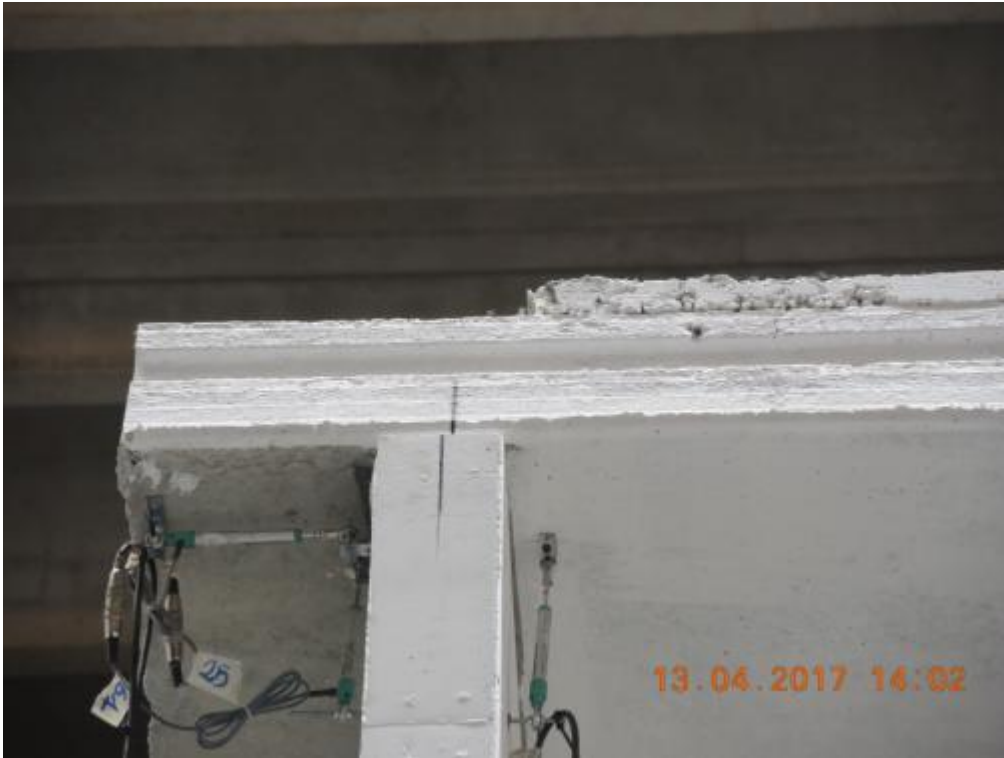
Figure 186. Detail of the second-storey floor slab after Test run #6 – accumulation of displacement residuals.
