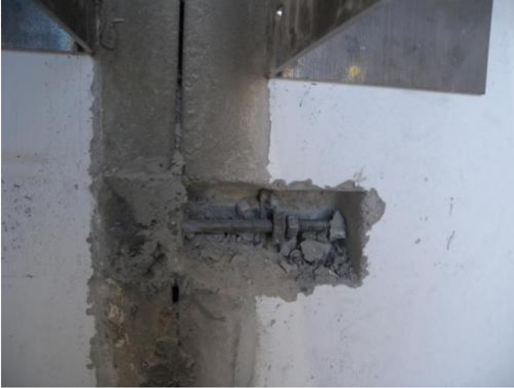
Figure 339. Enlarged view of a three-way connection after dismantling of the stability wall – Second storey.
