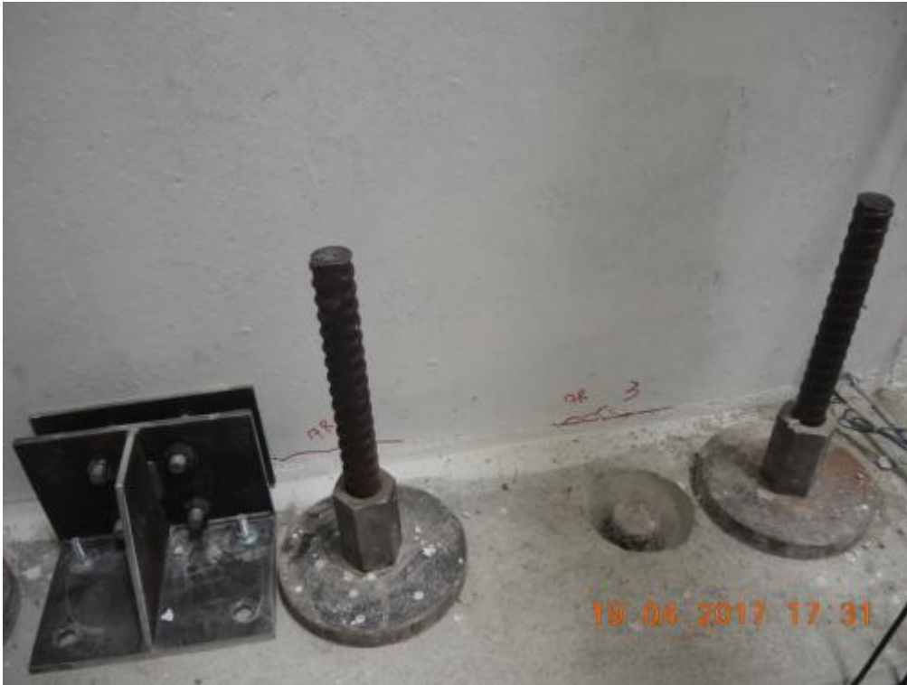
Figure 284. Crack pattern at the base of the other transversal wall – South side, first floor.
