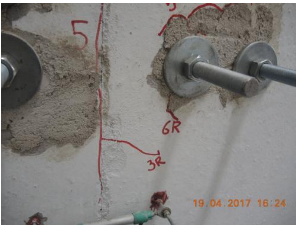
Figure 270. Evolution of crack pattern in correspondence to the implemented retrofitting intervention – Bottom.
