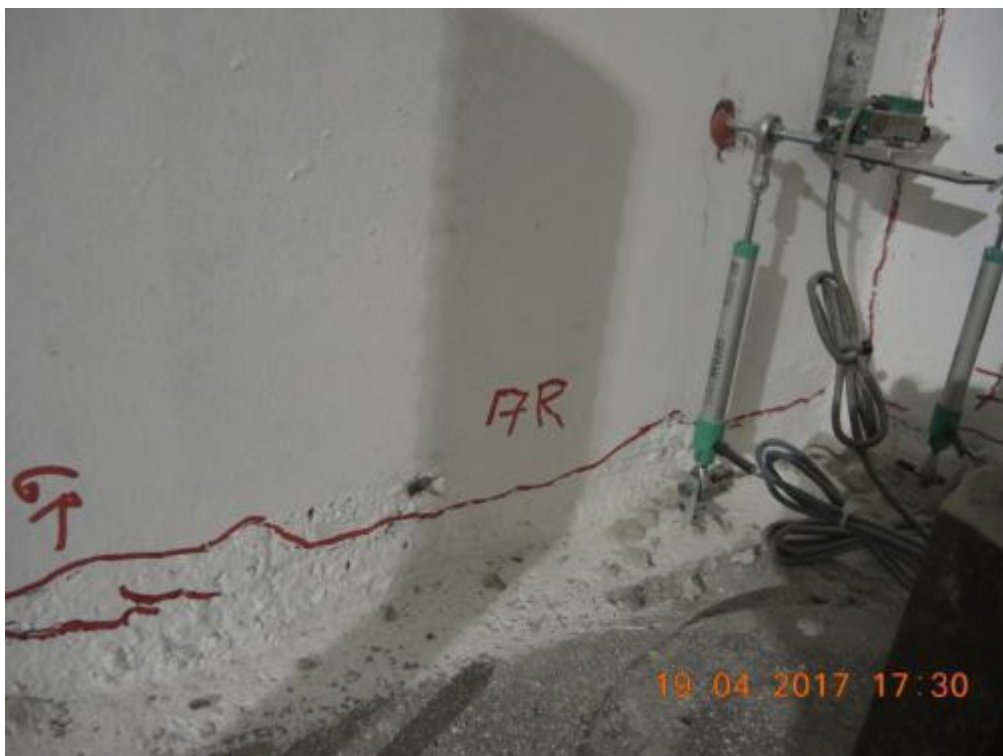
Figure 281. Crack pattern at the base of the ground-floor stability wall – West side, opposite edge.
