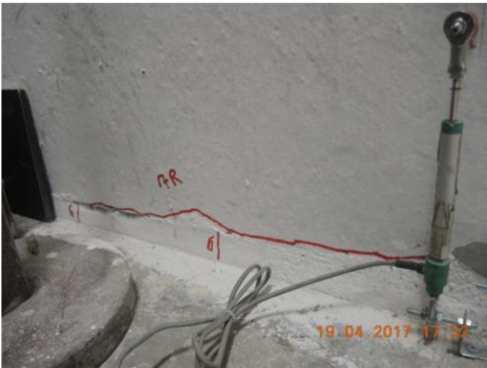
Figure 283. Crack pattern at the base of one of the transversal wall – South side, first floor.
