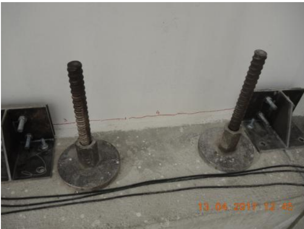
Figure 177. Propagation of horizontal cracks along the depth of the ground-floor stability wall – Opposite side.
