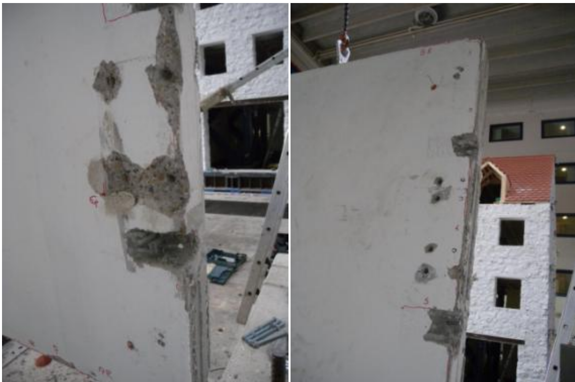
Figure 359. Damage pattern of the first-floor stability wall after dismantling of connections and setup.
