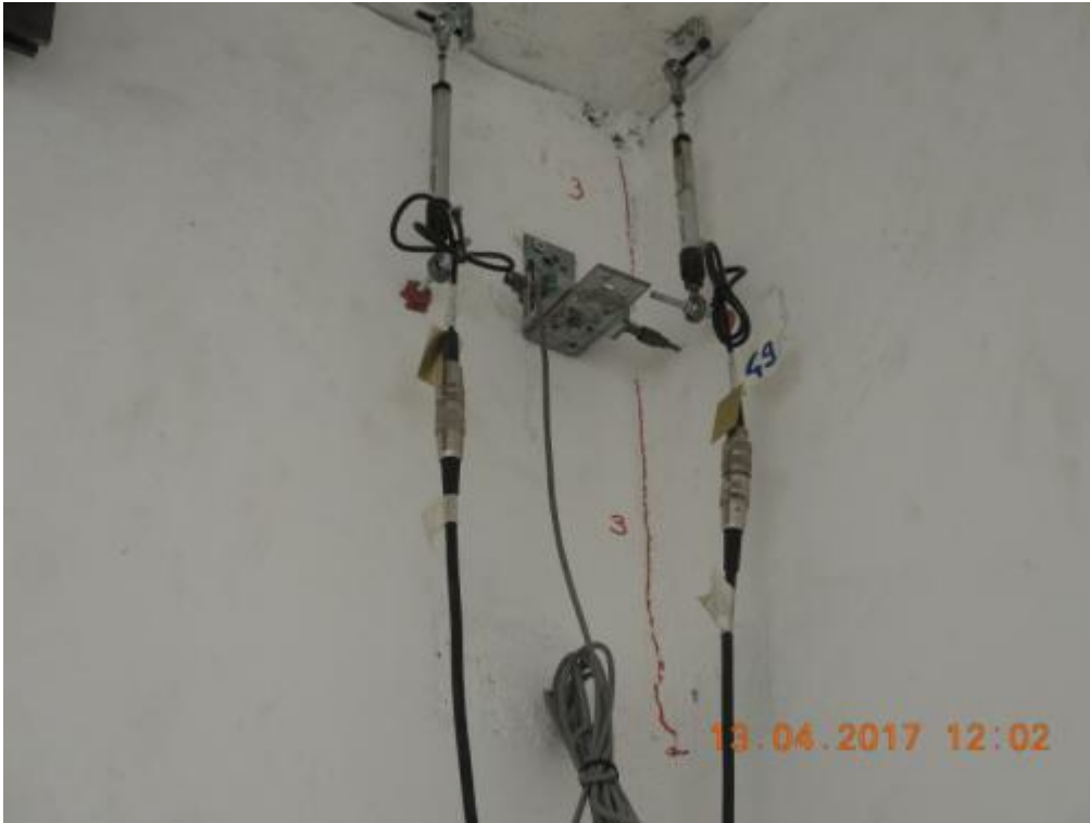
Figure 173. Crack opening in correspondence to the connection between stability and lateral walls – Top.
