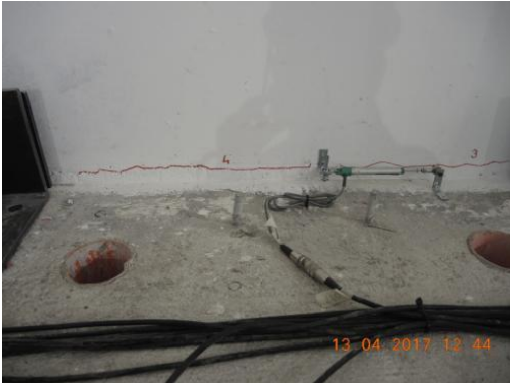
Figure 176. Propagation of horizontal cracks along the depth of the ground-floor stability wall – Wall base.
