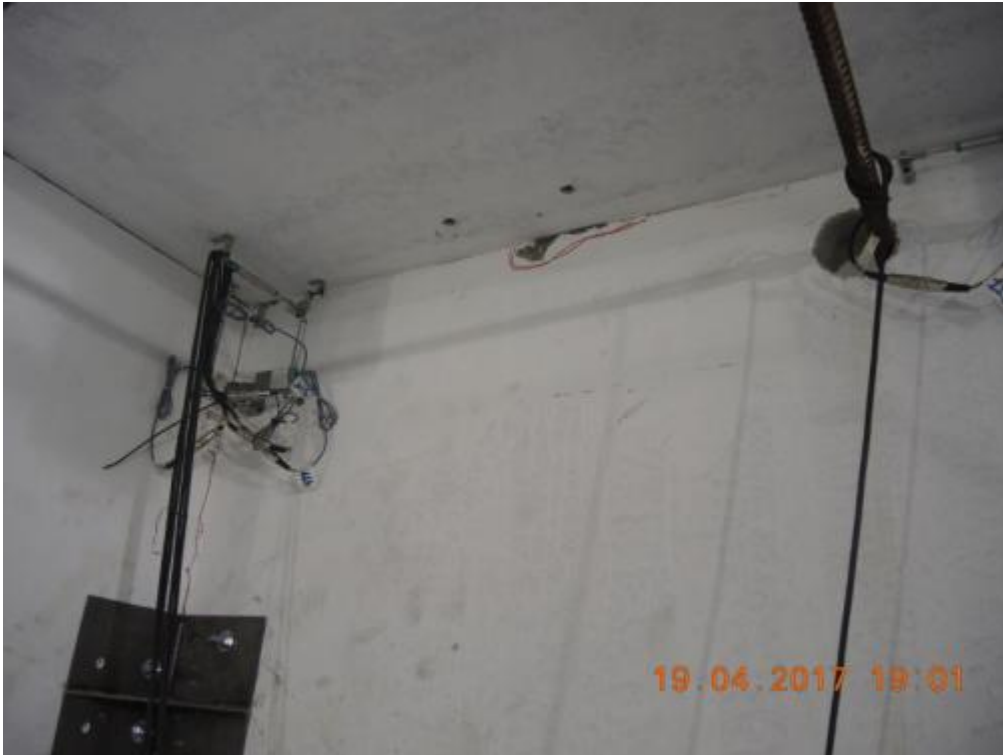
Figure 315. Chipping of concrete at the top of the second-storey stability wall – East side.
