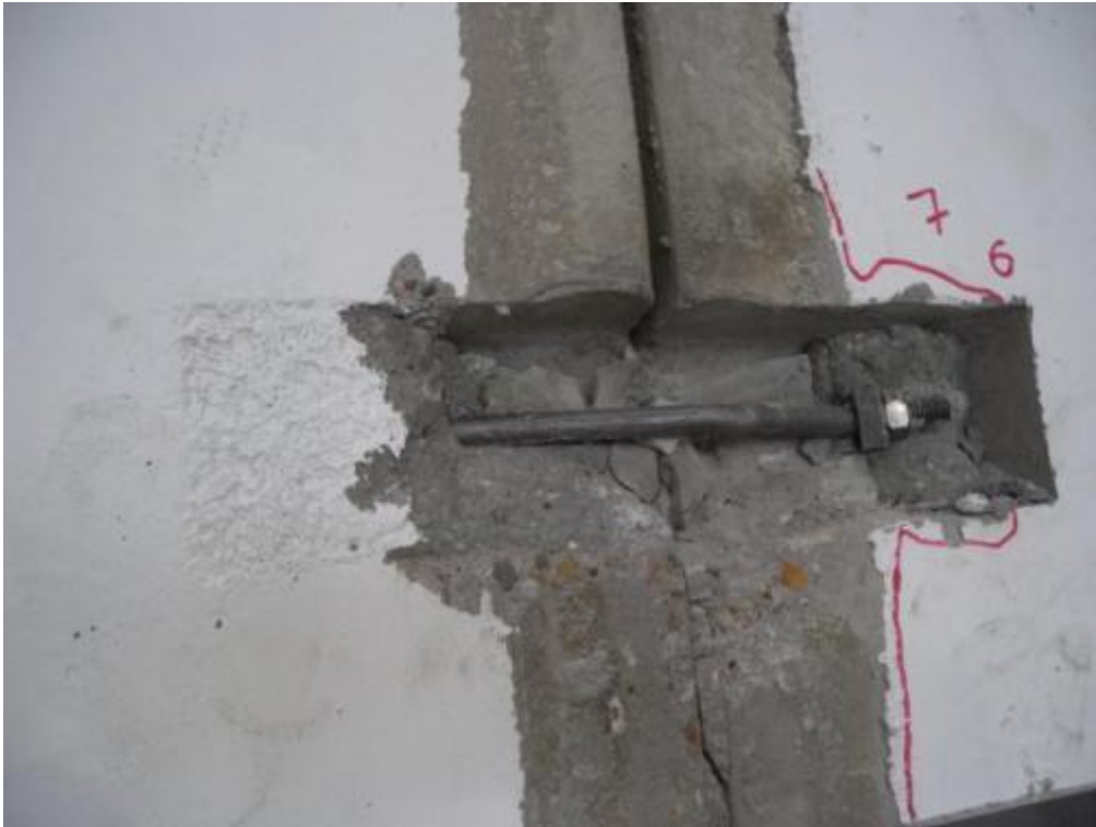
Figure 363. Detail of flexural failure mechanism of a hooked connector – Above the top clip.
