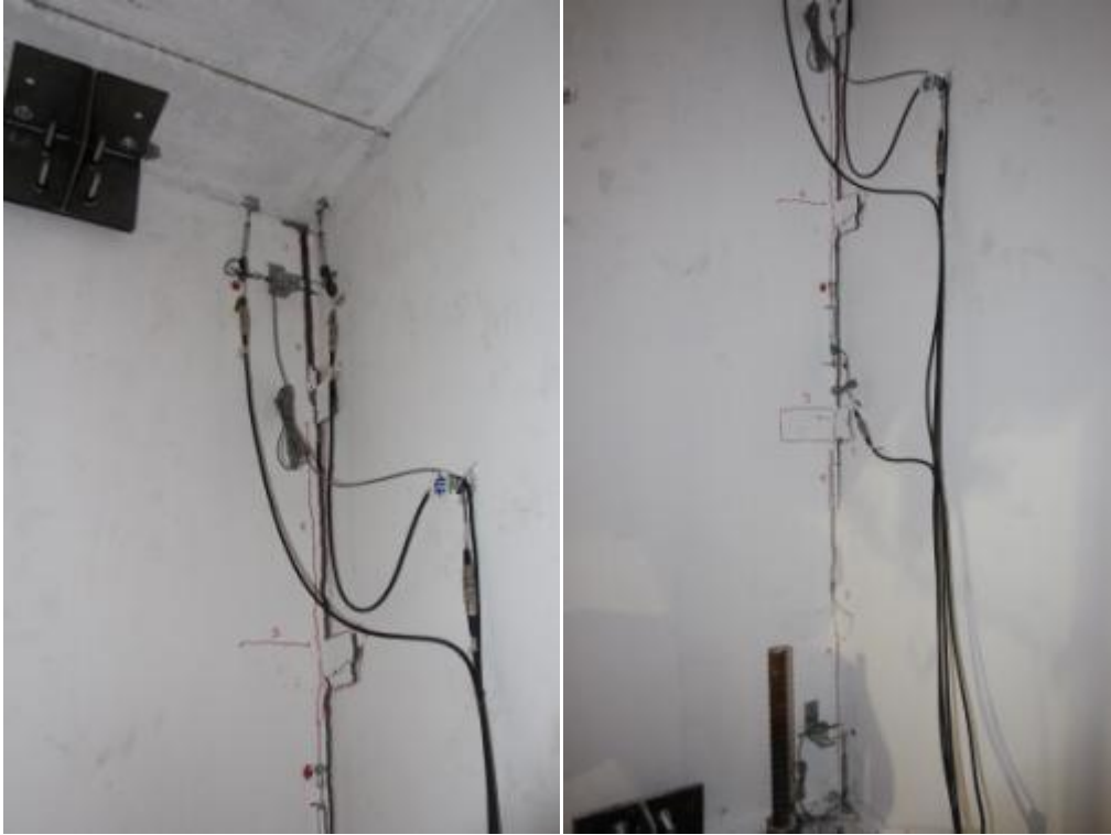
Figure 204. Gap opening between the stability and lateral walls – Top and mid-height, opposite side.
