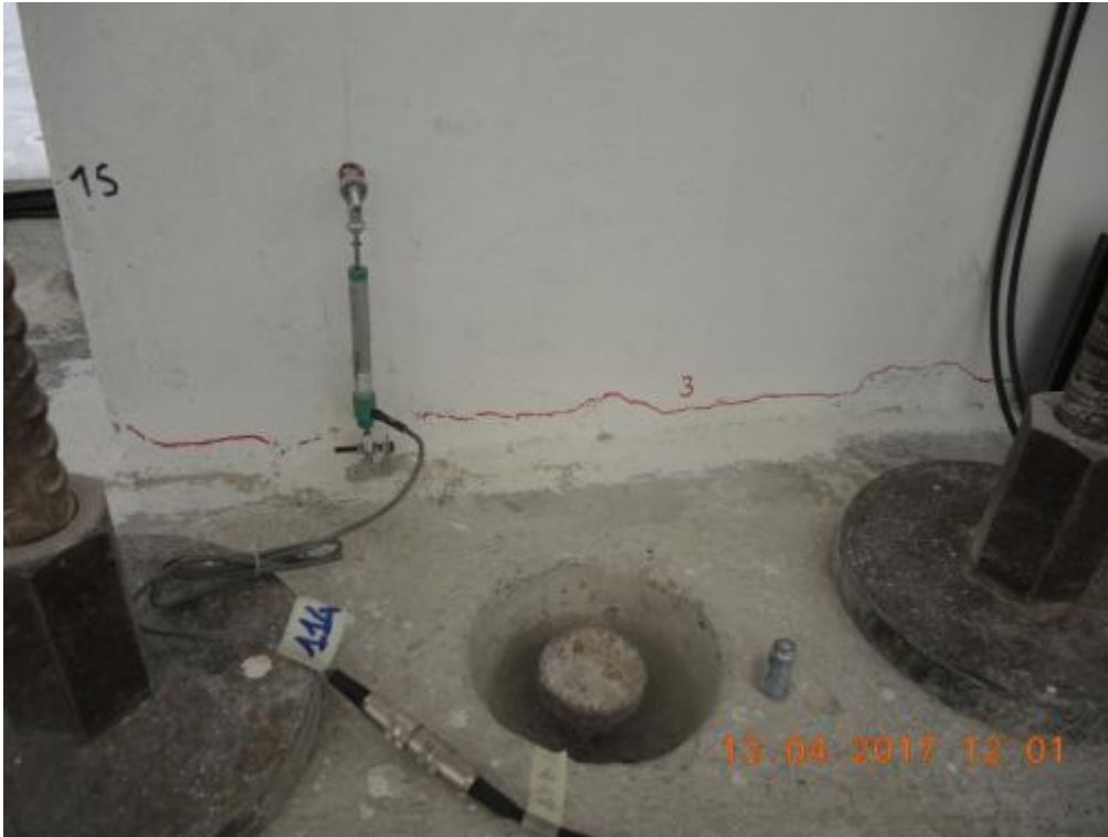
Figure 171. Crack pattern at the base of the first-floor stability wall – Edge of the wall.
