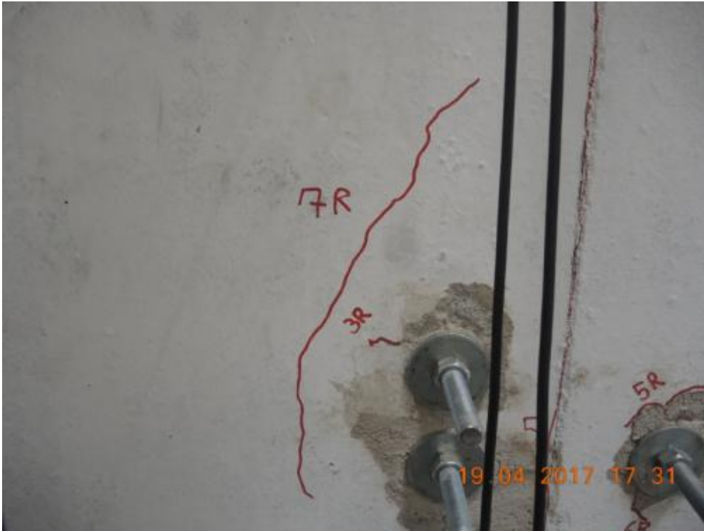
Figure 282. Formation of a new crack in one of the lateral walls close to steel angles and bolted rods.
