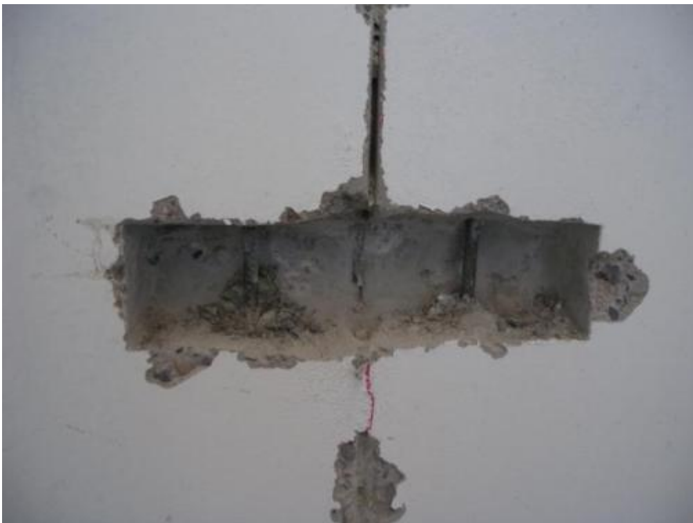
Figure 347. Panel reinforcement after removal of the hooked anchor – Lateral walls, first storey.
