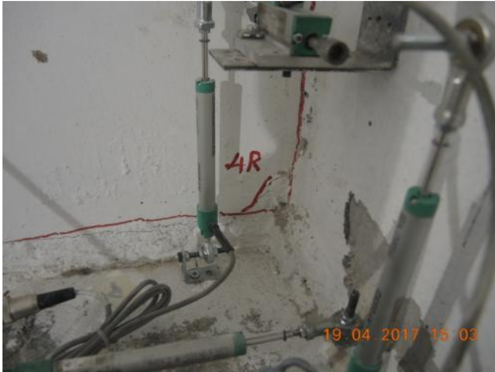
Figure 265. Formation of new minor cracks at the base of the transversal walls – South side.
