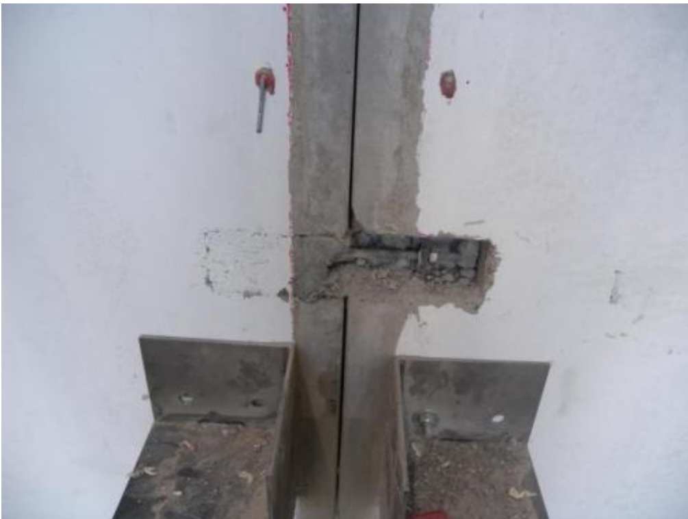
Figure 338. Detail of anchors and grout in a three-way connection after dismantling of the stability wall.
