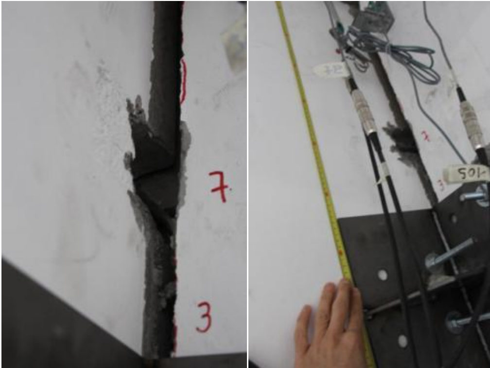
Figure 216. EUC-BUILD4 “retrofitted” specimen – Detail of the gap between stability and lateral walls.
