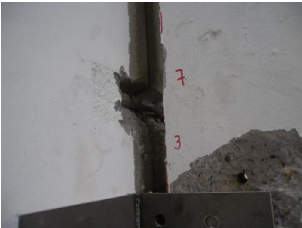
Figure 353. Removal of screwed clip angles and detail of failed connector – First storey, South side.
