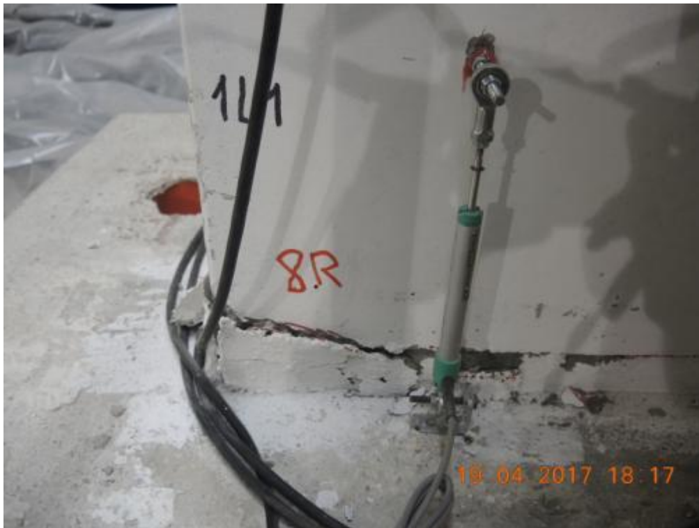
Figure 289. Detail of concrete crushing at the base of lateral wall W1L1 – East side.
