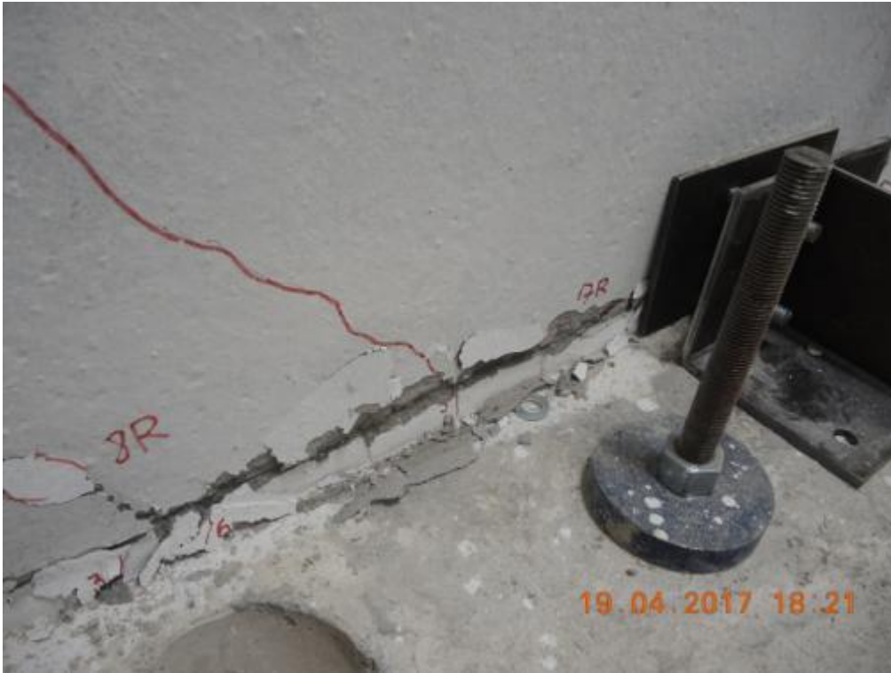
Figure 299. Detail of concrete crushing at the base of transversal wall W1L1 – West side, South face.
