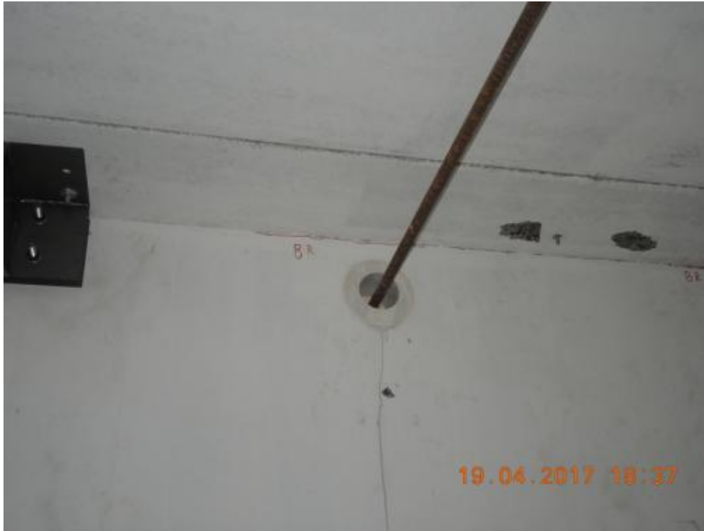
Figure 307. Concrete chipping at the top of the ground-floor stability wall – West side, mid-depth.
