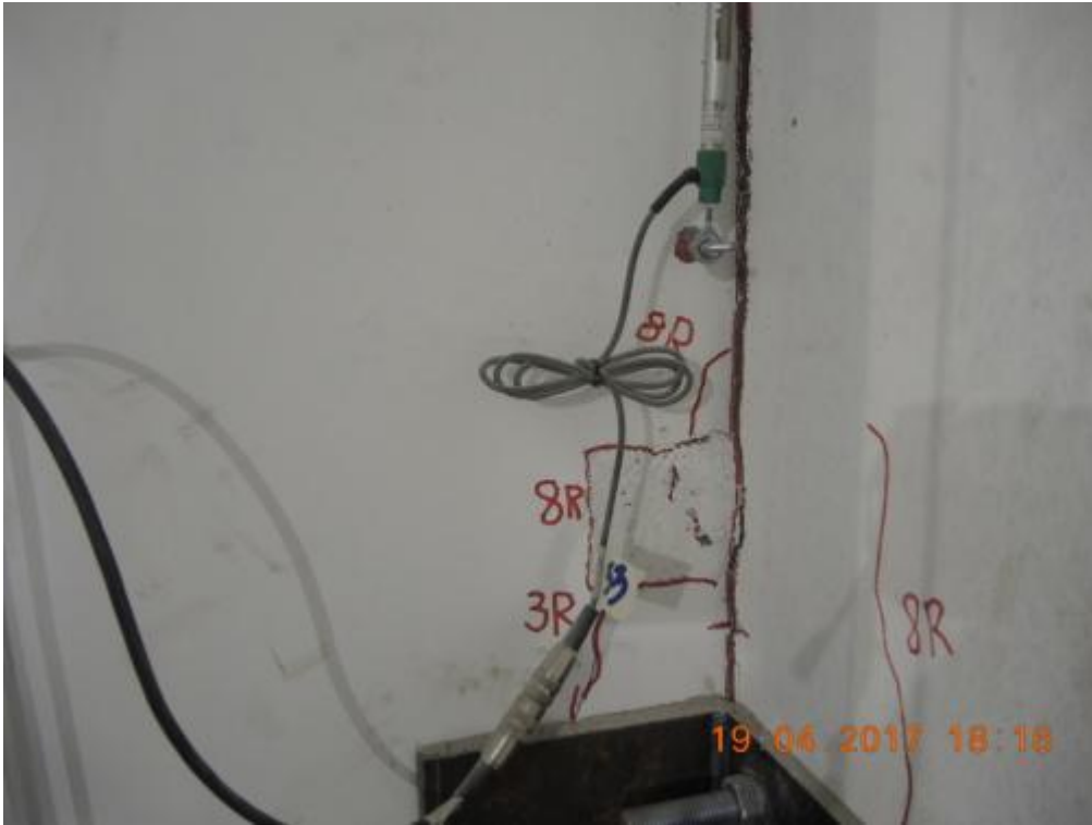
Figure 287. Detail of cracks in the transversal and stability walls – Bottom steel angle, East side.
