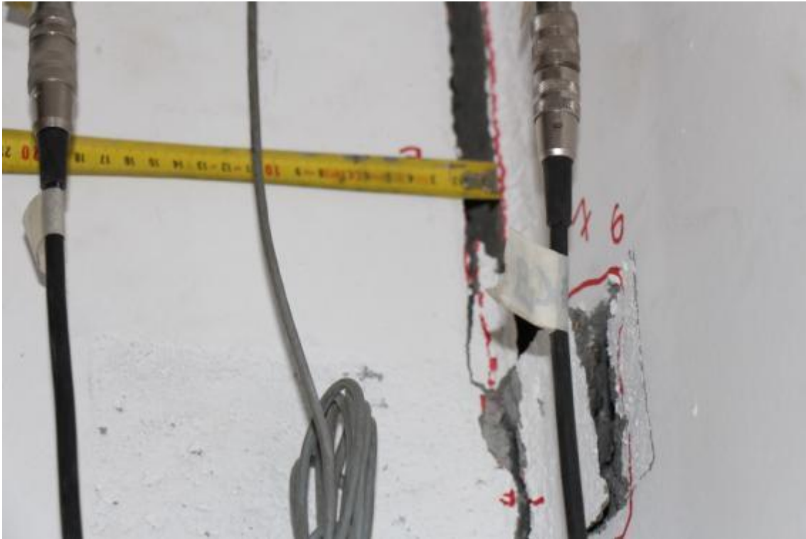
Figure 206. Detail of gap opening between the stability and lateral walls – Top, West side.
