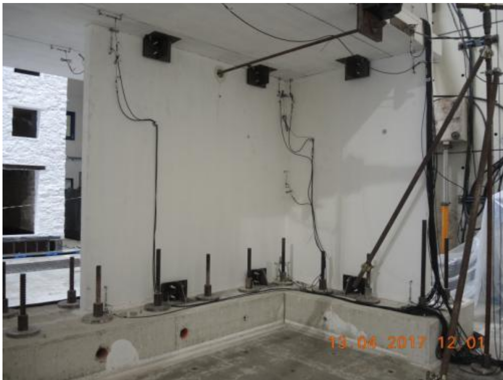
Figure 170. Development of cracks in the ground-floor stability wall.
