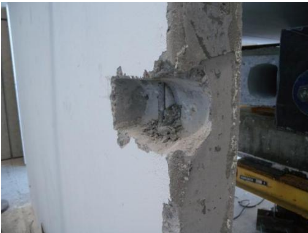
Figure 349. Detail of longitudinal rebar in one of the transversal walls – First storey, North side.
