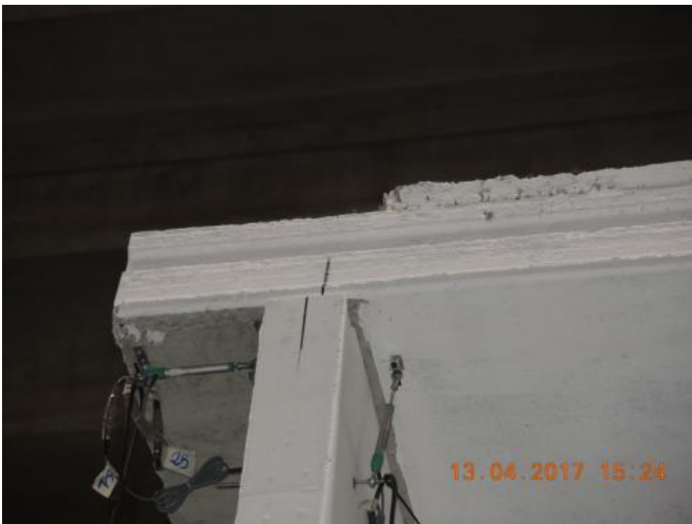
Figure 199. Accumulation of displacement residuals due to sliding – Detail of the second-storey floor slab.
