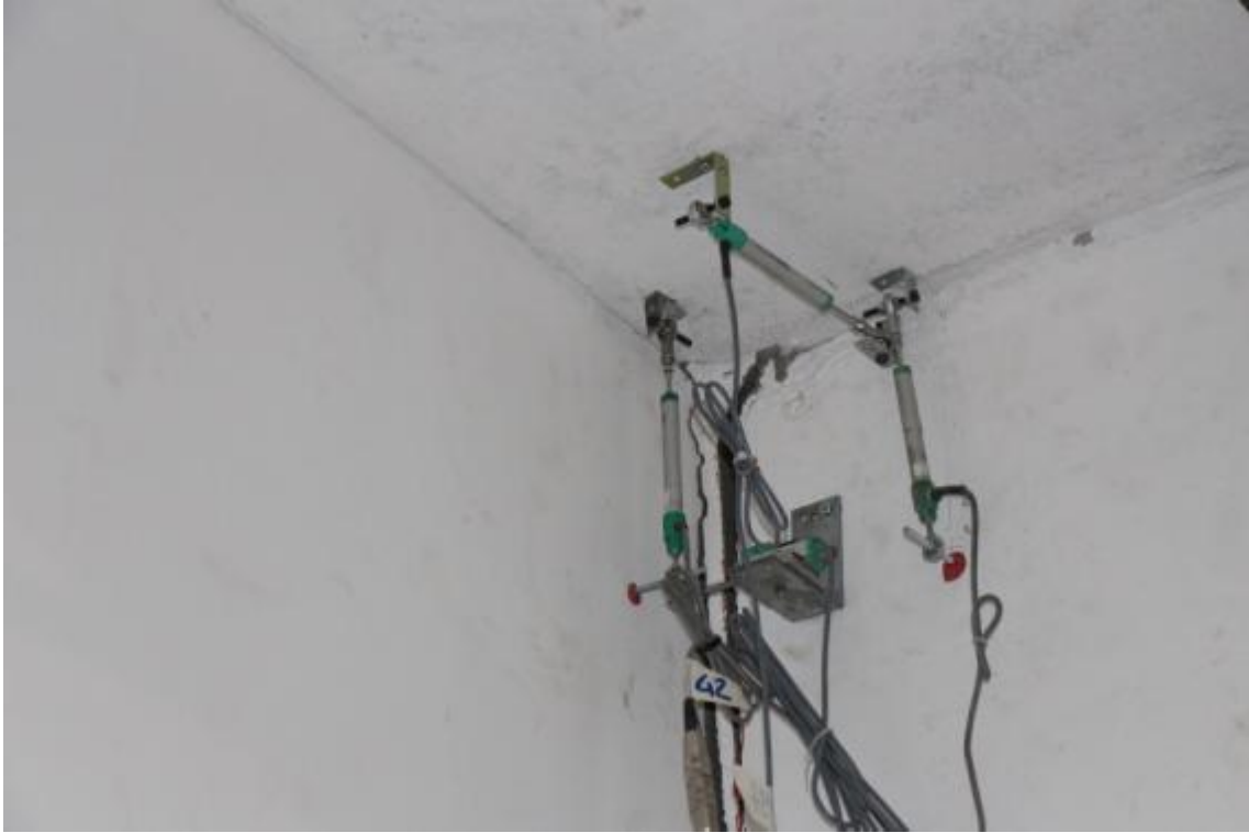
Figure 202. Detail of the complete gap opening between the stability and lateral walls – Top.
