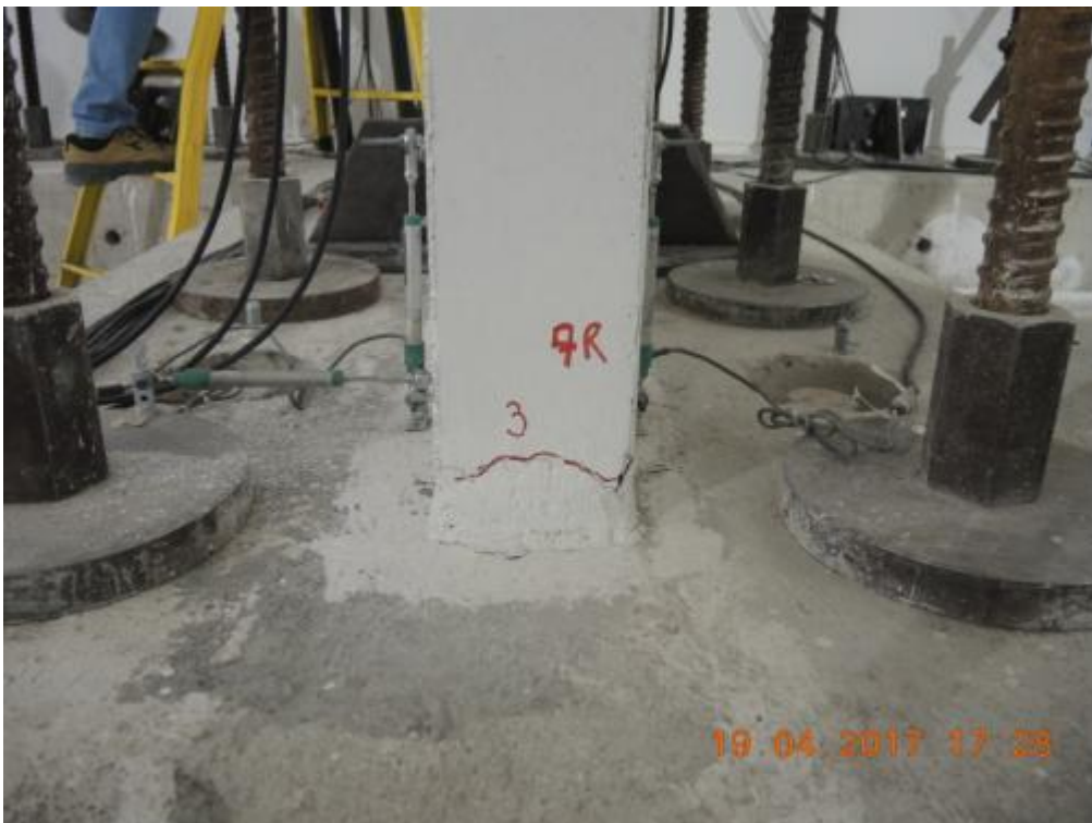
Figure 277. Damage/crack pattern at the base of the ground-floor stability wall – North side, North face.
