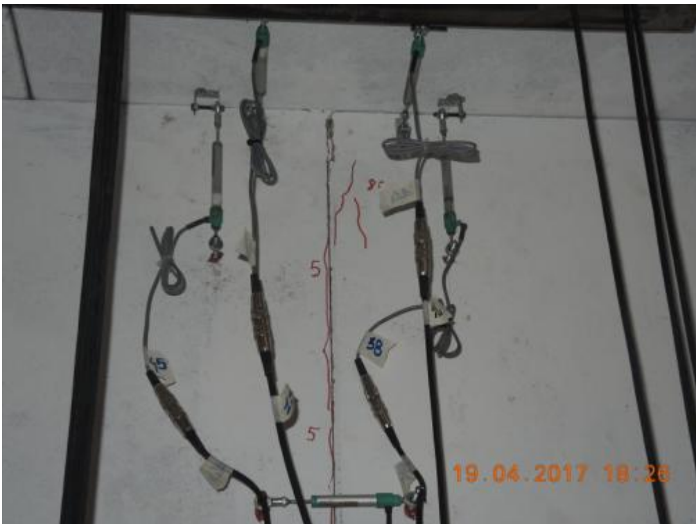
Figure 300. Formation and propagation of new cracks at the top of lateral wall W1L1 – West side, South face.
