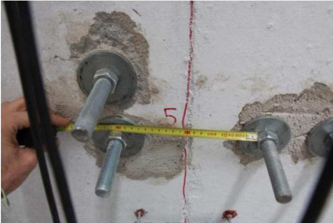
Figure 218. EUC-BUILD4 “retrofitted” specimen – Detail of bolts and washers, South lateral walls.
