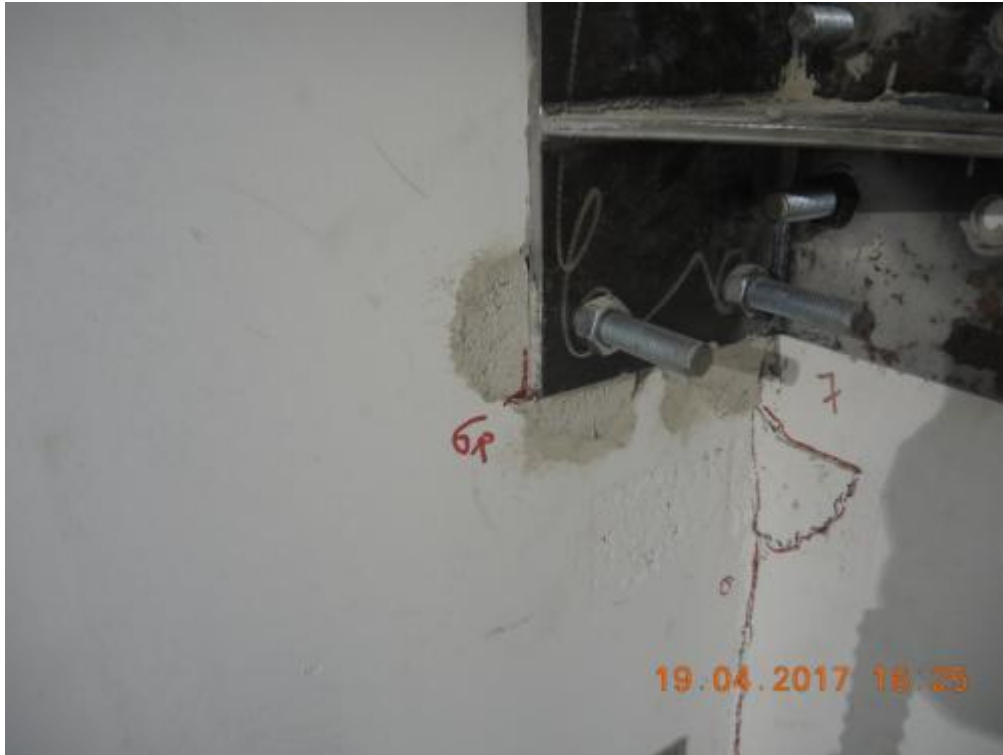
Figure 273. Crack pattern in correspondence to the bottom steel angle – Opposite/West side.
