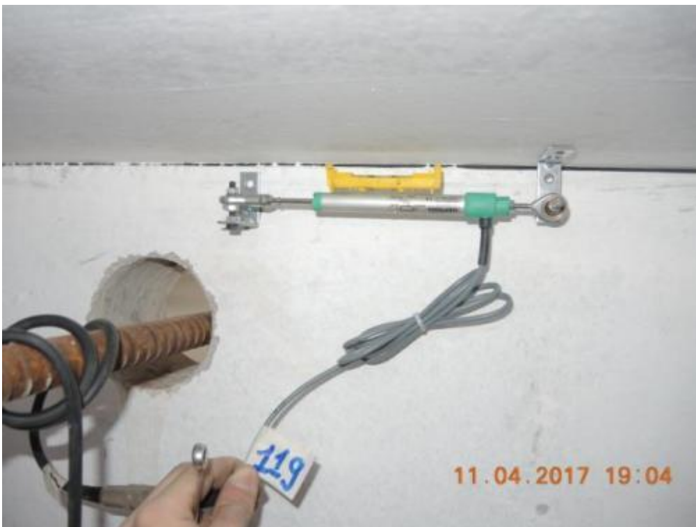
Figure 126. Instrumentation for slab-to-stability wall sliding – Second floor slab, top of the wall.
