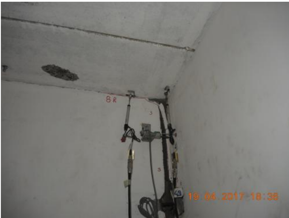
Figure 306. Concrete chipping at the top of the ground-floor stability wall – West side, edge.
