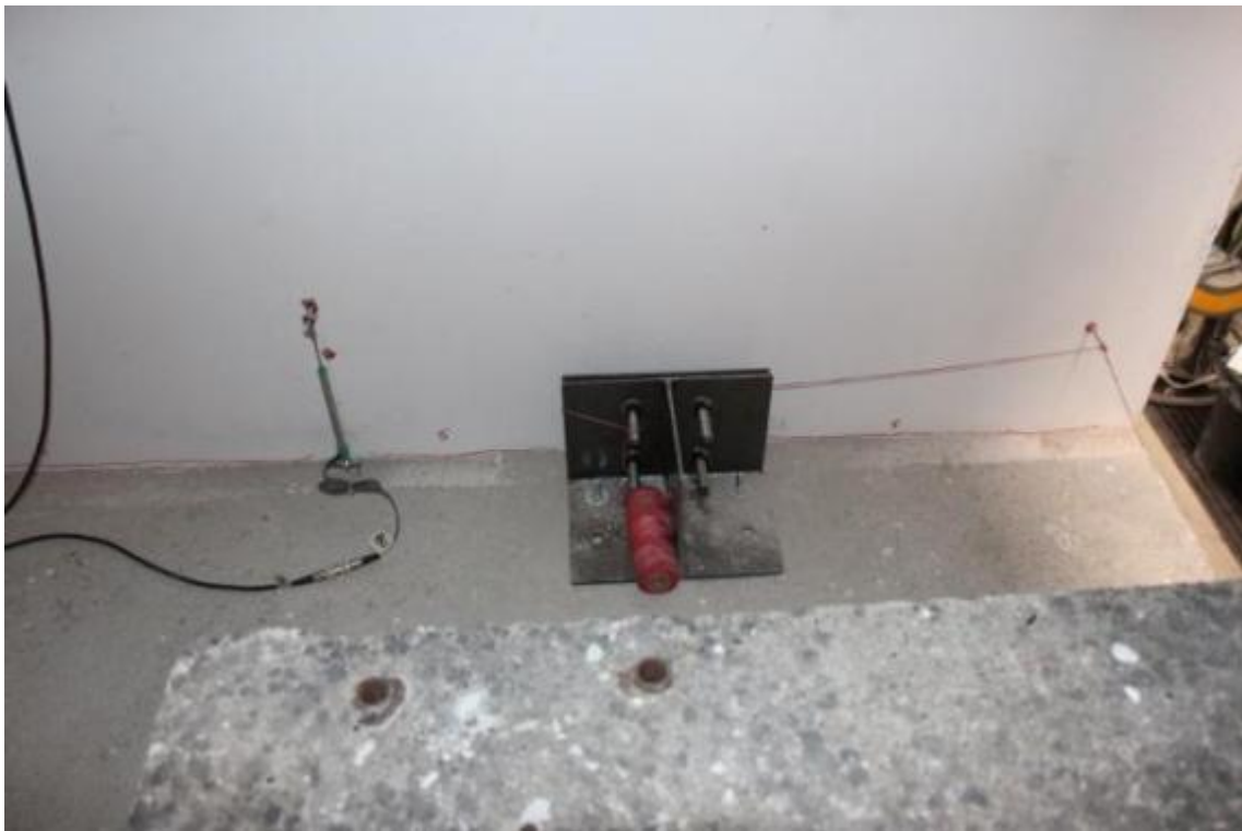
Figure 197. Crack pattern at the base of the second-storey transversal walls – North side, internal face.
