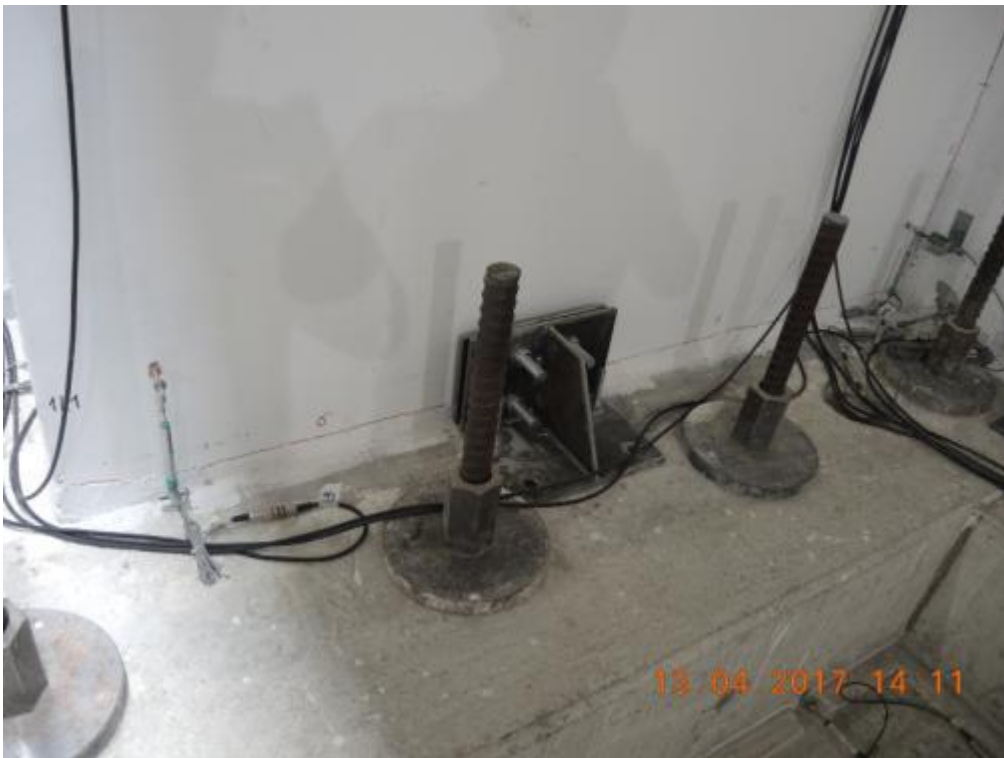
Figure 187. Crack pattern at the base of lateral wall W1L1 – South side, internal edge.
