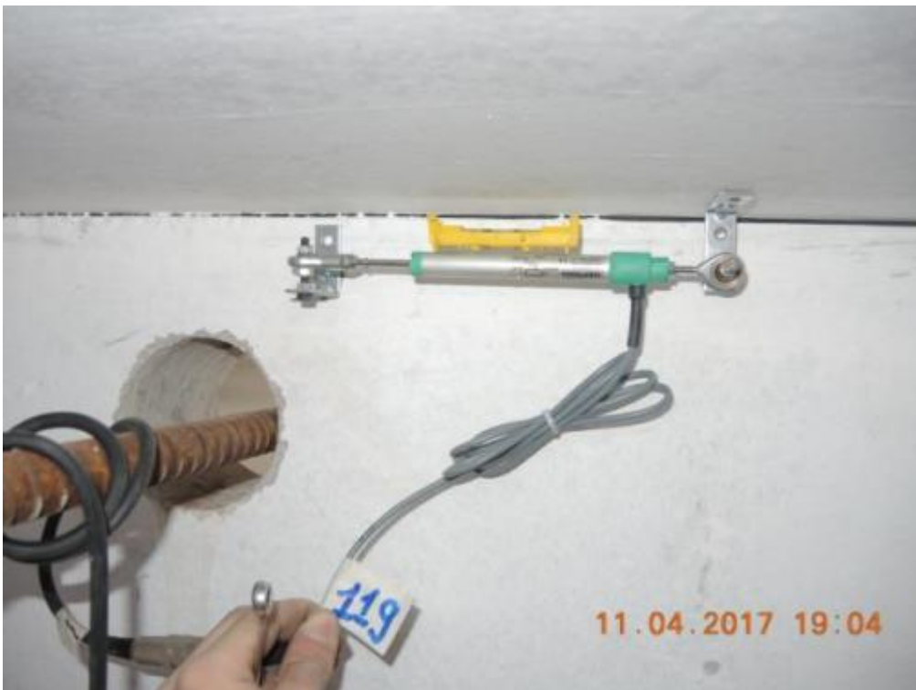
Figure 74. Detail of post-tensioned bars and clearance with respect to the stability wall panel.
