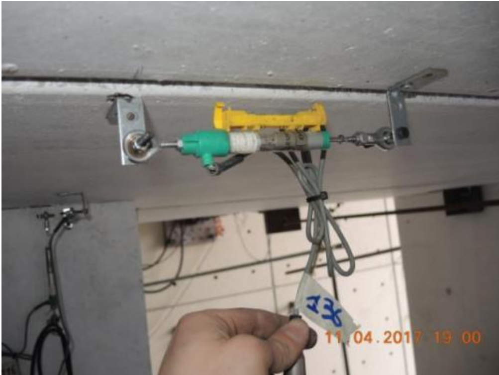
Figure 129. Instrumentation installed for relative displacement between slab panels – Opposite side.
