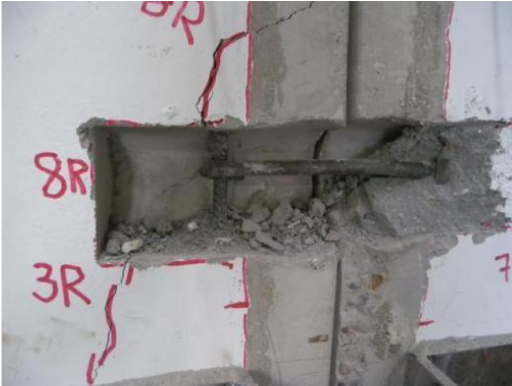
Figure 361. Detail of flexural failure mechanism of a hooked connector – Above the bottom down clip.
