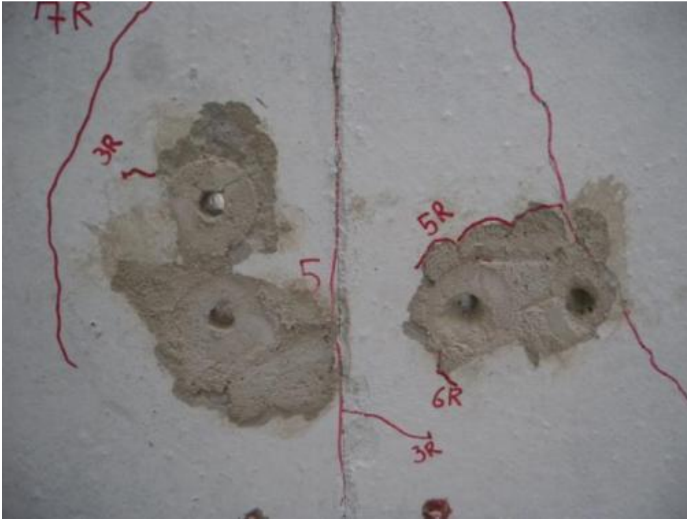
Figure 365. Removal of screwed clip angles and damage/crack pattern in the transversal wall panels.
