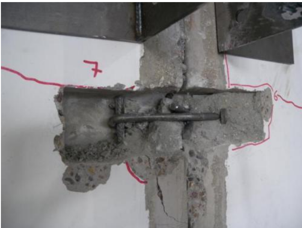
Figure 362. Detail of flexural failure mechanism of a hooked connector – Below the top clip.
