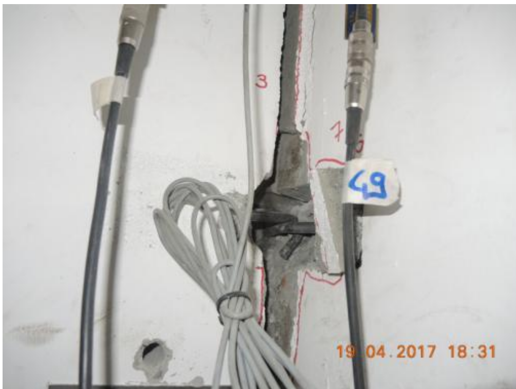
Figure 304. Enlarged view of flexural failure mechanism of a three-way anchor – West side, first storey.
