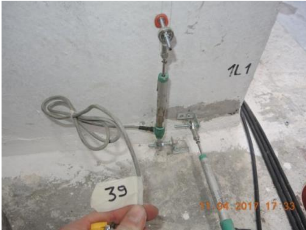
Figure 117. Detail of the instrumentation installed at the base of a lateral wall.
