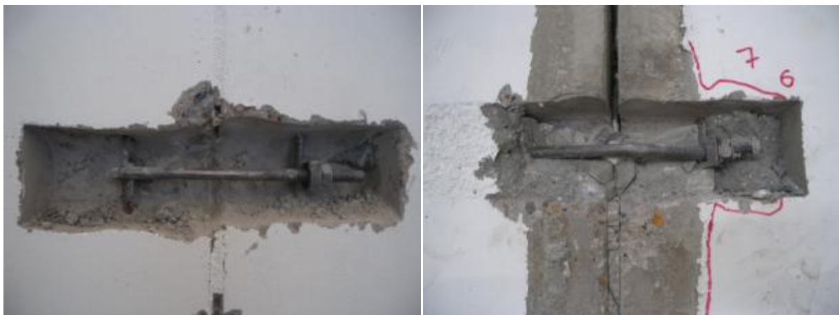
Figure 3. Arrangement of hook reinforcement in EUC-BUILD4 specimen and flexural failure mechanism.
