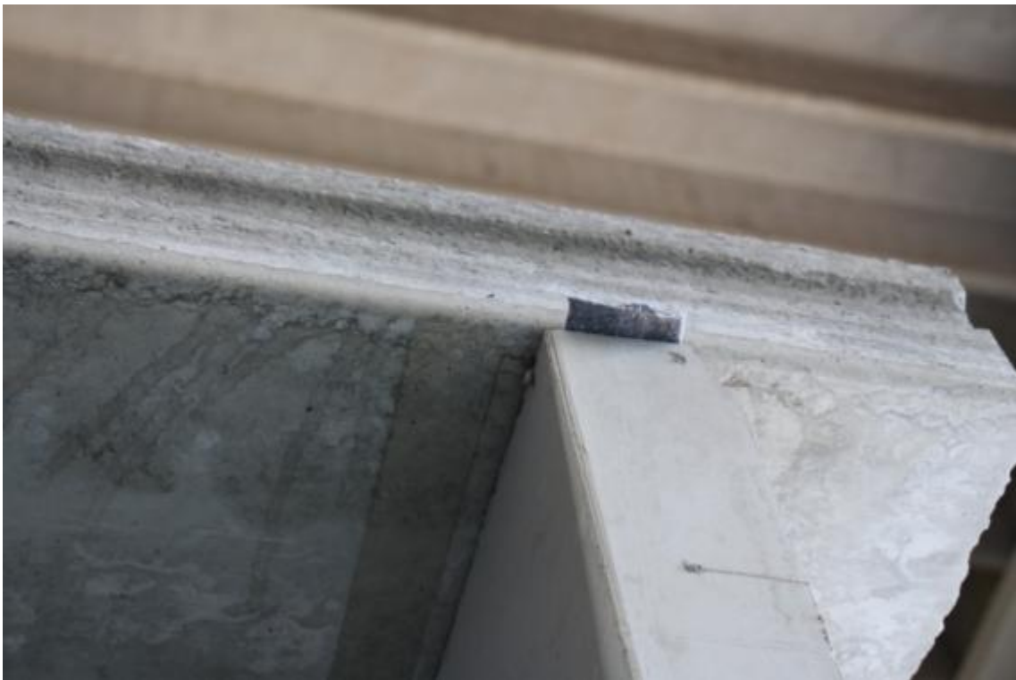
Figure 35. Detail of fabric felt underneath precast slabs, as well as of 250 mm overhang in wall-slab joints.
