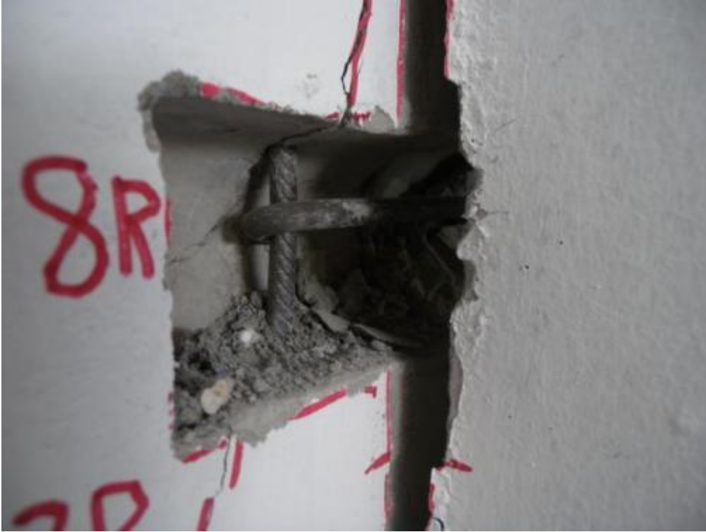
Figure 352. Enlarged view of bent hook reinforcement before dismantling of wall panels – First storey.
