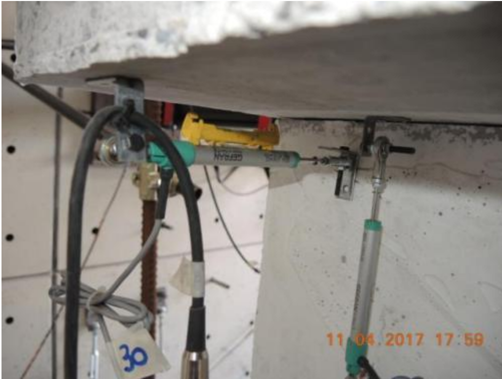
Figure 115. Potentiometers installed onto the top of the lateral walls - Second storey, opposite side.
