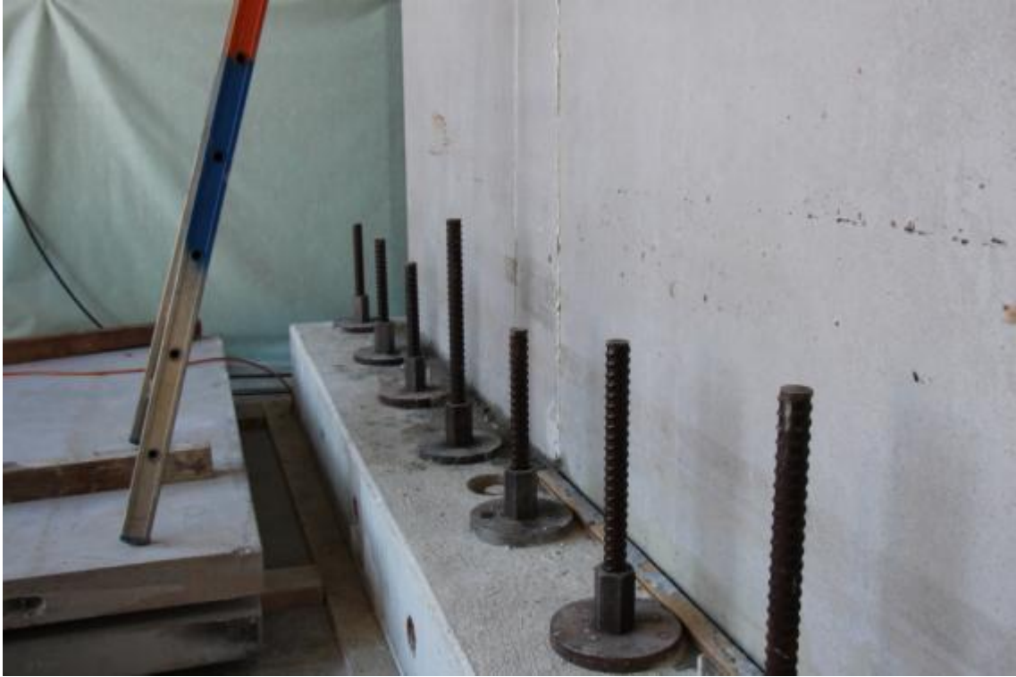
Figure 26. Detail of a mortar joint at the base of EUC-BUILD4 specimen – lateral wall.
