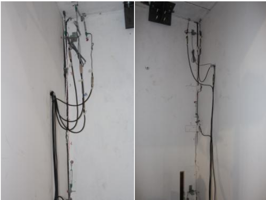
Figure 201. Failure of three-way connection and complete gap opening between the stability and lateral walls.
