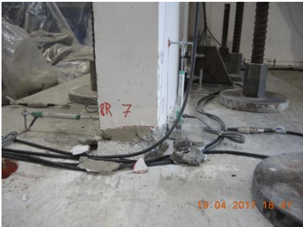
Figure 310. Transversal wall W1L1 after removal of crushed concrete – West side, lateral face, edge.
