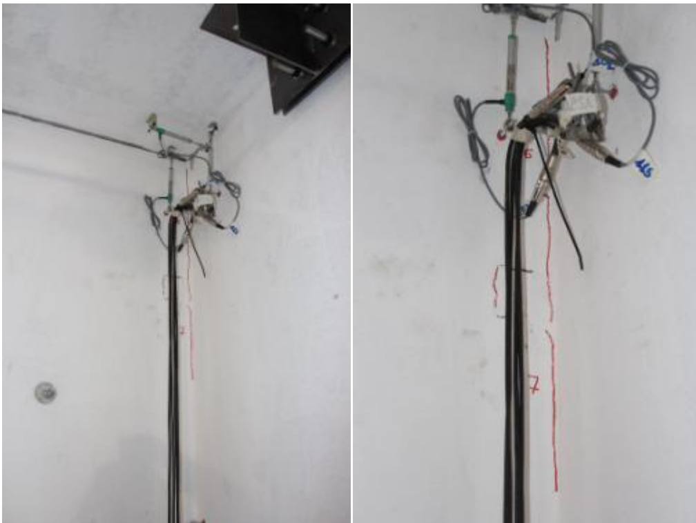
Figure 209. Vertical crack in the top three-way joint between the stability and lateral walls – Second floor.
