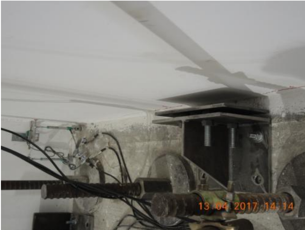
Figure 192. Detail of the crack pattern at the base of the transversal walls – South side.
