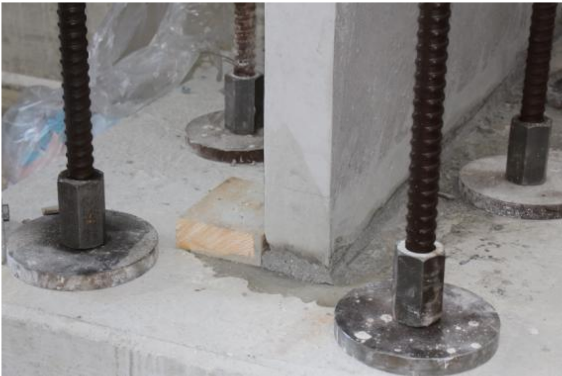
Figure 33. Detail of the mortar joint at the base of the opposite lateral wall – enlarged view.
