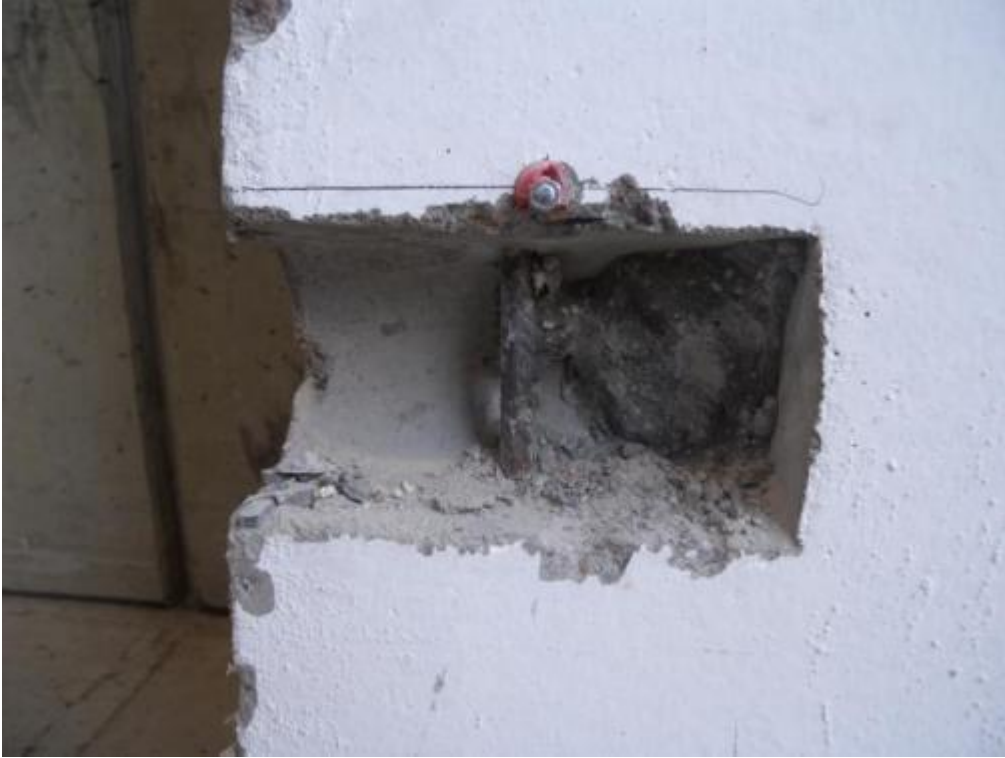
Figure 335. Detail of mortar in one of the niches for two-way panel-to-panel connection – Second-storey.
