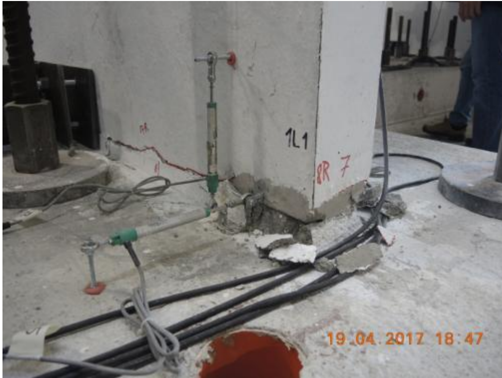
Figure 309. Lateral wall W1L1 after removal of crushed concrete – West side, South face, edge.
