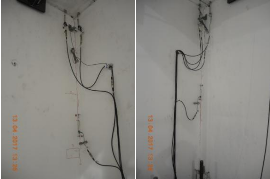
Figure 183. Three-way connection: propagation of crack pattern in the niches and along the wall height.
