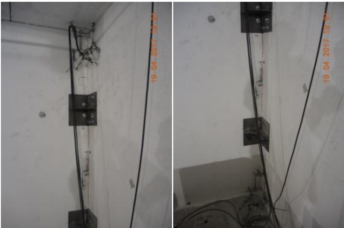
Figure 314. Damage pattern of retrofitted three-way connections – East side, North face, second storey.
