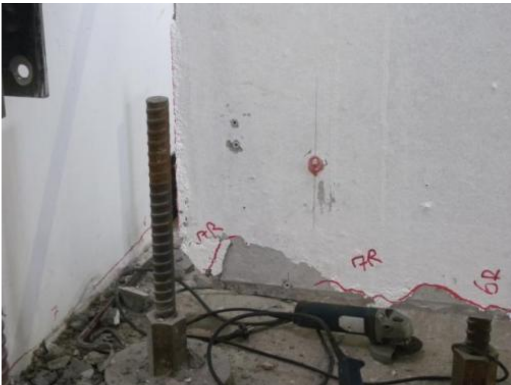
Figure 355. Ground-floor stability wall panel – Detail of damage at the base, South edge/corner.
