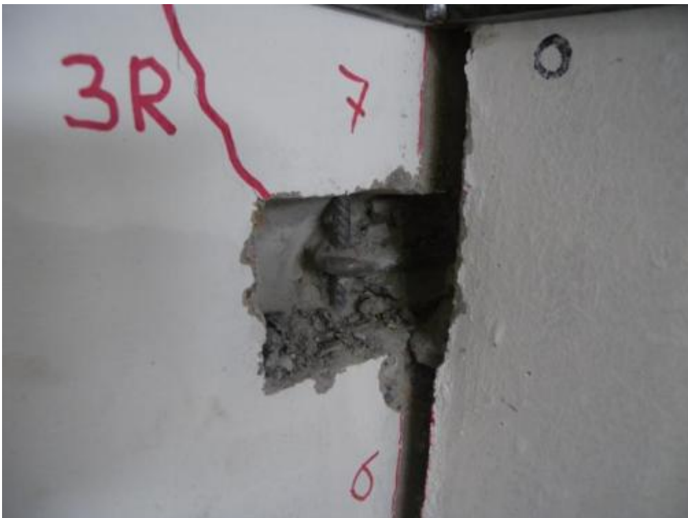
Figure 351. Detail of hooks and grout in a panel niche before dismantling of screwed steel angles.
