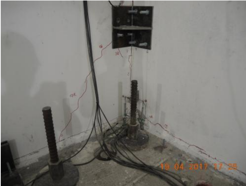
Figure 274. Propagation of inclined cracks running from the bottom steel angle to the lateral wall base.
