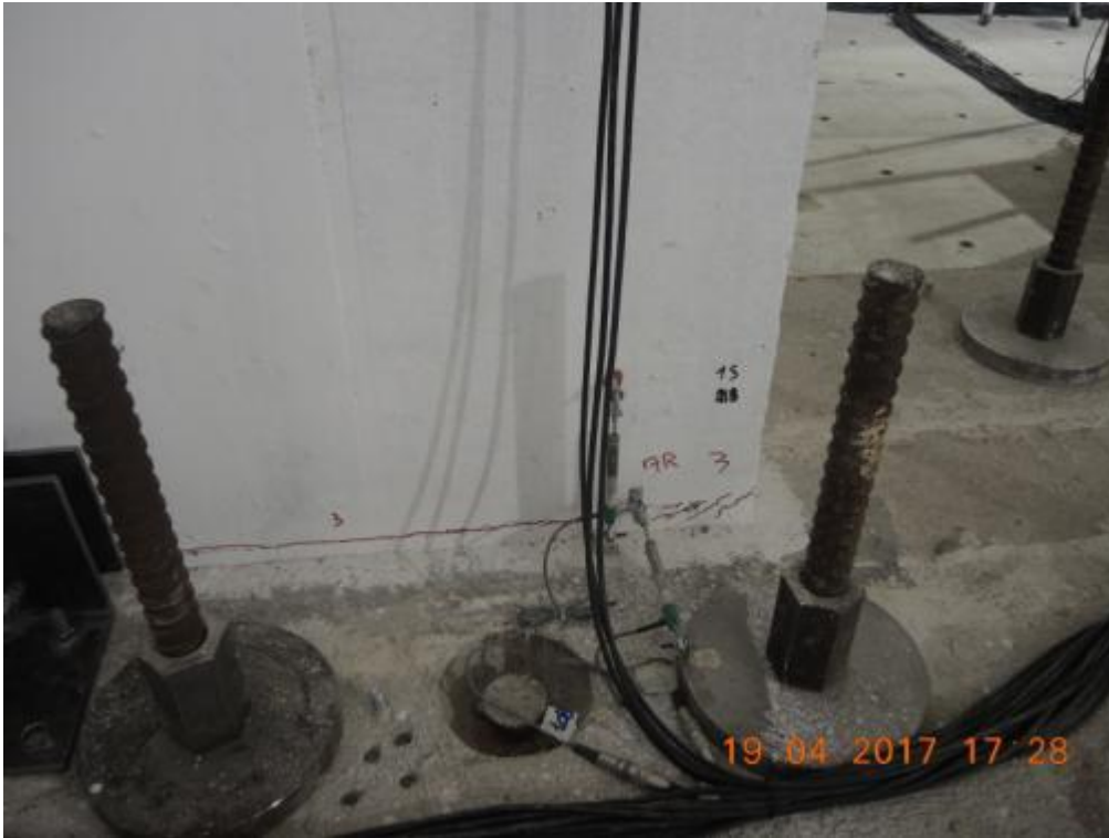
Figure 276. Damage/crack pattern at the base of the ground-floor stability wall – Opposite (North) side.
