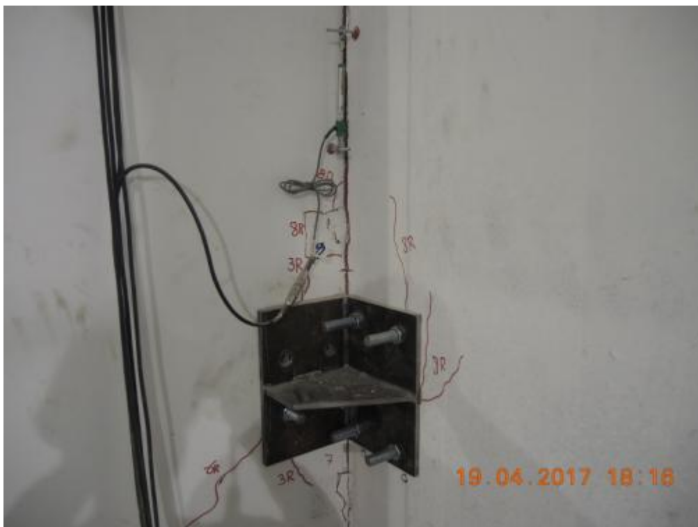
Figure 286. Crack pattern of transversal and stability walls – Bottom steel angle, East side.
