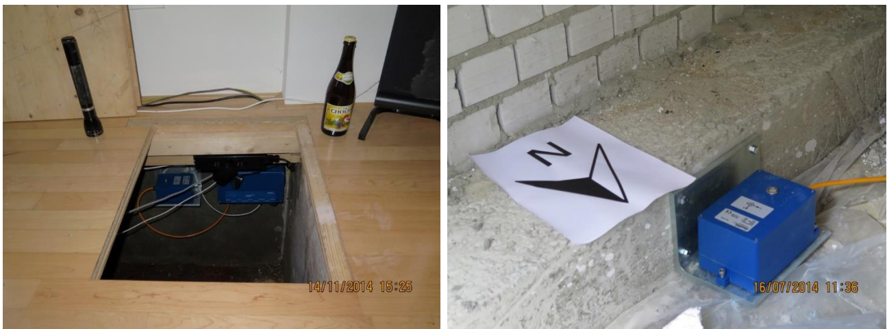
Figure 13.5. Examples of TNO accelerographs attached to foundation beams
