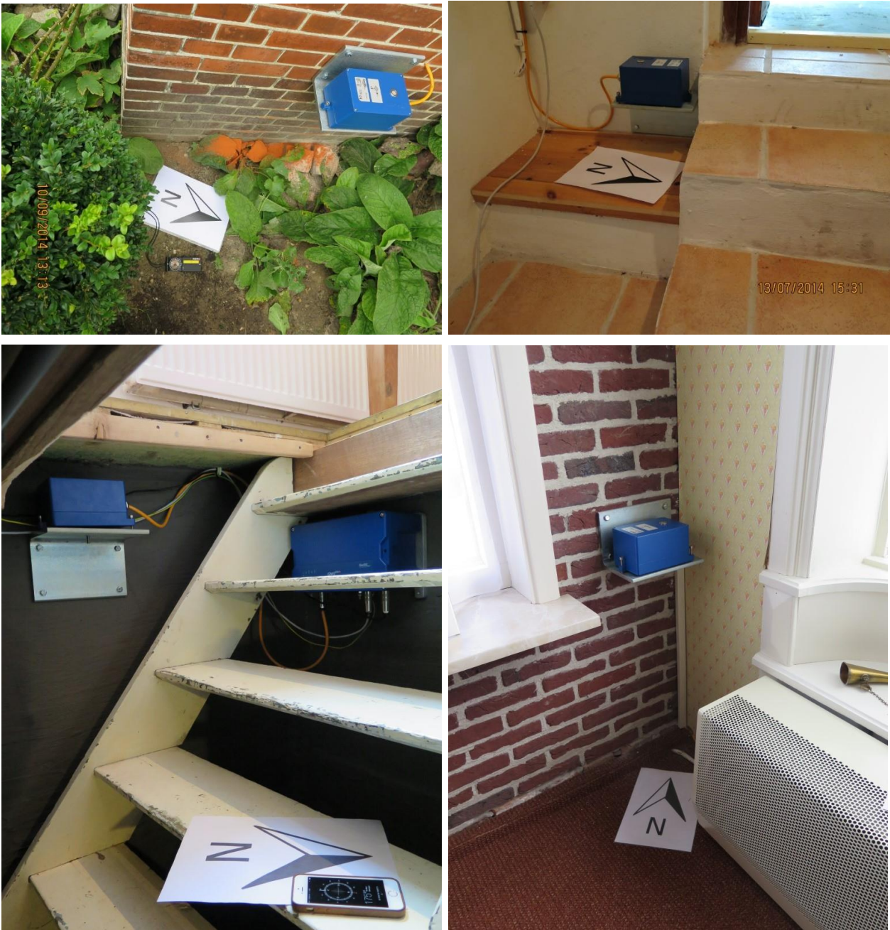
Figure 13.3. Examples of installation details of the TNO accelerographs; the lower left-hand image shows an instrument on the wall of the basement
