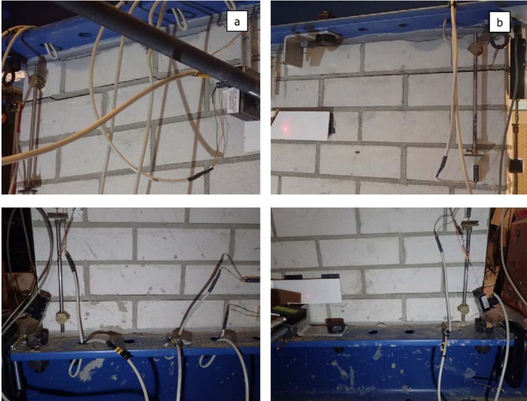
Figure 28: TUD-COMP-3: Rocking cracks at the top & bottom left corners (a) and top & bottom right corners (b)
