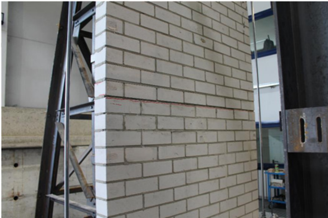
Figure 130: EUC-COMP-4: View of mid-height crack
