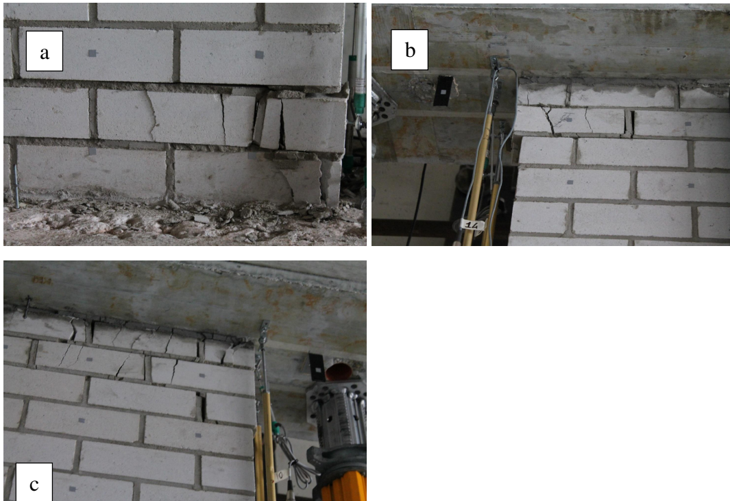
Figure 74: EUC-COMP-1: Toe-crushing damage at end of test (a) bottom right; (b) top left corner; (c) top right corner
