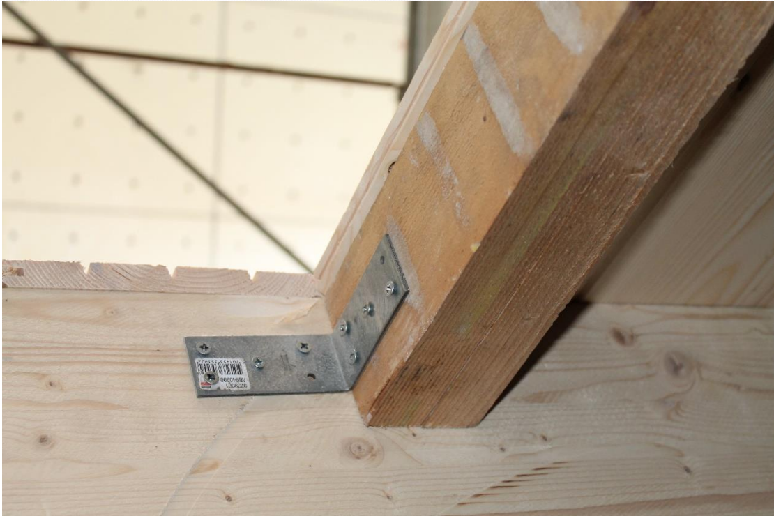
Figure 28. Detail of the connection between the timber beam of the opening and the girder
