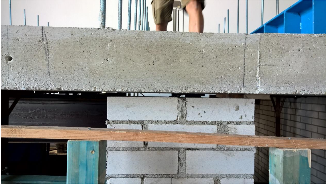
Figure 21. Detail of the connection between the r.c. slab of the second floor and the inner leaf (c.s. walls)- view of the gap - West side
