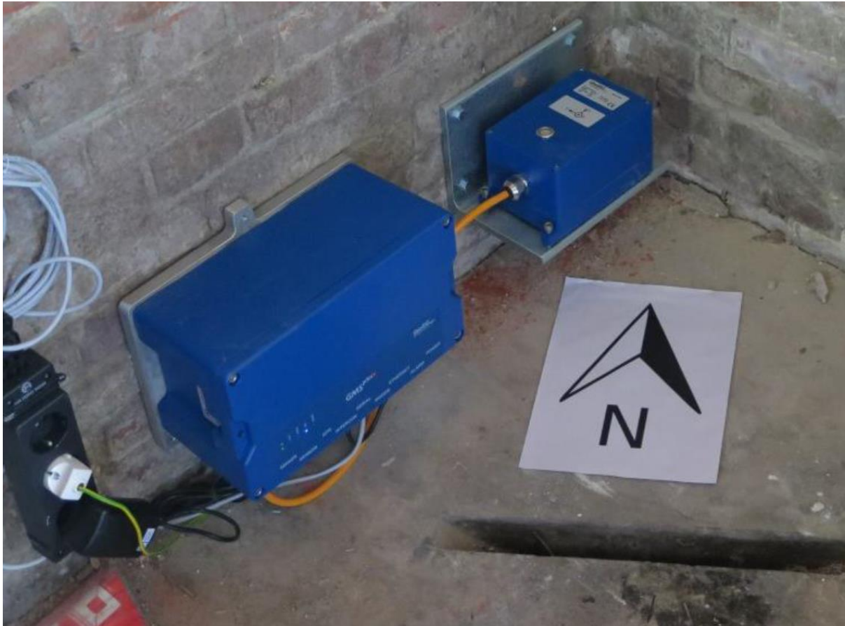
Figure 5.2 Vibration monitoring system – recorder (left) and sensor (right)
