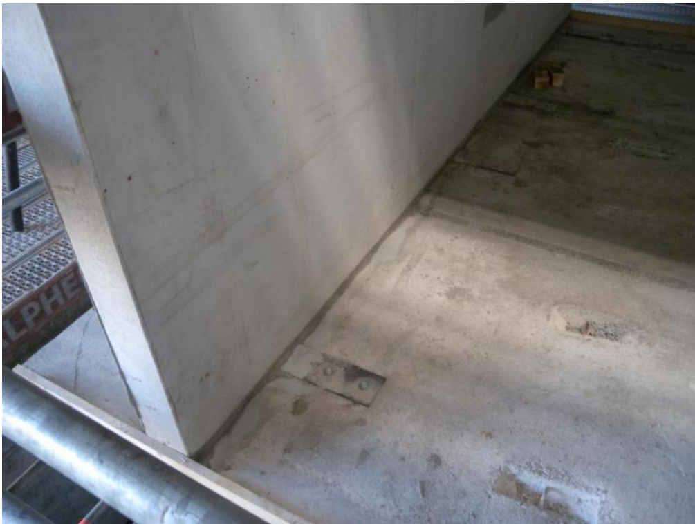
Figure 117. Key details – L-shaped panel-to-slab steel connector, anchoring of long side to slab, first storey.
