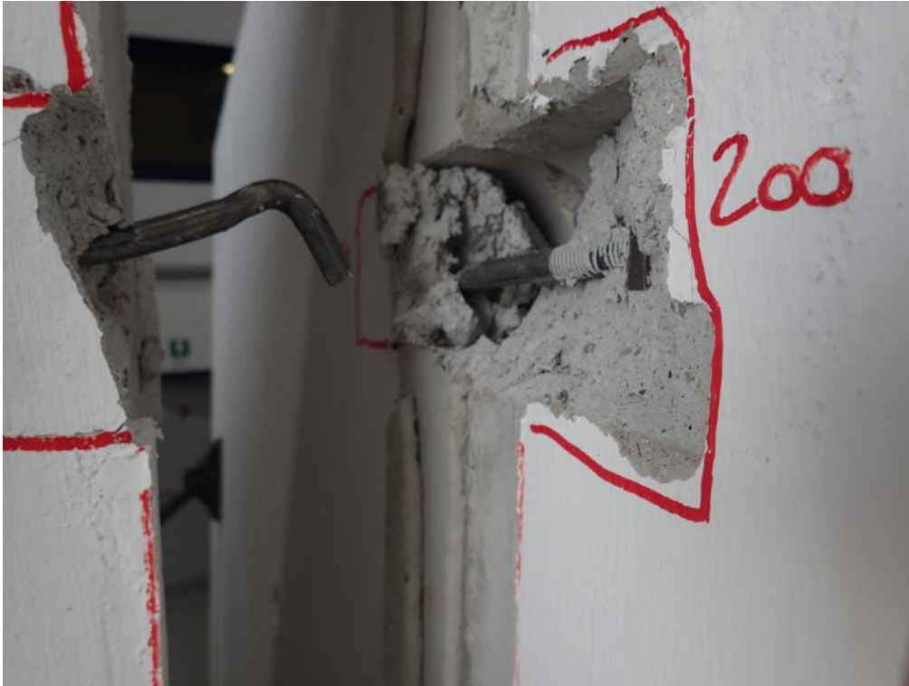
Figure 545. Enlarged view of steel hooks embedded in lateral and stability walls – Top connection.
