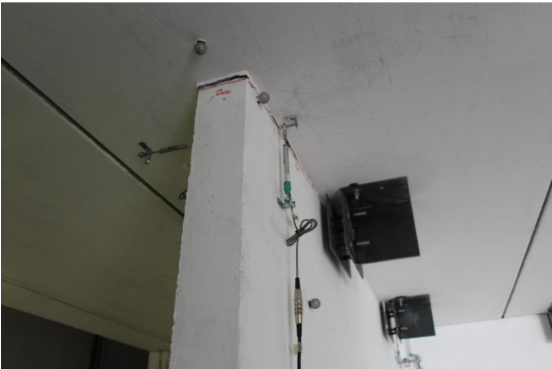
Figure 311. Full-depth/full-width crack of mortar joint between the second-storey stability wall and slab.
