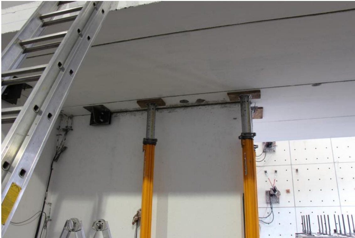
Figure 94. Propping-up of slab, to allow removal of felt layer and gap filling by means of non-shrink mortar.
