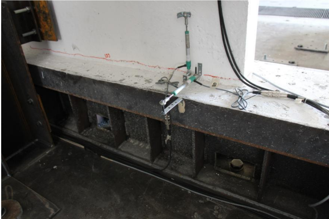
Figure 260. Crack running from the edge to the centre of the first-storey stability wall – East wall face.
