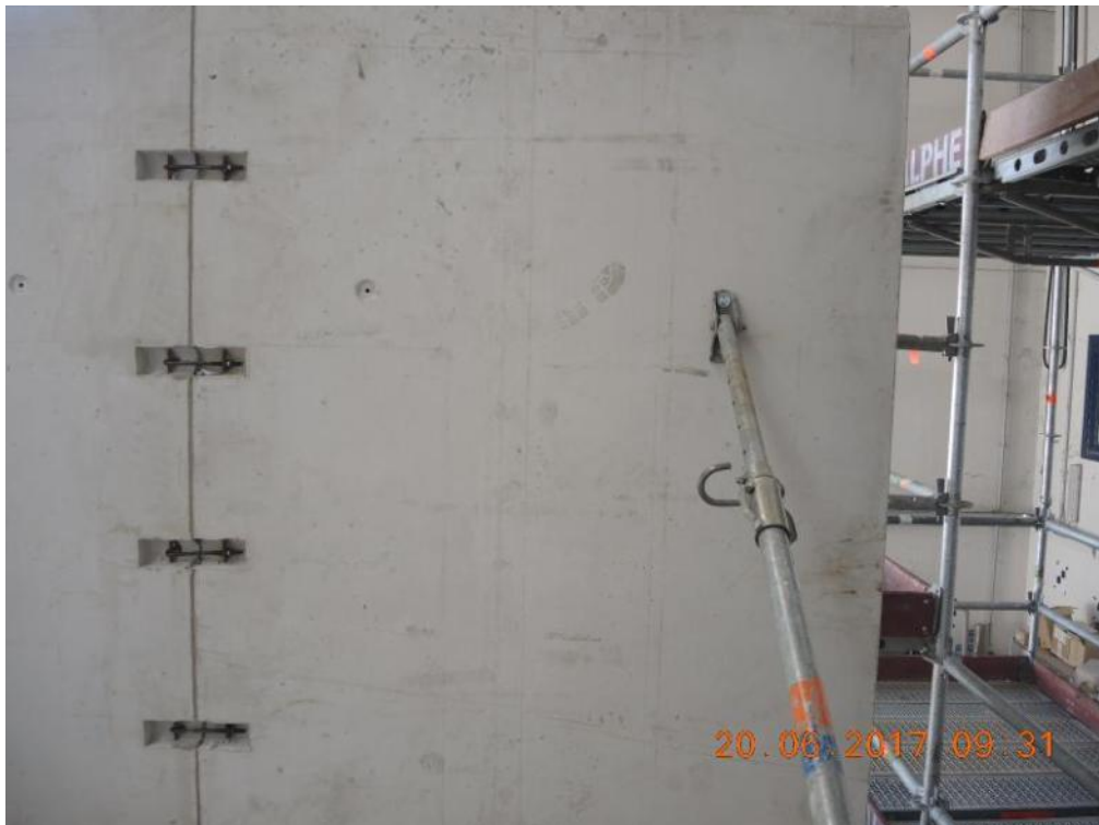
Figure 115. Key details – Two-way connections and temporary props for lateral stability during erection.
