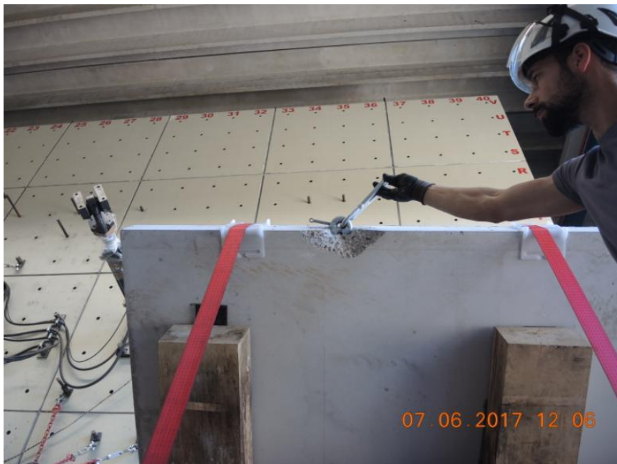
Figure 98. Detail of a stability wall panels featuring some damage in one of the lifting hook areas.
