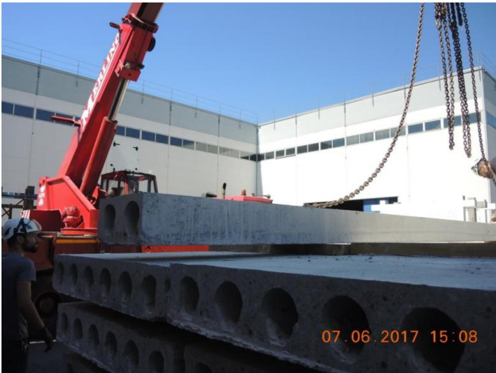
Figure 111. Uplift and transportation of precast slab panels – Detail of a 400 mm wide panel.
