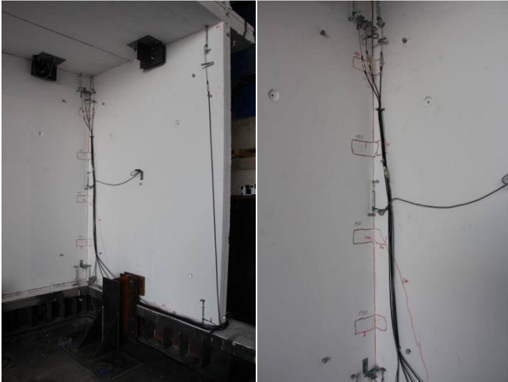
Figure 294. Crack pattern of the ground-floor stability wall – Enlarged view and detail of three-way joints.
