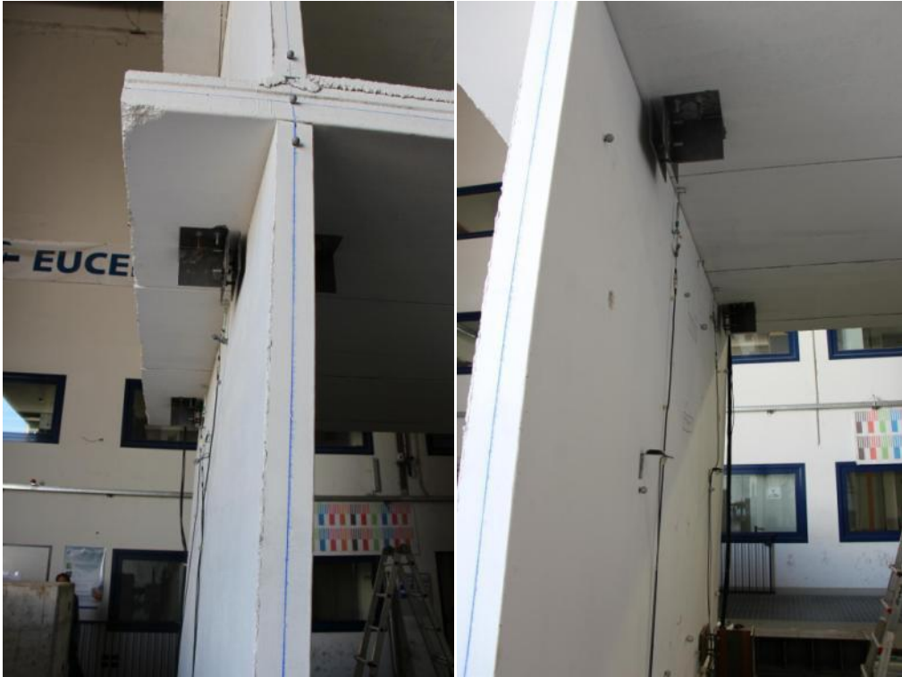
Figure 330. North-sided ground-floor lateral walls at the end of testing – North and South wall faces.
