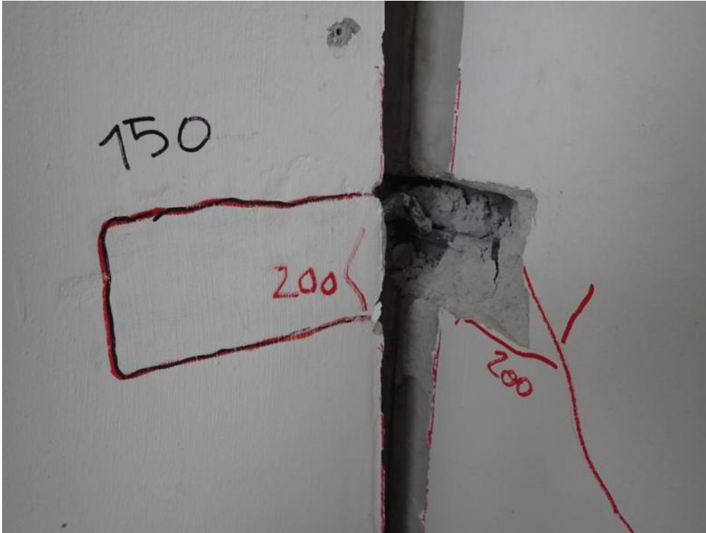
Figure 549. Damage of steel connectors between stability and lateral walls – Second joint from the base.
