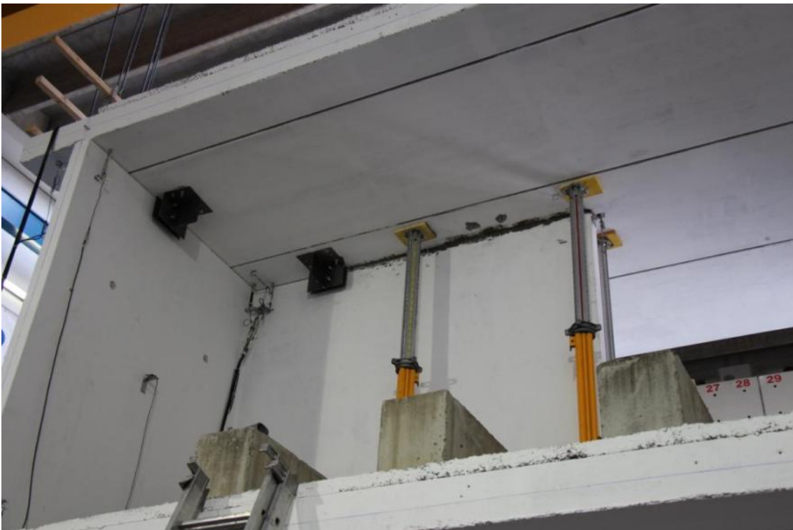
Figure 167. Mortar filling at the second-floor gap – Overall view of the mortar layer.
