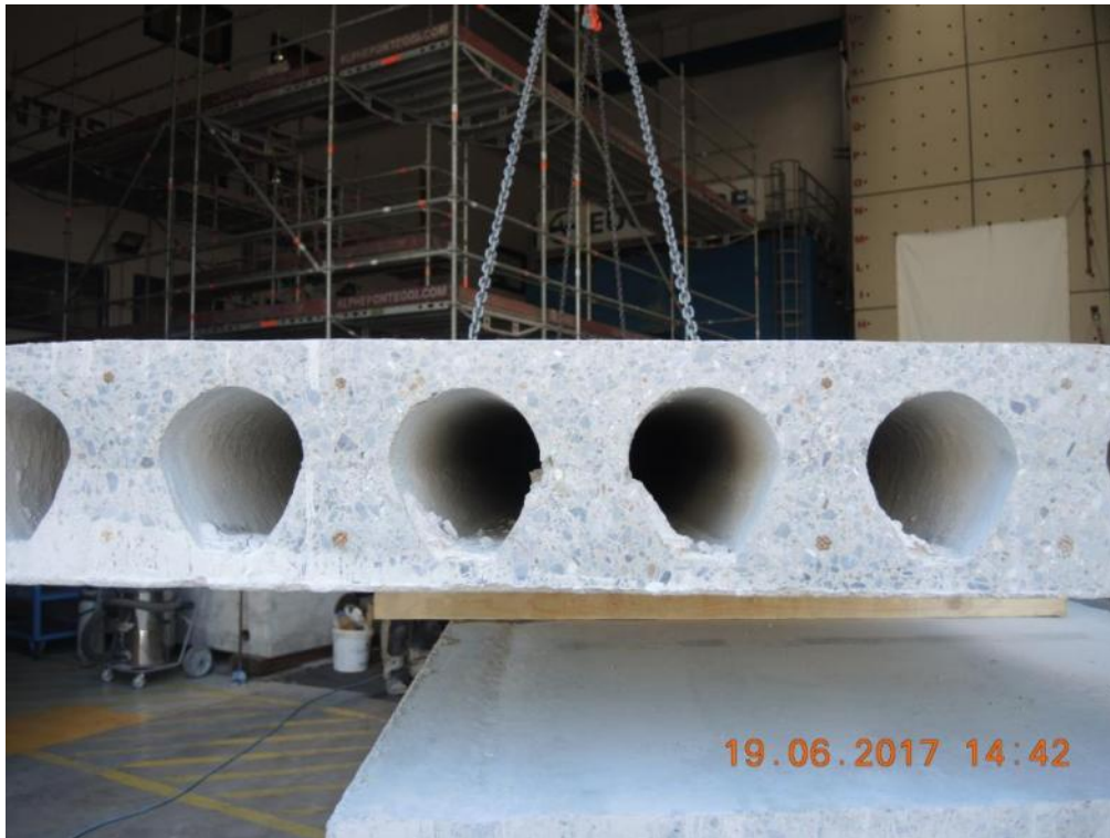
Figure 126. Crane-induced uplift of a precast slab panel for flooring the first-storey of EUC-BUILD5 specimen.
