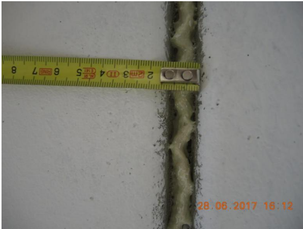
Figure 157. Enlarged view of the gap between the slab panels of EUC-BUILD5 specimen.
