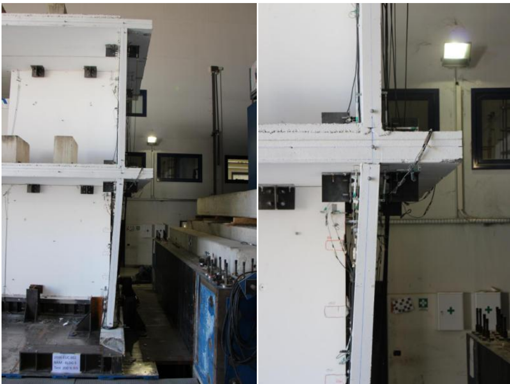
Figure 329. Overall and detailed views of the South-sided transversal walls at the end of testing.
