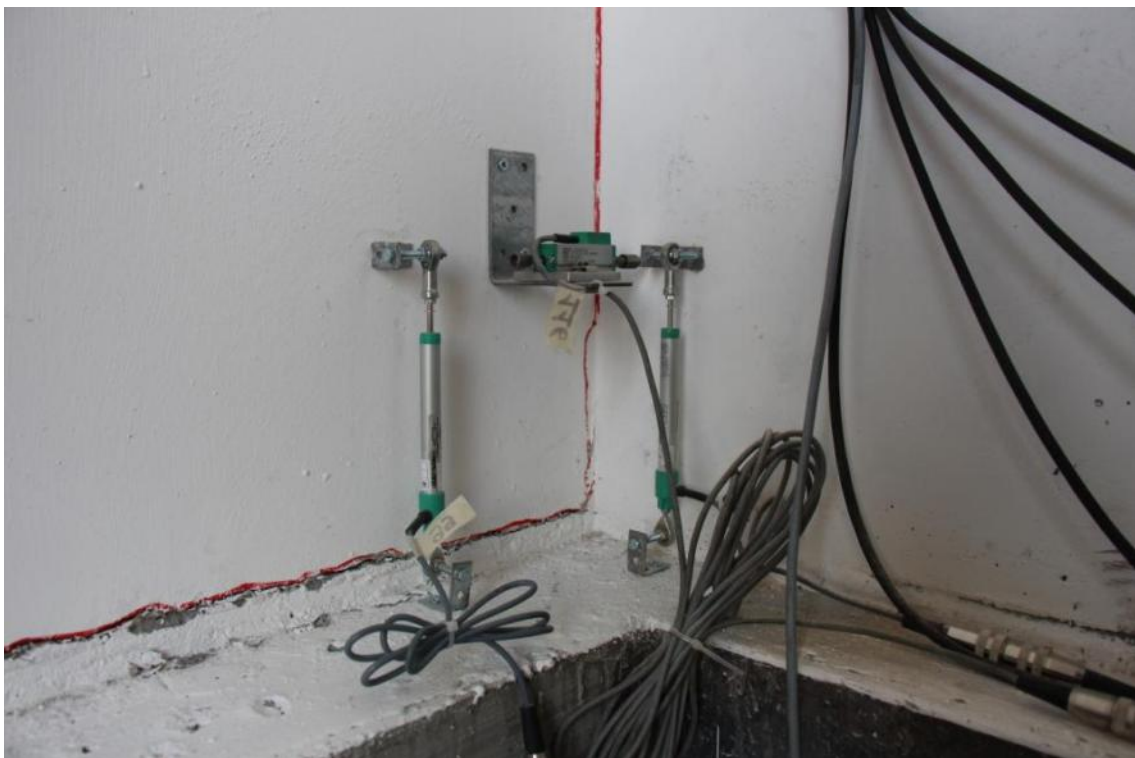
Figure 271. Vertical crack along the height of the first-storey stability wall – South edge.
