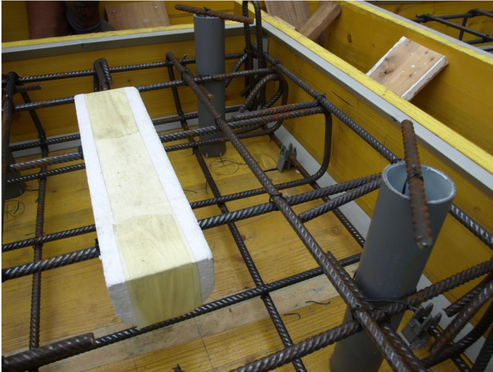
Figure 55. Detail of reinforcing rebars and polystyrene block in one of the wall stripes – Horizontal panel.
