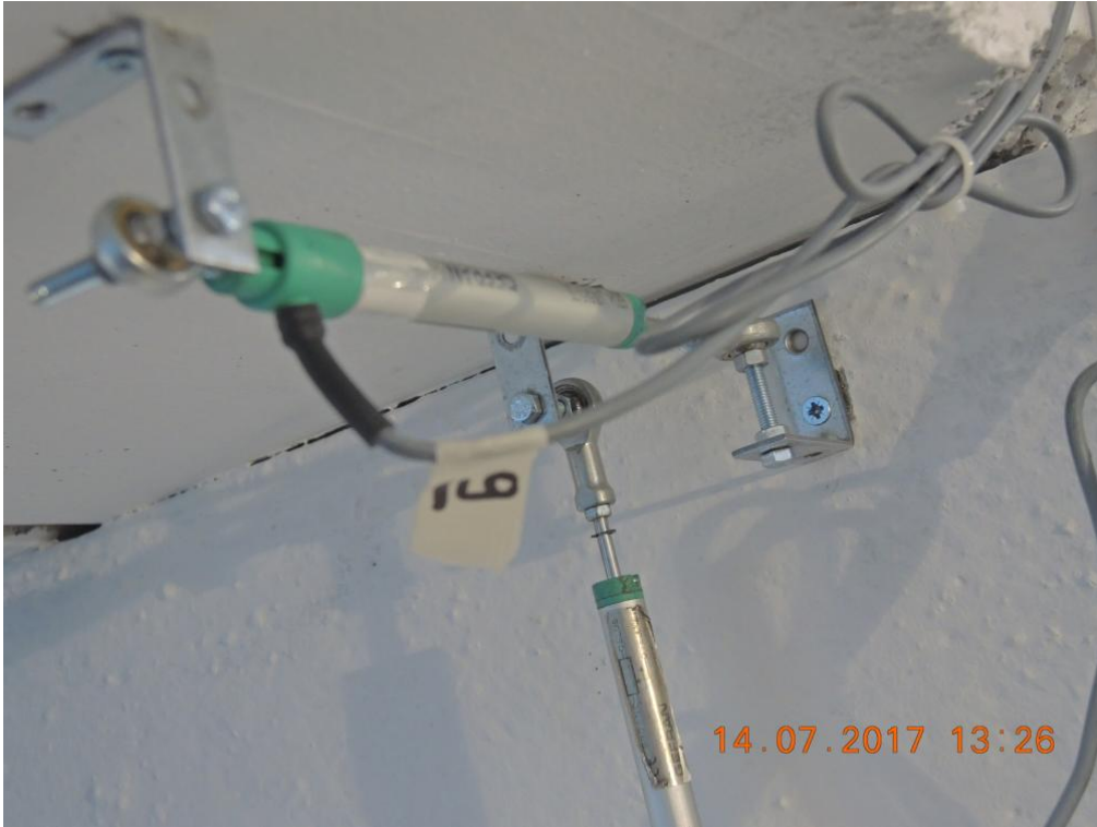
Figure 209. Instrument at the top of the second-storey South-East-sided lateral wall – East corner.
