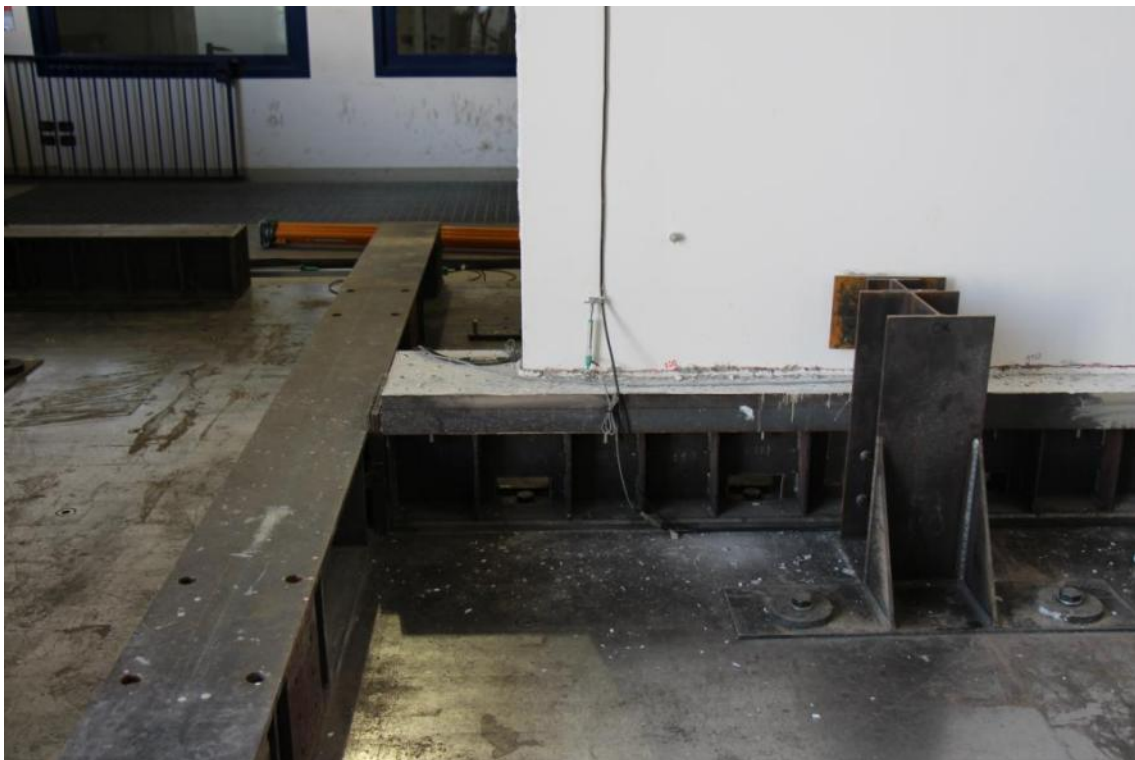
Figure 321. Sliding and concrete crushing at the base of the first-storey stability wall – West-side view.
