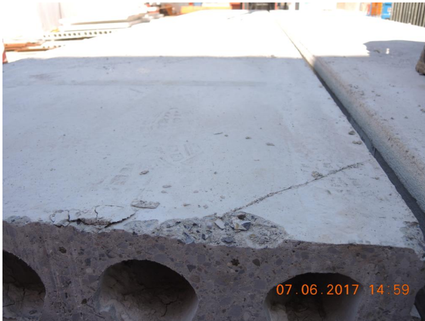
Figure 97. Example of precast hollow core slab panel and detail of minor scratch at one of its ends.
