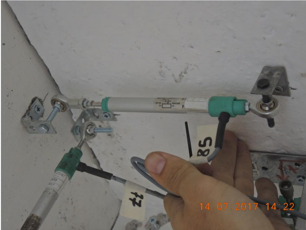
Figure 223. Instrumentation at the top of the second-storey stability wall.
