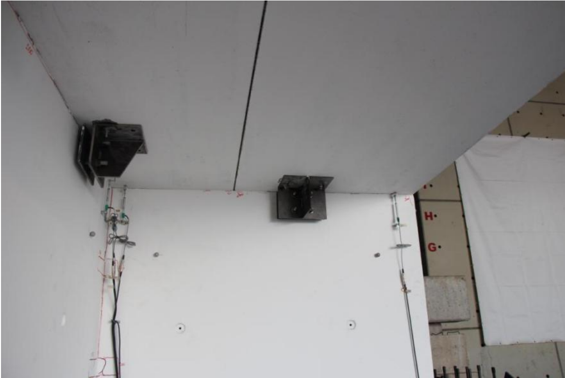
Figure 306. Concrete damage/chipping at the top of the first-storey lateral wall 1L2.
