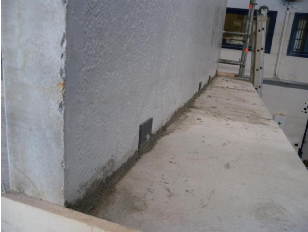
Figure 142. Panel-to-slab steel plate connectors after mortar filling grouting underneath panels – South side.
