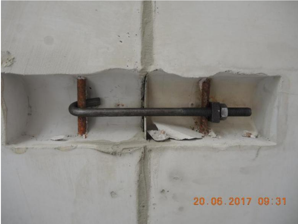
Figure 116. Key details – Arrangement of two-way connections and anchoring system for hook connectors.
