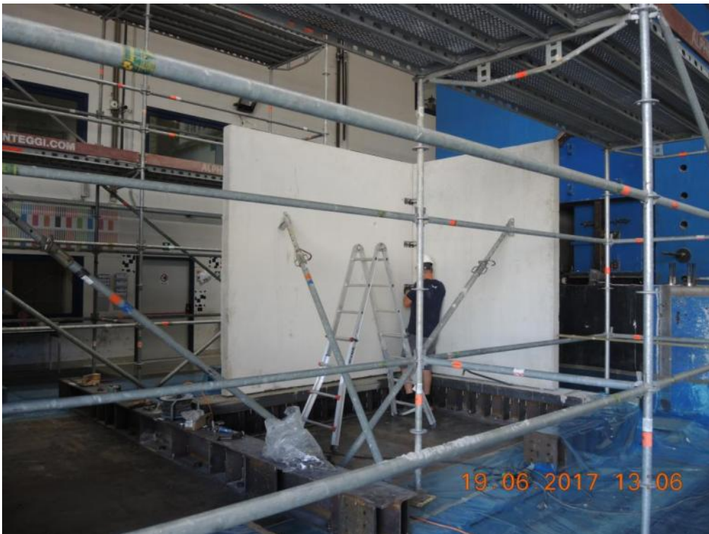
Figure 123. Erection of the first-storey stability wall on the steel foundation and fastening of steel connectors.
