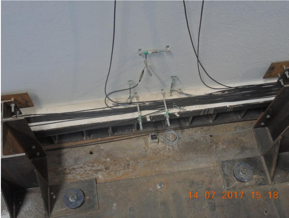
Figure 201. Instruments at the base of the South-sided transversal walls – First storey, South wall face.
