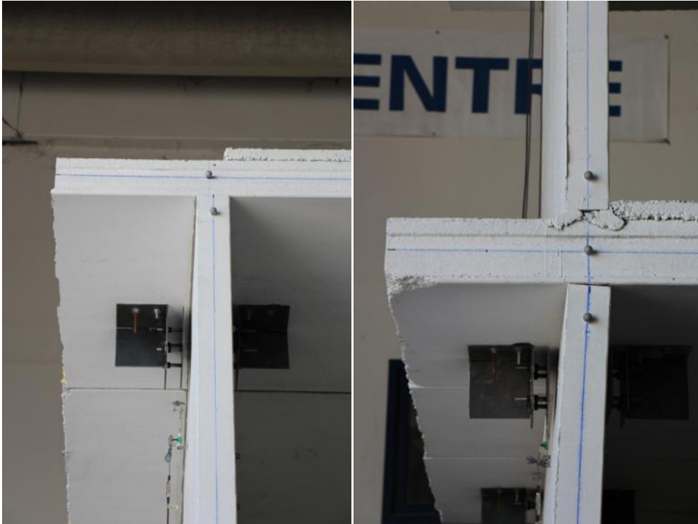
Figure 328. Detailed views of the first-storey and second-storey slabs and North-sided lateral walls.
