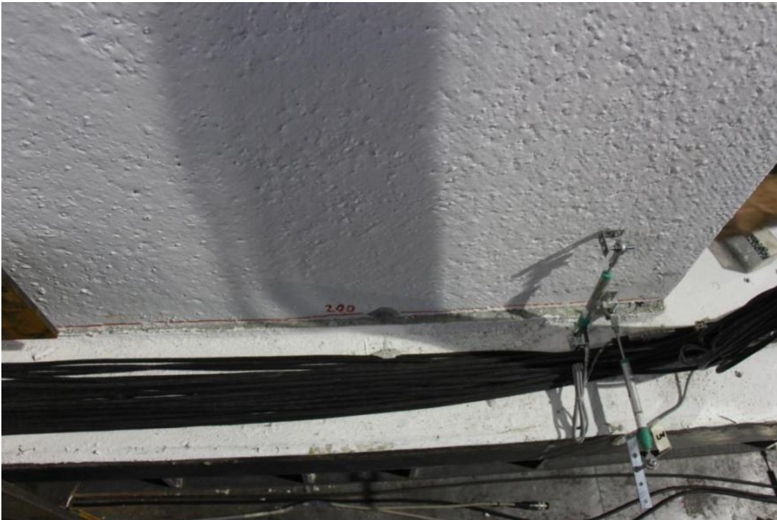
Figure 301. Full-depth/full-width horizontal crack at the base of the first-storey lateral wall 1L1.
