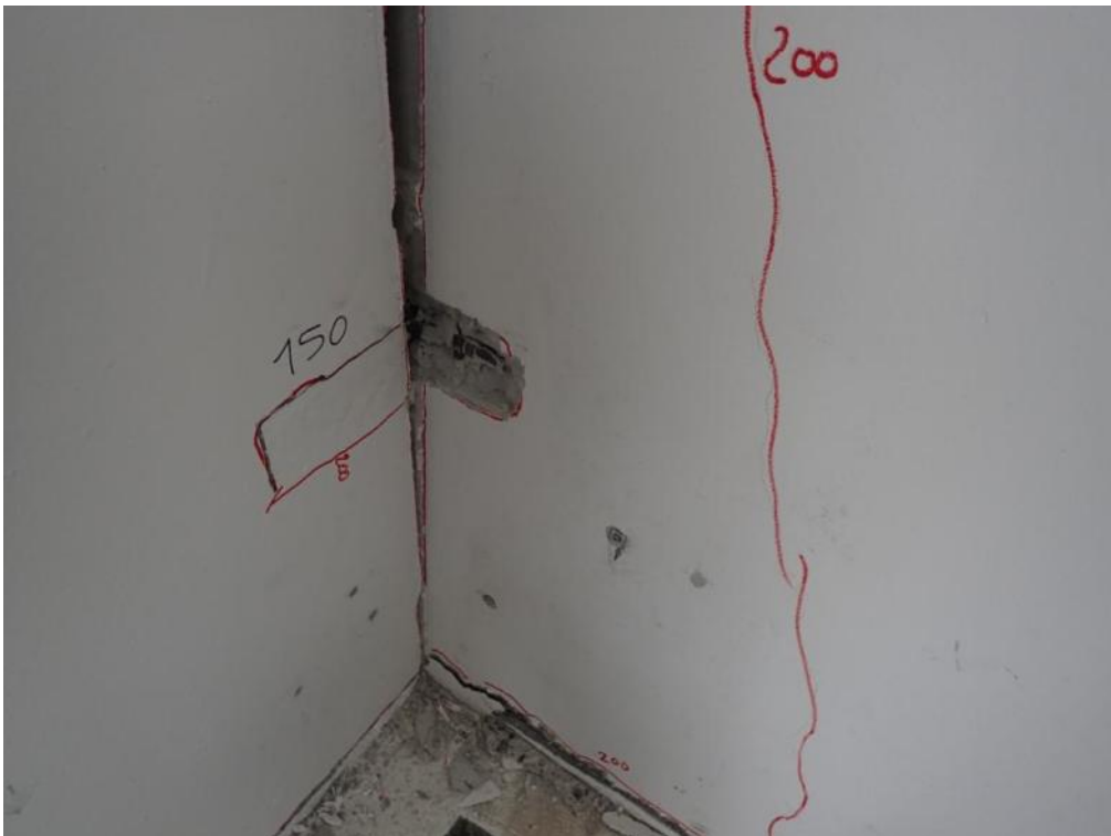
Figure 552. Damage pattern of the bottom three-way connection between stability and lateral walls.
