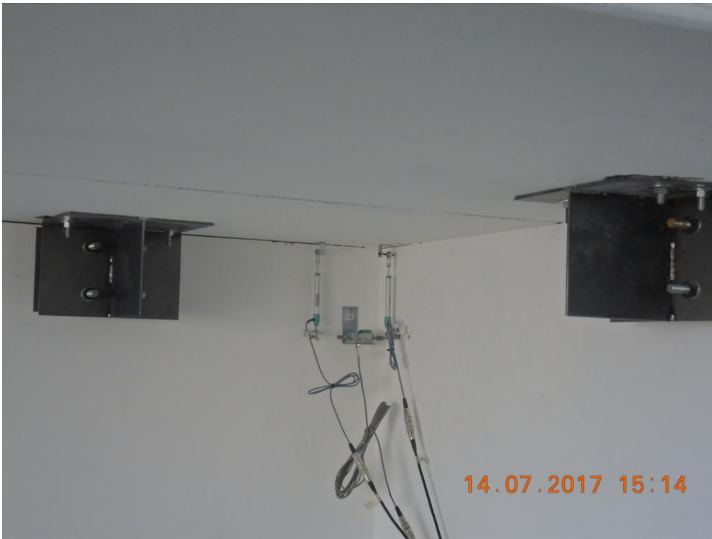
Figure 197. Instruments installed at the top of stability wall and counterpart lateral wall.
