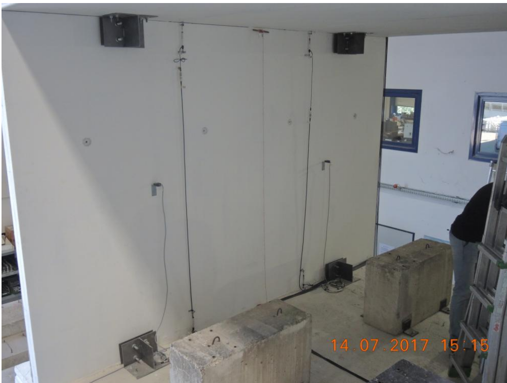
Figure 198. Instrumentation installed on the North-sided transversal walls – Second storey, South wall face.
