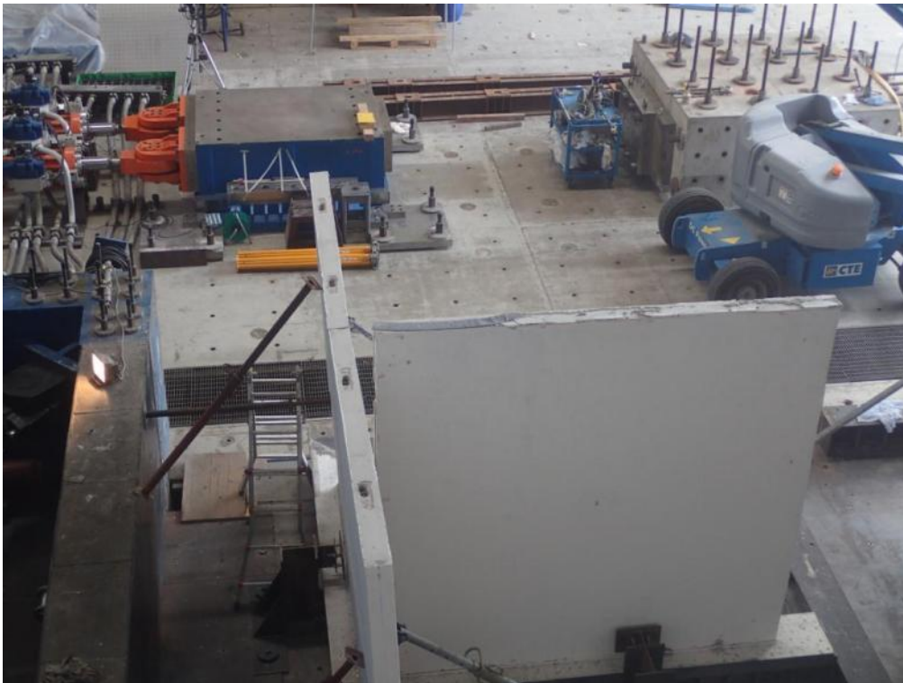
Figure 540. Top view of stability and transversal walls after dismantling of the first-storey slab.
