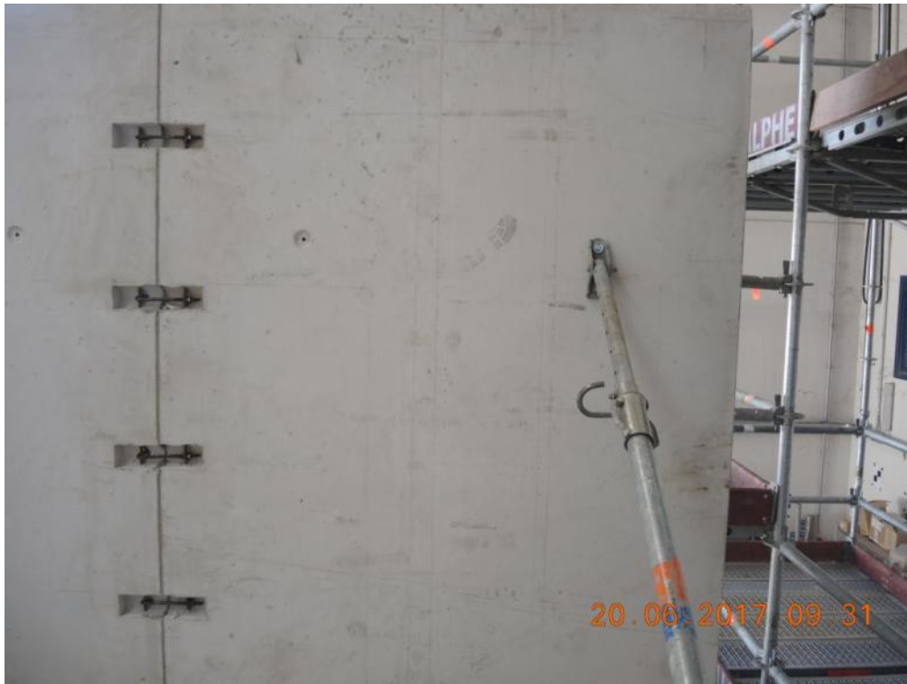
Figure 130. Detail of the installed temporary props – Anchorage to precast wall panels of the second storey.
