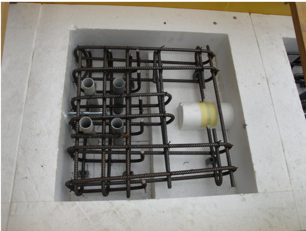
Figure 56. Detail of reinforcing rebars and polystyrene block in one of the wall stripes – Vertical panel.
