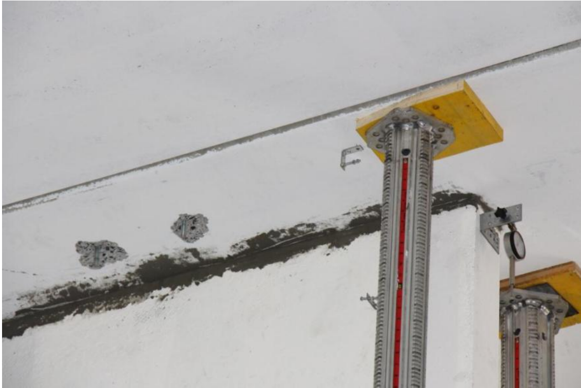
Figure 168. Mortar filling at the second-floor gap – Detailed view of the mortar layer.
