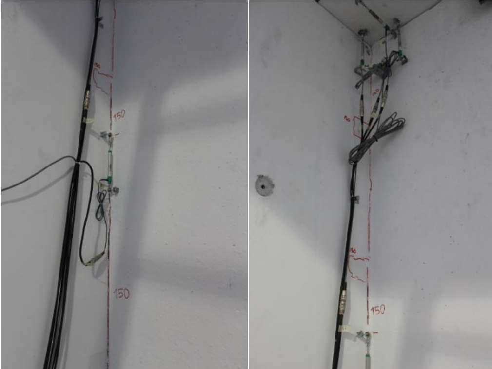
Figure 282. Crack pattern of three-way joints – East and West faces of the ground-floor stability wall.
