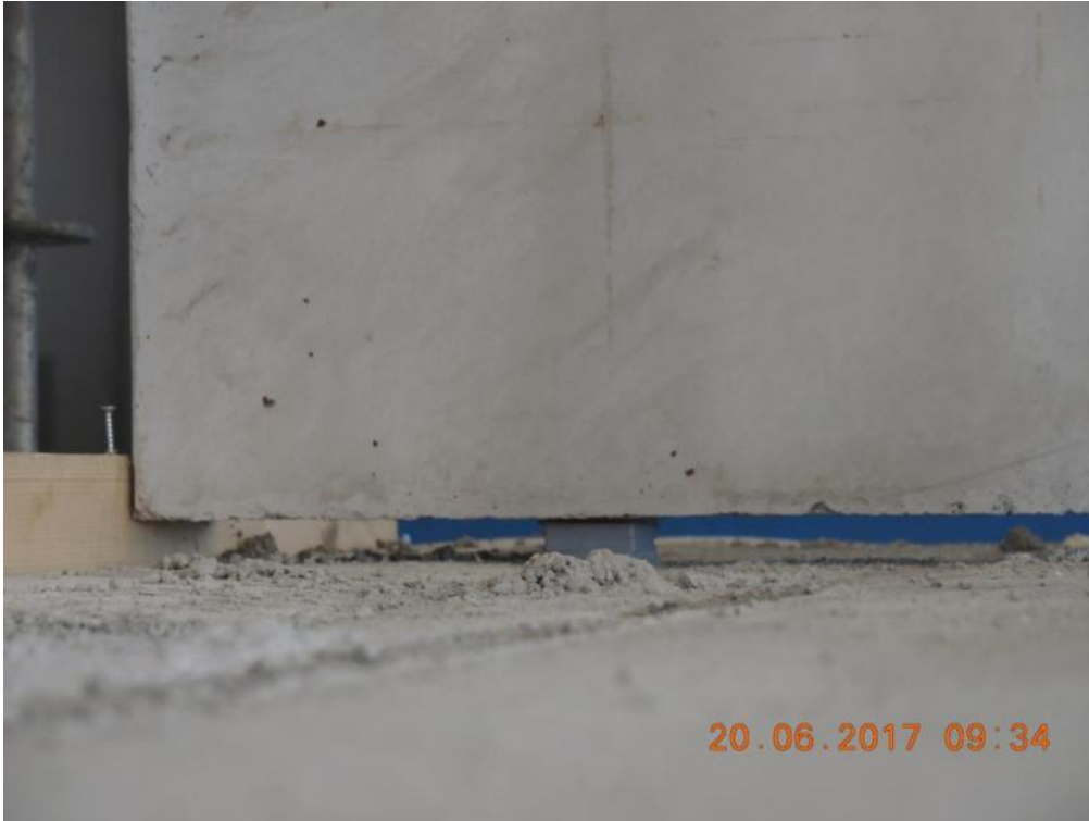
Figure 134. Detail of a spacer underneath the second-storey transversal walls for mortar grout.
