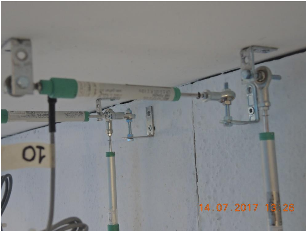
Figure 210. Instrument at the top of the second-storey South-East-sided lateral wall – West corner.
