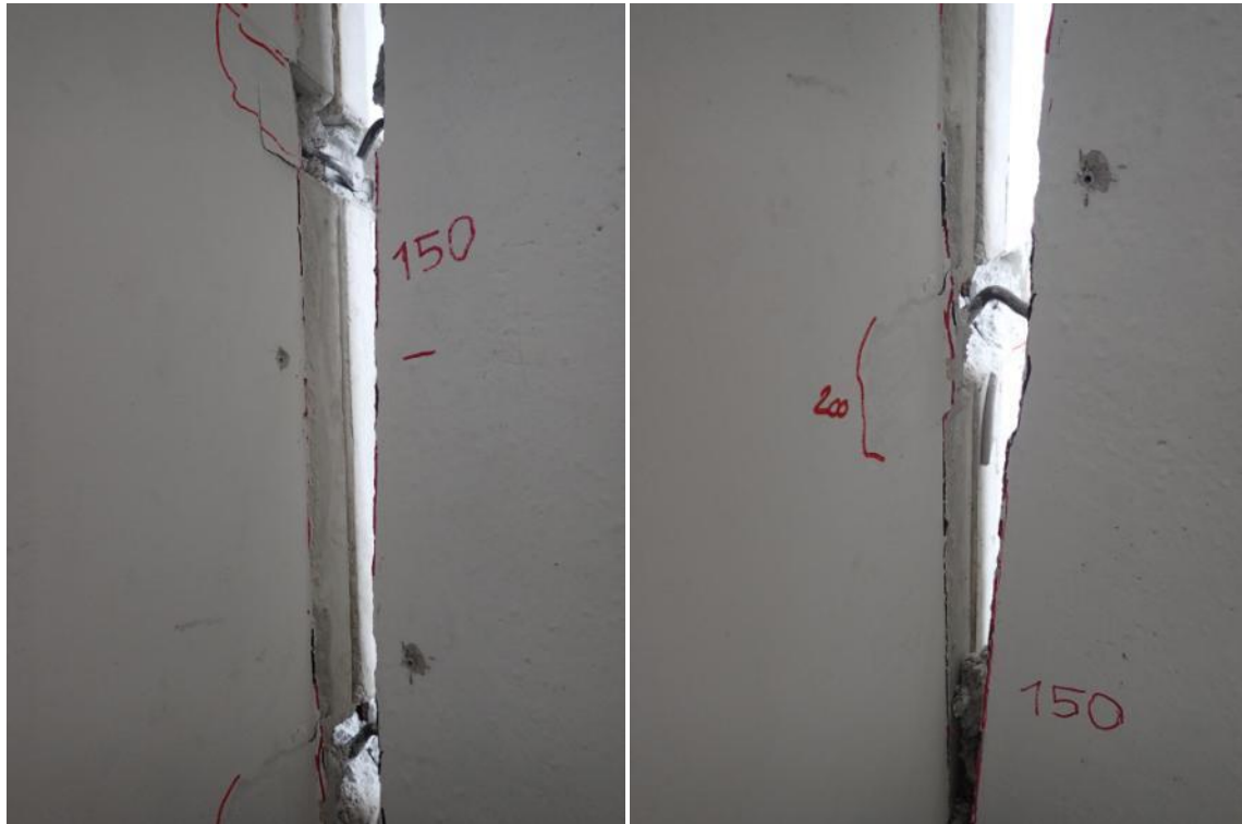
Figure 542. Permanently-bent steel connectors embedded in the sockets of the stability wall.
