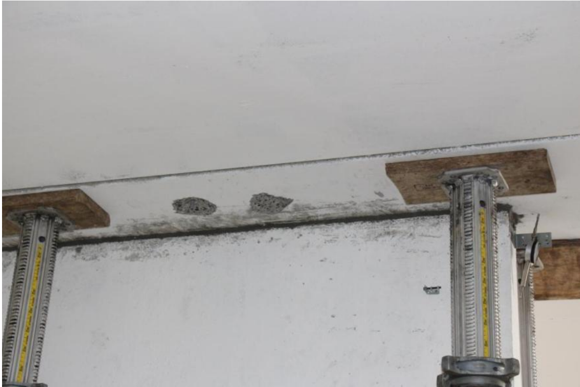
Figure 160. Mortar filling intervention at the first-floor gap – Overall view of the mortar layer.
