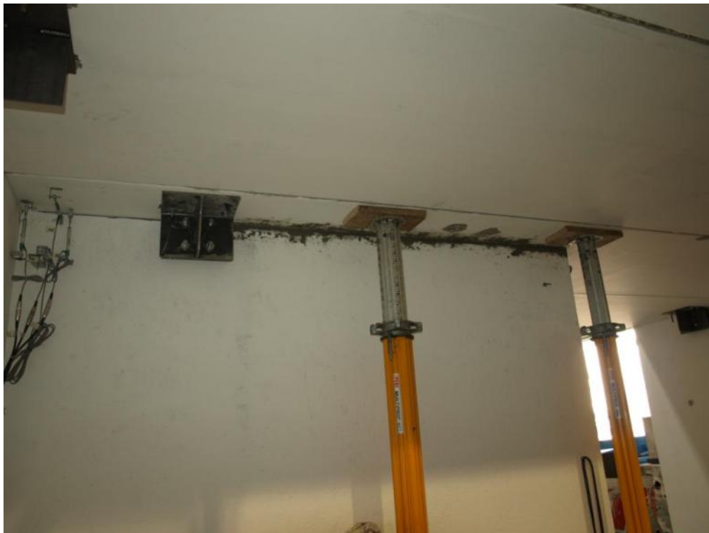
Figure 163. Mortar filling intervention at the first-floor gap – Overall view of the East-sided wall face.
