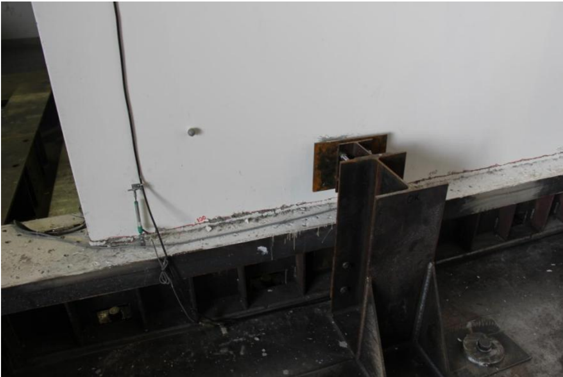
Figure 297. Full-depth/full-width horizontal crack at the base of the first-storey stability wall.
