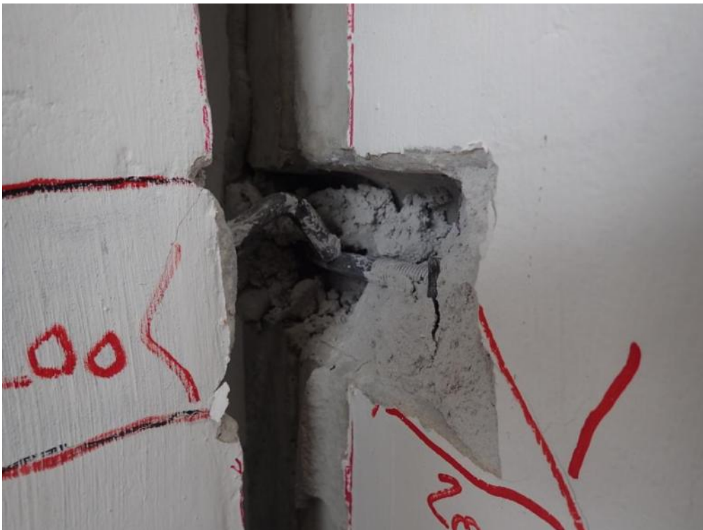
Figure 550. Enlarged view of failed steel connectors in the second panel joint from the base.
