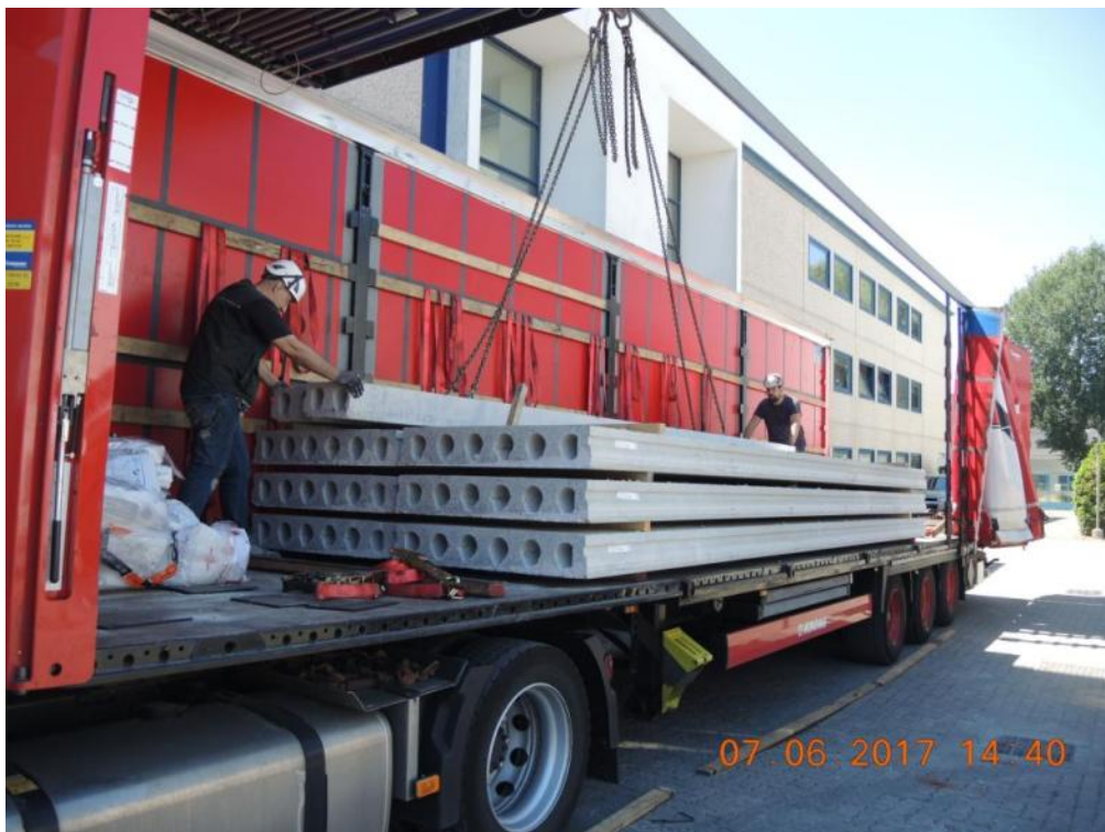
Figure 107. Crane-induced uplift of precast slab panels – Detail of the adopted four-points lifting scheme.
