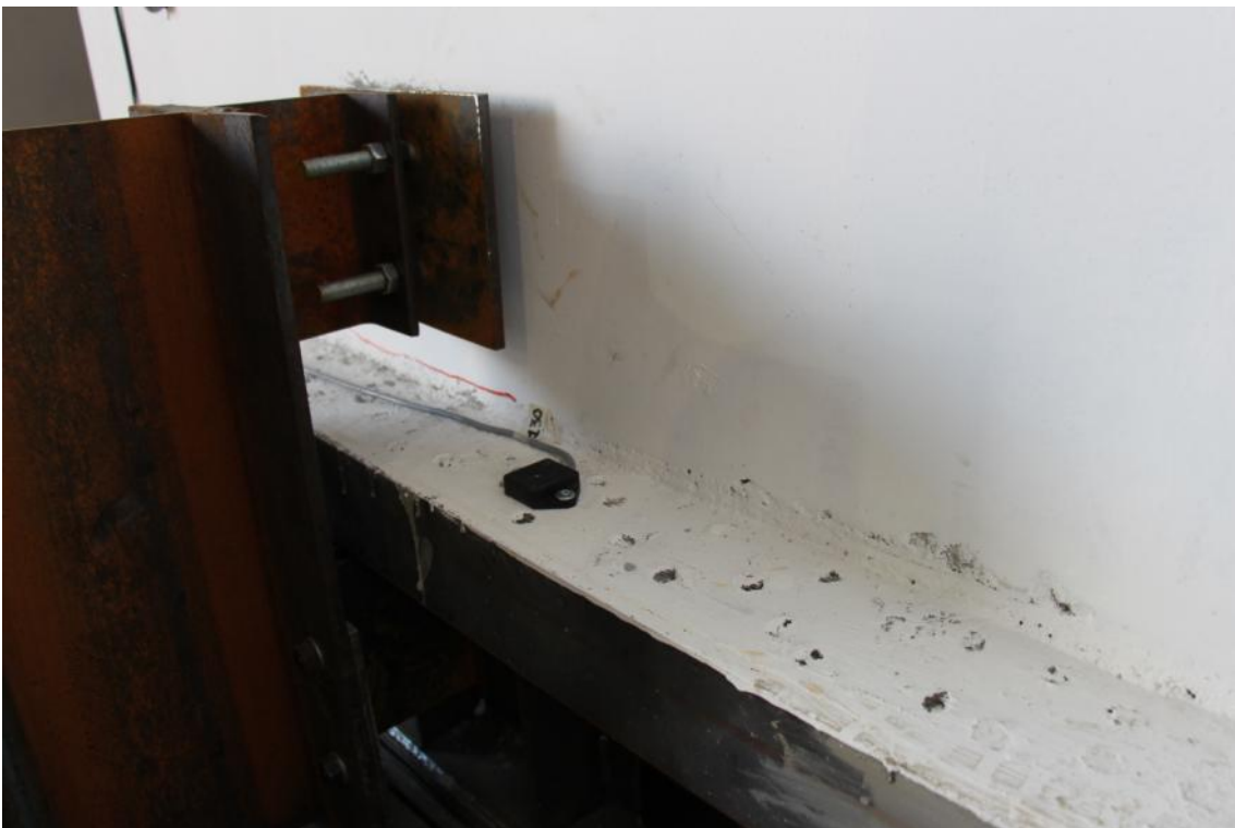
Figure 259. Crack running from the edge to the centre of the first-storey stability wall – Wall base.
