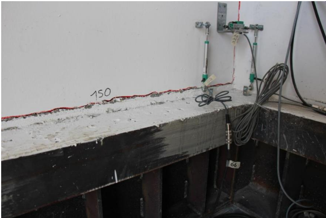
Figure 270. Crack running along the entire depth of the ground-floor stability wall – Wall base.
