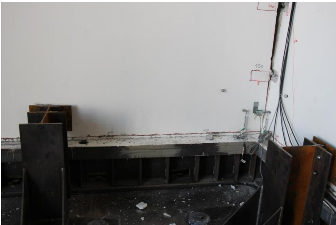
Figure 323. Failure of bottom three-way joints damage pattern at the base of the stability wall.
