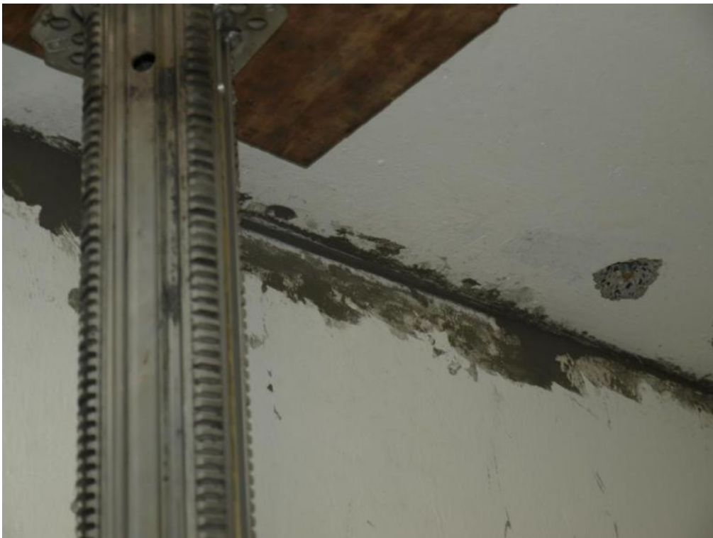
Figure 165. Mortar filling intervention at the first-floor gap – Detail of the South-sided wall edge.
