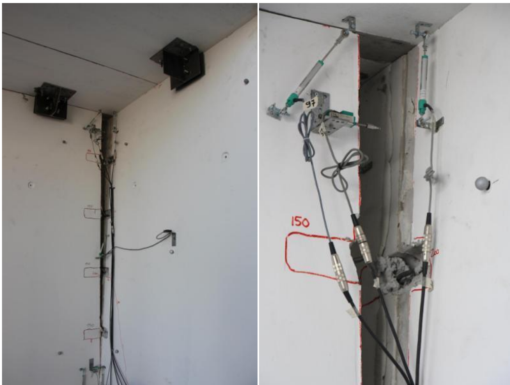
Figure 337. Permanently-bent steel connectors in the top three-way panel joint.
