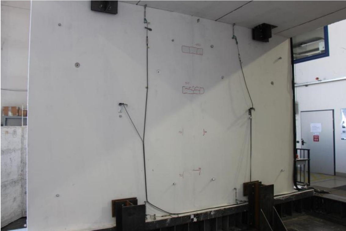
Figure 288. Cracks along the boundaries of the connectors sockets – North-sided ground-floor lateral walls.
