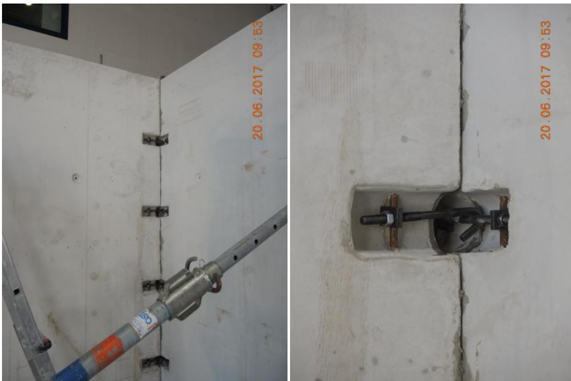
Figure 113. Key details for construction of precast structures of this type – Three-way panel connections.
