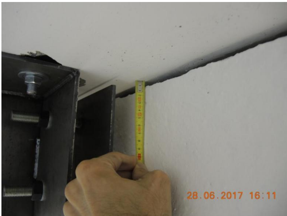
Figure 154. EUC-BUILD5 specimen after construction – Gap between stability wall and slab panel (South edge).
