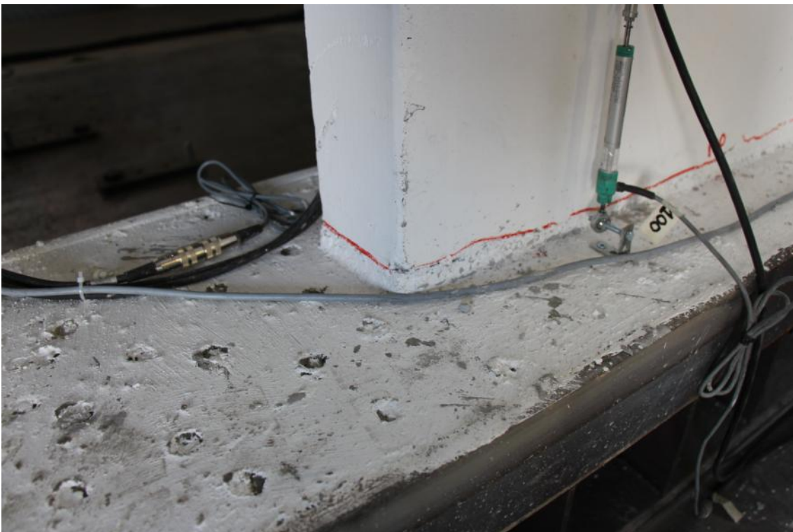
Figure 257. Crack pattern at the base of the first-floor stability wall – Edge of the wall.
