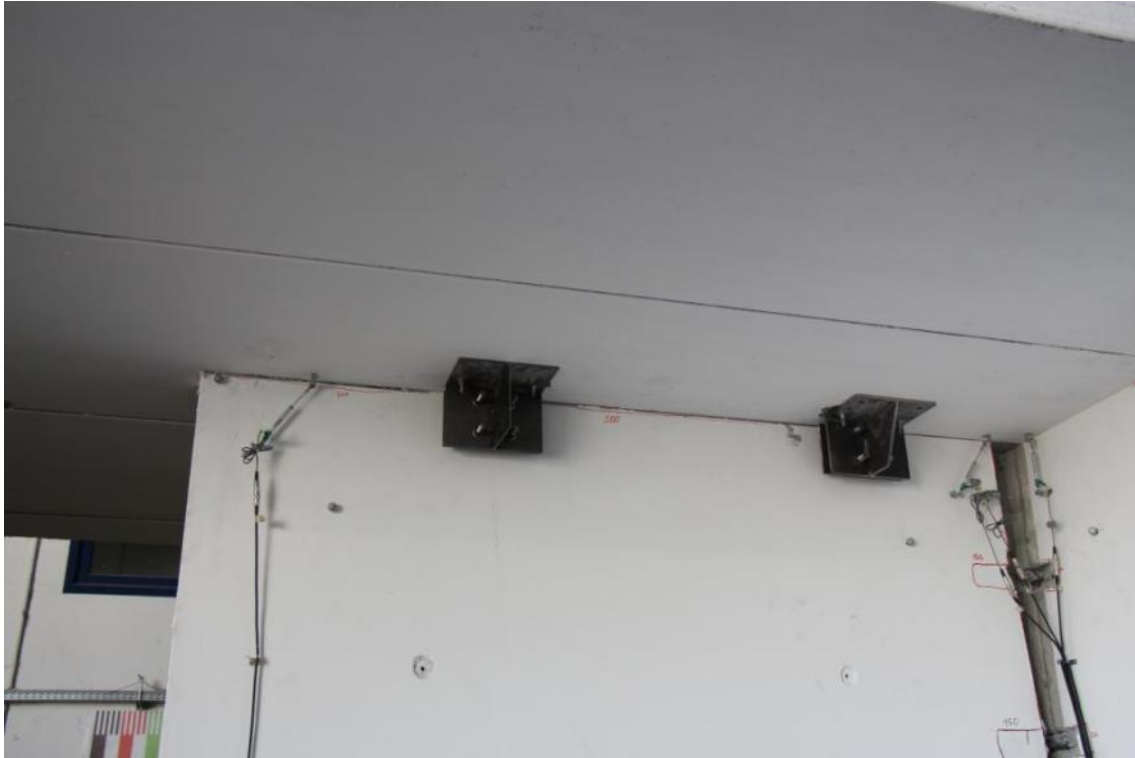
Figure 322. Connection failure and damage pattern in the mortar joint beneath the first-storey slab.
