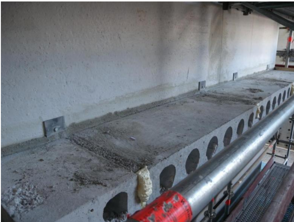
Figure 143. Panel-to-slab steel plate connectors after mortar filling grouting underneath panels – North side.
