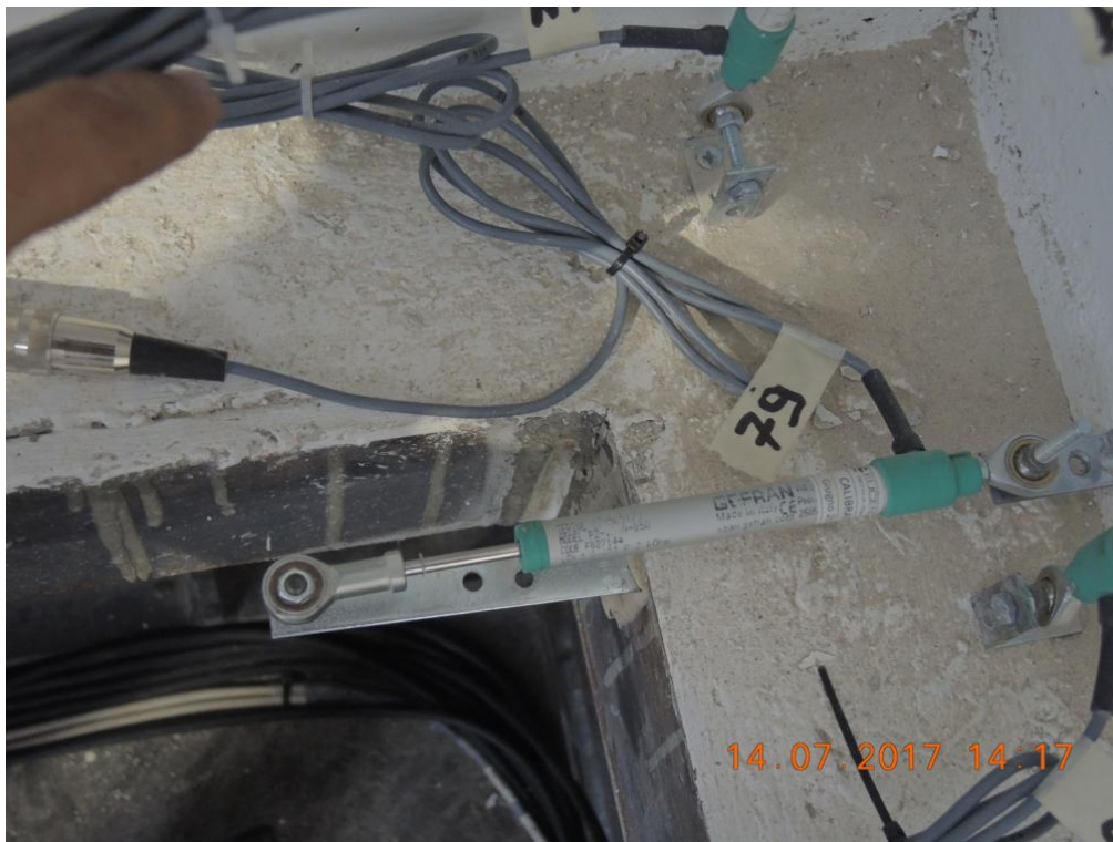
Figure 220. Instrumentation at the base of the first-storey stability and lateral walls.
