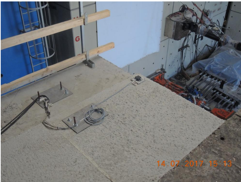
Figure 232. Detail of a 3D accelerometer installed on the second floor slab – South-West side.
