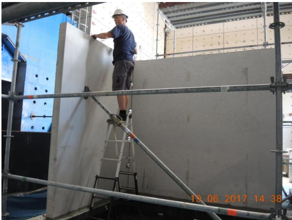
Figure 125. Detail of placing fabric felt layers on top of precast wall panels – South-East-sided lateral wall.
