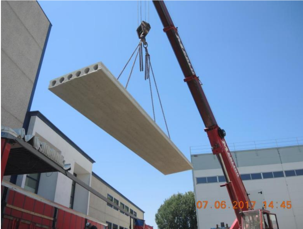
Figure 110. Uplift and transportation of precast slab panels – Detail of a 1200 mm wide panel.
