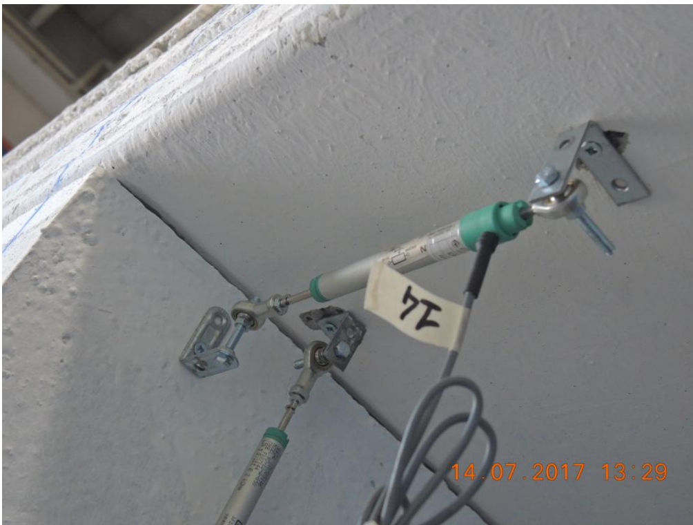
Figure 212. Instrument at the top of the second-storey South-West-sided lateral wall – West corner.
