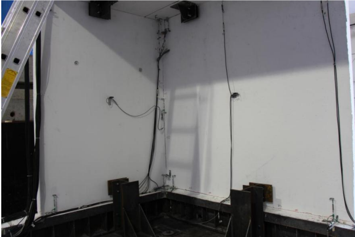
Figure 276. Crack pattern of the ground-floor stability wall – East wall face, base and connectors sockets.
