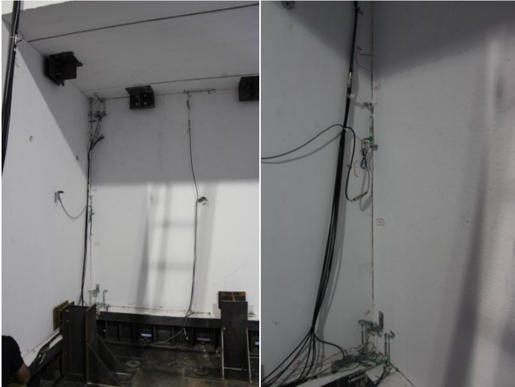
Figure 302. Extensive damage of the top three-way joint – East face of the first-storey stability wall.
