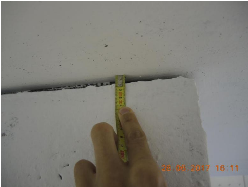
Figure 153. EUC-BUILD5 specimen after construction – Gap between stability wall and slab panel (North edge).
