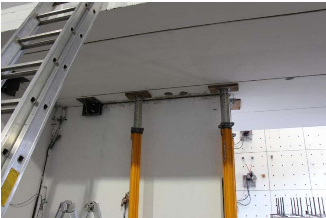
Figure 159. Mortar filling intervention at the first-floor gap – Temporary steel elements for slab panel uplift.
