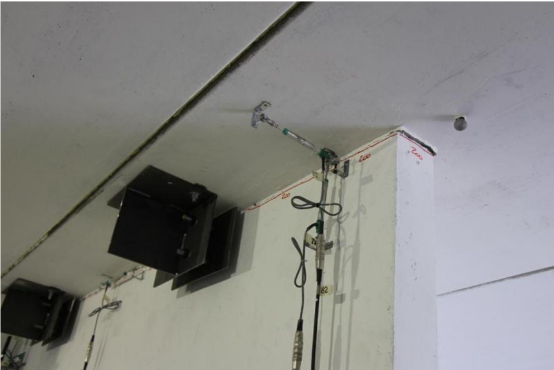
Figure 309. Damage pattern of the mortar joint between the second-storey stability wall and slab.
