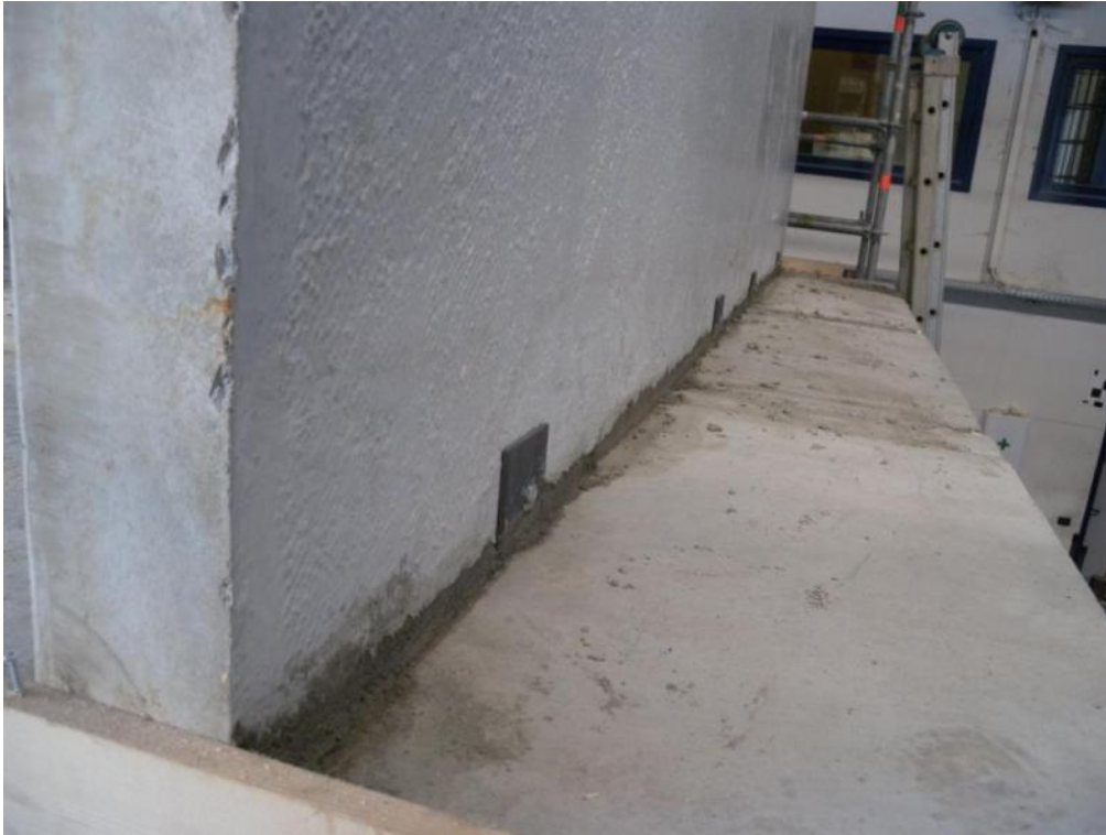
Figure 118. Key details – L-shaped panel-to-slab steel connector, anchoring of short side to wall, first storey.
