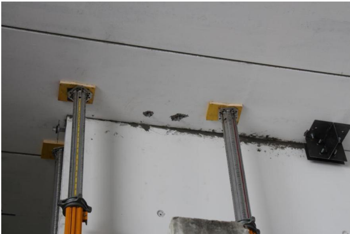
Figure 169. Mortar filling at the second-floor gap – Overall view of the West-sided wall face.
