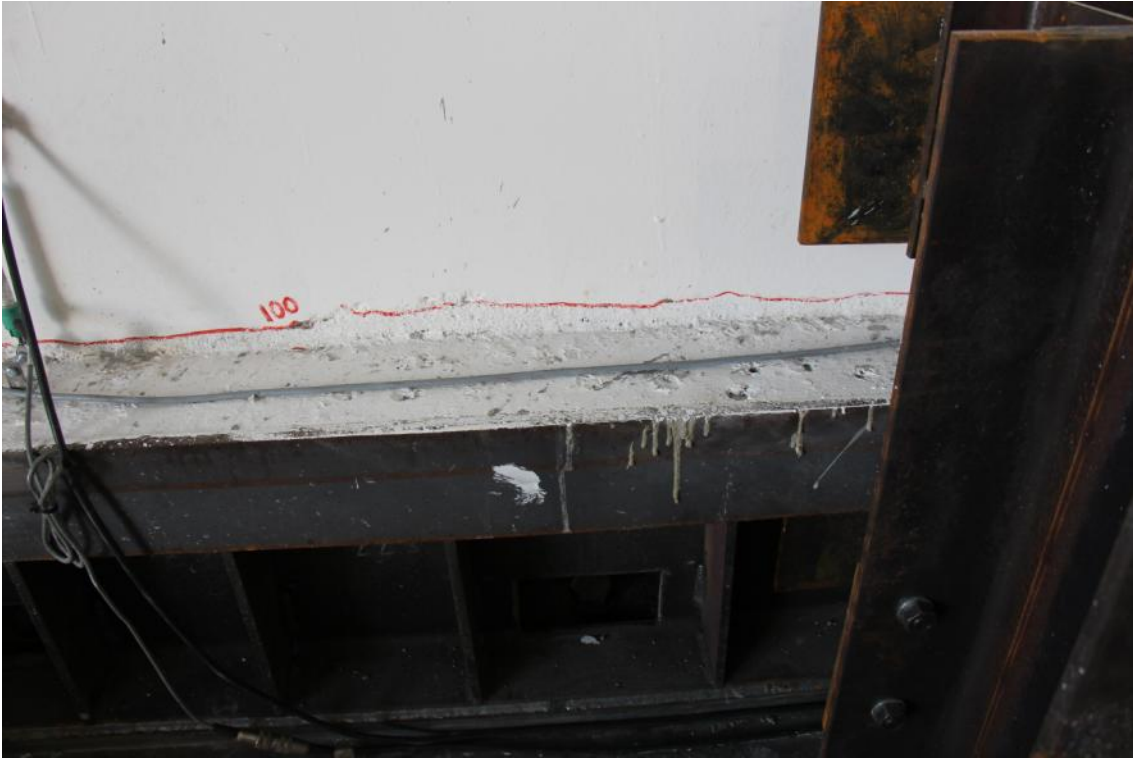
Figure 258. Detail of crack at the base of the first-storey stability wall – Centre of the wall panel.
