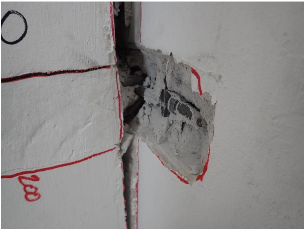
Figure 554. Side view of the bottom three-way connection between stability and lateral walls.
