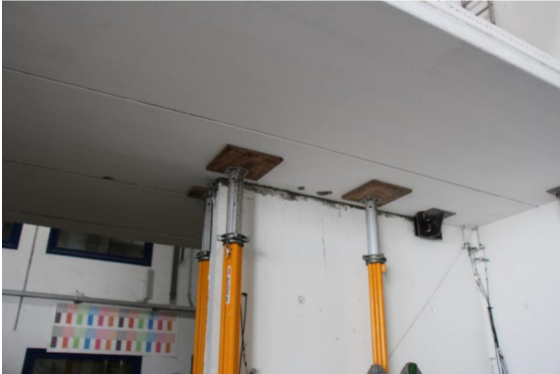
Figure 162. Mortar filling intervention at the first-floor gap – Overall view of the West-sided wall face.
