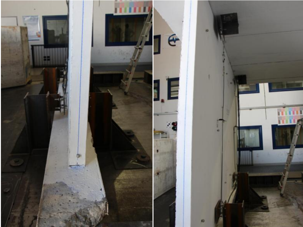
Figure 326. Damage at the base of lateral walls and rocking with loss of verticality – Detail of wall 1L4.
