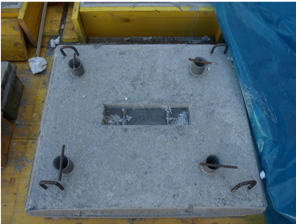
Figure 64. Removal of polystyrene in one horizontal panel and detail of the connector socket.
