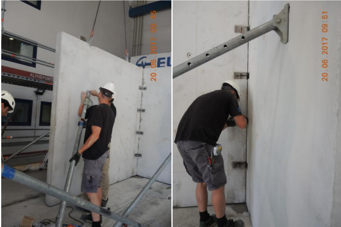
Figure 138. Installation of temporary props on the second-storey stability wall and arrangement of connectors.
