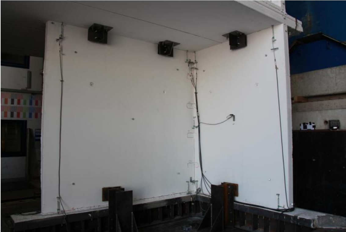
Figure 268. Crack pattern of the ground-floor stability wall – Wall base and connectors sockets.
