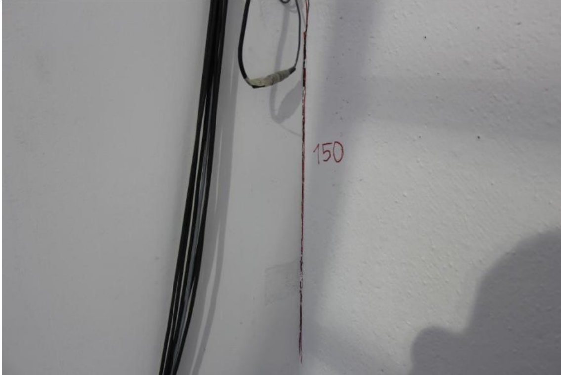
Figure 278. Vertical crack and detachment between stability and transversal walls – East wall face.
