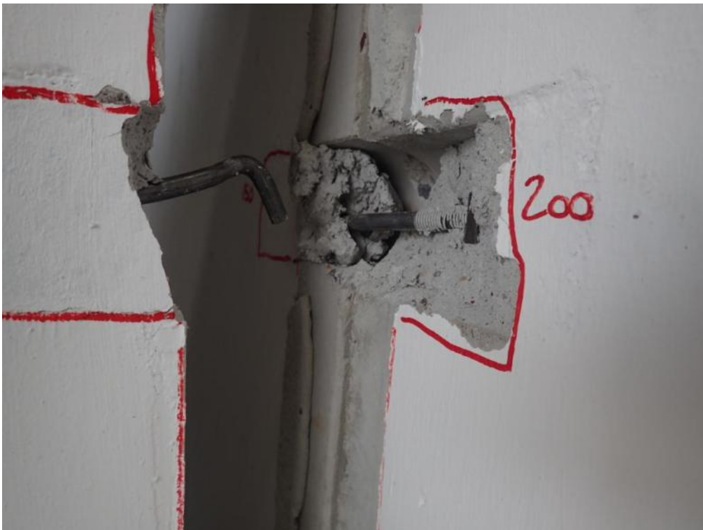
Figure 544. Outwardly-bent and upwardly-bent steel hooks in lateral and stability walls – Top connection.
