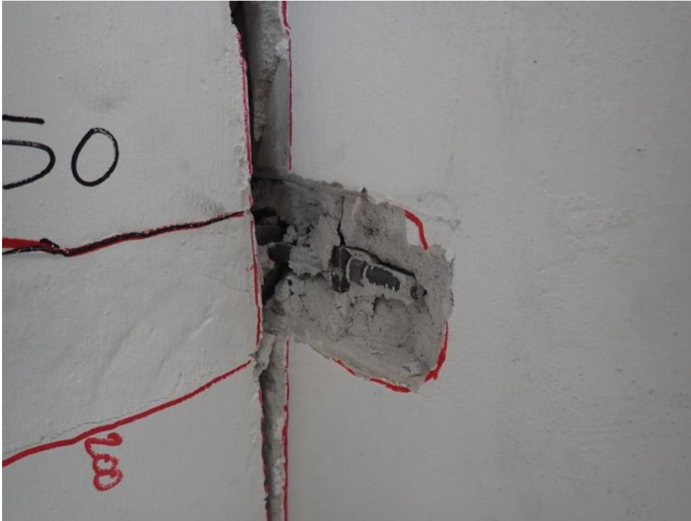
Figure 553. Detailed view of the bottom three-way connection between the stability and lateral walls.
