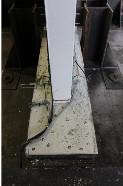
Figure 304. Crack running through the entire width of the first-storey stability wall – Corner, front view.
