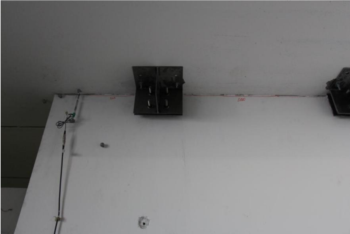
Figure 296. Damage pattern of the mortar joint between the ground-floor stability wall and the slab panel.
