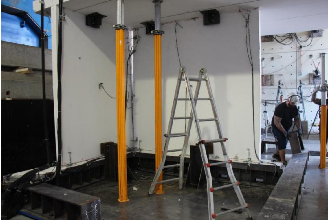
Figure 334. Installation of props in face of the very precarious stability of the structure after the test.
