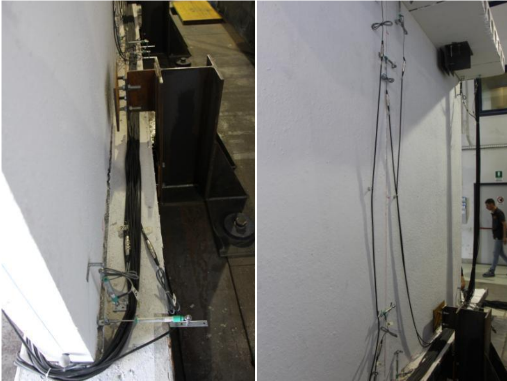
Figure 298. Full-depth/full-width horizontal crack at the base of the first-storey lateral wall 1L2.
