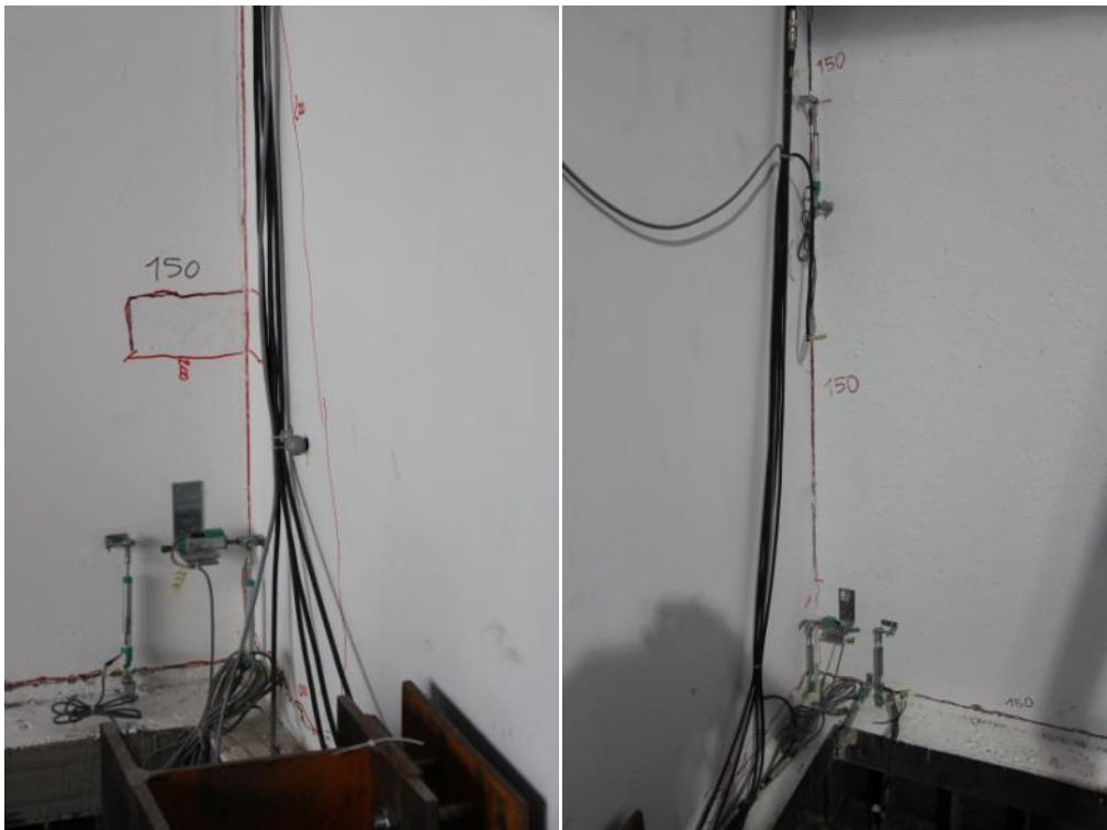
Figure 315. Damage pattern of top and bottom three-way joints at the end of Test run #8.
