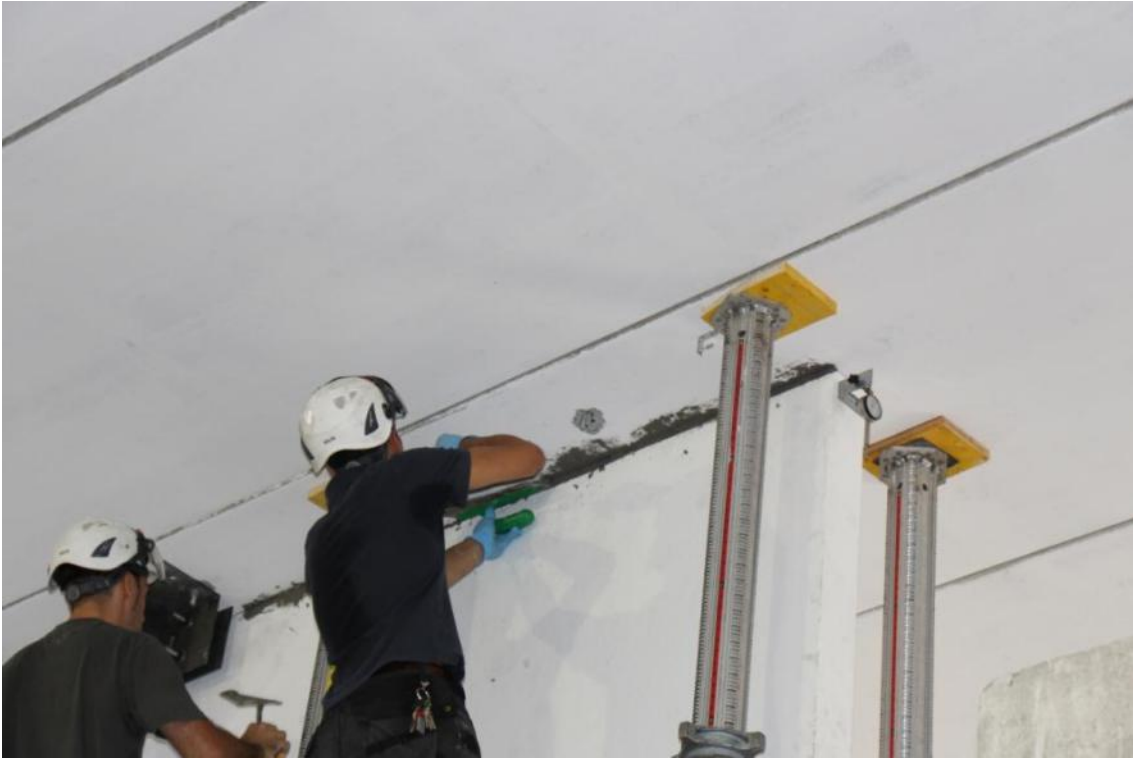
Figure 166. Mortar filling at the second-floor gap – Temporary steel elements for slab panel uplift.
