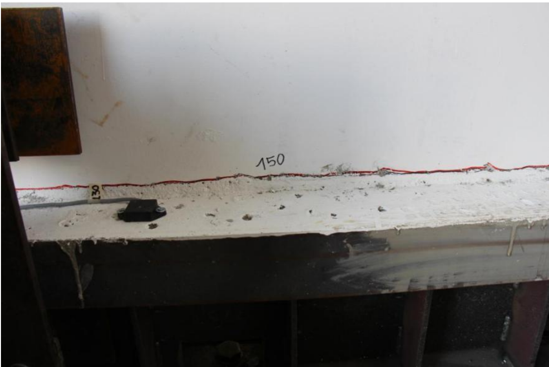
Figure 269. Propagation of horizontal crack along the depth of the ground-floor stability wall – Wall base.
