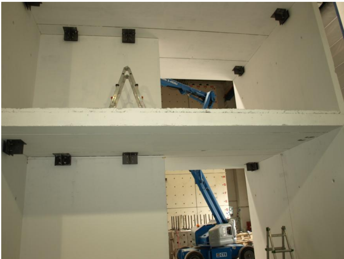
Figure 93. Gap between the stability walls and the slabs.
