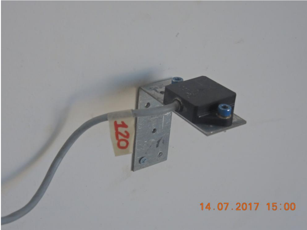
Figure 227. Detail of a 1D accelerometer installed on one of the lateral wall panels.
