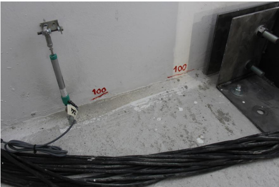
Figure 265. Cracks developed at the base of the second-storey stability wall – West wall face, North edge.
