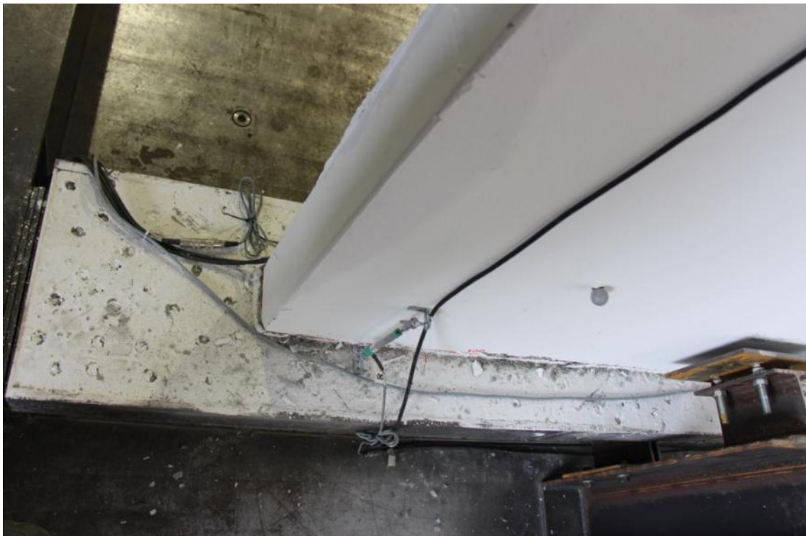
Figure 305. Crack running through the entire width of the first-storey stability wall – Corner, side view.
