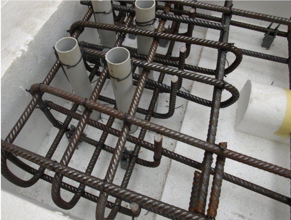
Figure 57. Detail of reinforcing rebars and plastic tubes in one of the wall stripes – Vertical panel.
