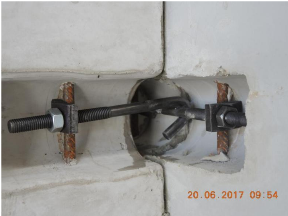
Figure 139. Enlarged view of a three-way connection between stability and lateral walls – Second storey.
