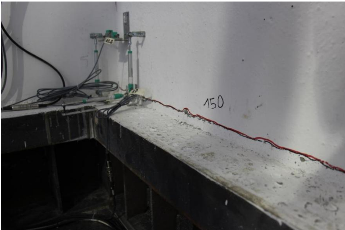
Figure 277. Crack running along the entire depth of the ground-floor stability wall – East wall face, base.
