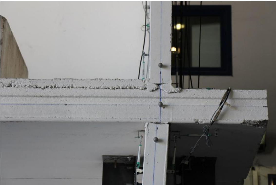
Figure 335. Detail of concrete spalling/crushing at the top of lateral wall 1L2.
