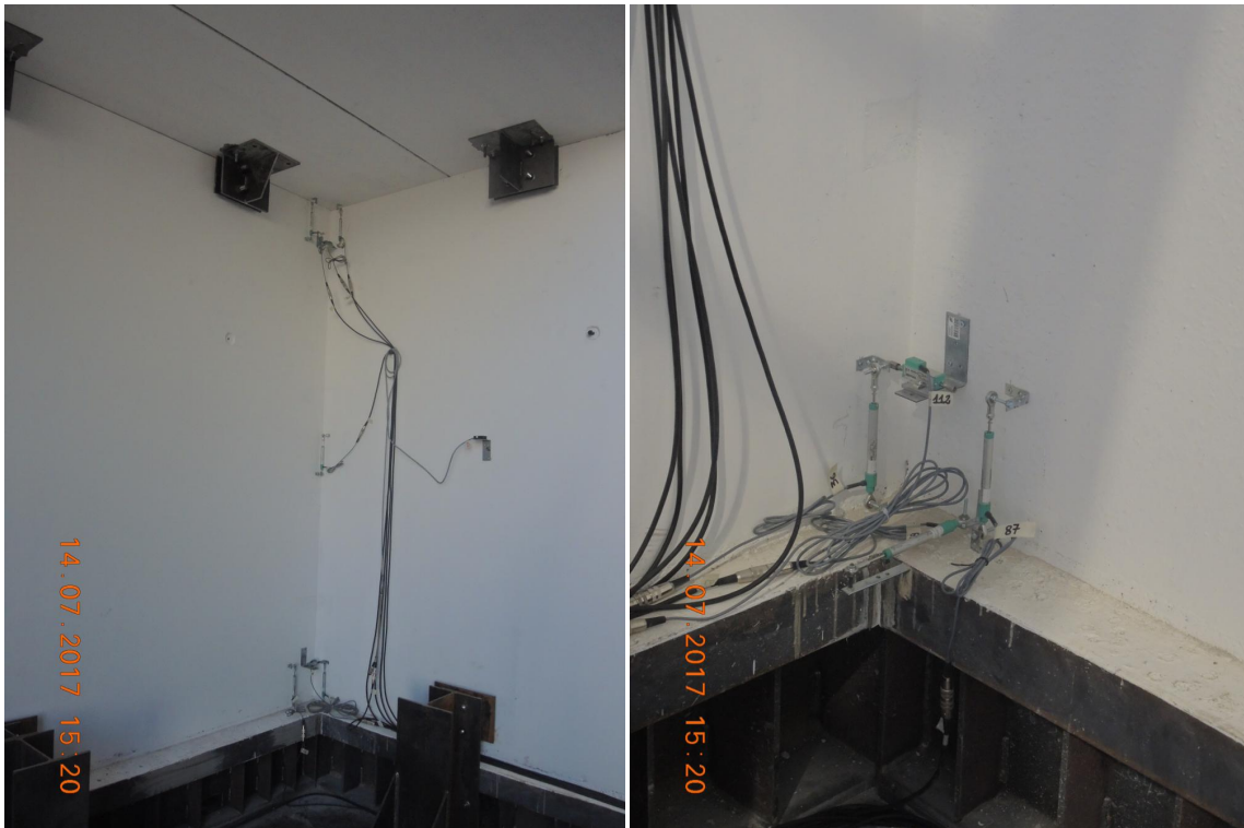
Figure 202. Instruments installed on stability and lateral walls – Global view and detail of the base.
