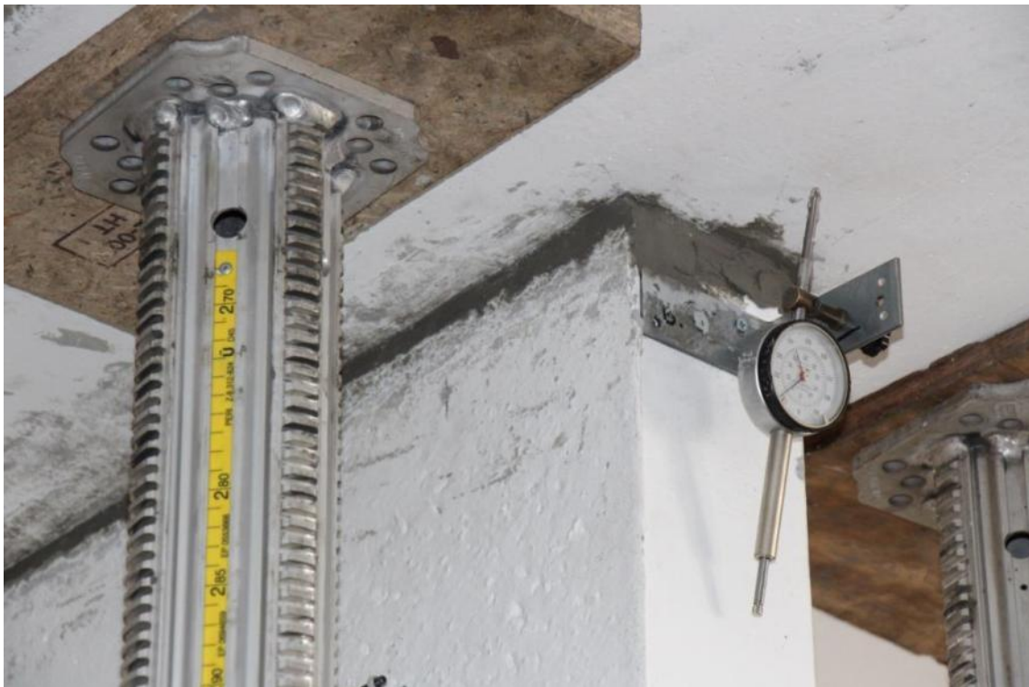
Figure 161. Mortar filling intervention at the first-floor gap – Detailed view of the mortar layer.
