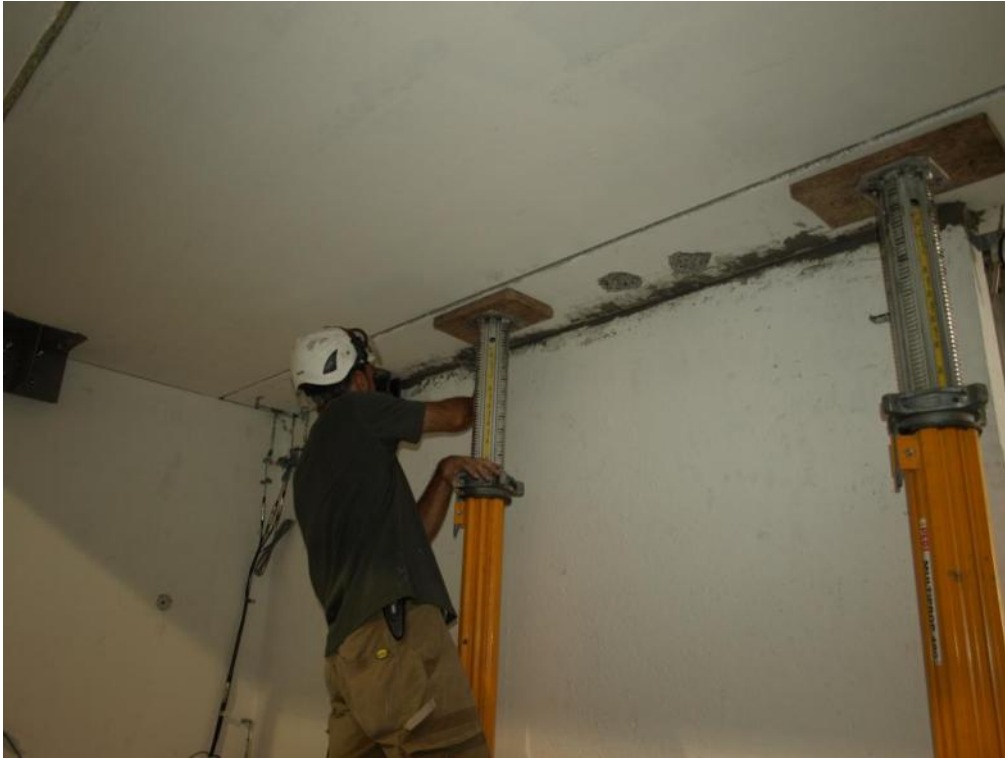
Figure 164. Mortar filling intervention at the first-floor gap – East-sided wall face, South-sided wall edge.
