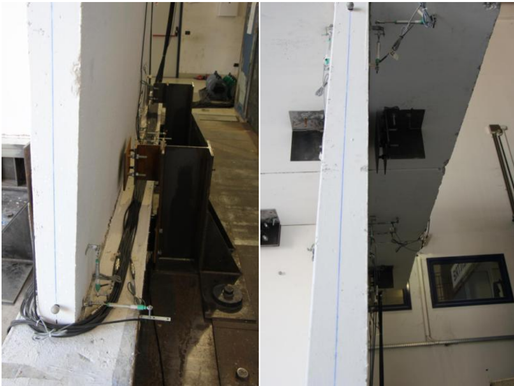
Figure 325. Damage at the base of lateral walls and rocking with loss of verticality – Detail of wall 1L2.
