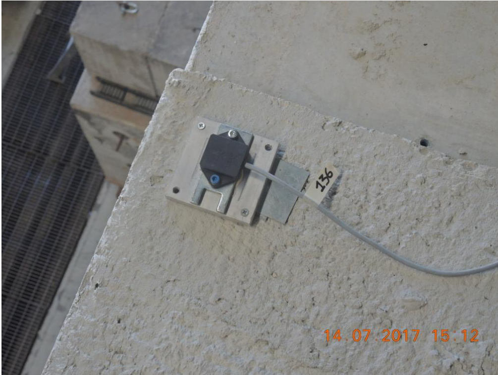
Figure 231. Detail of a 3D accelerometer installed on the second floor slab – North-West side.
