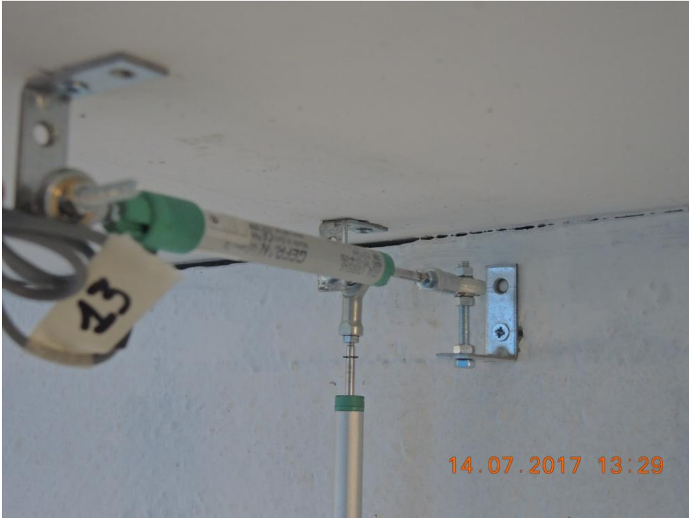
Figure 211. Instrument at the top of the second-storey South-West-sided lateral wall – East corner.
