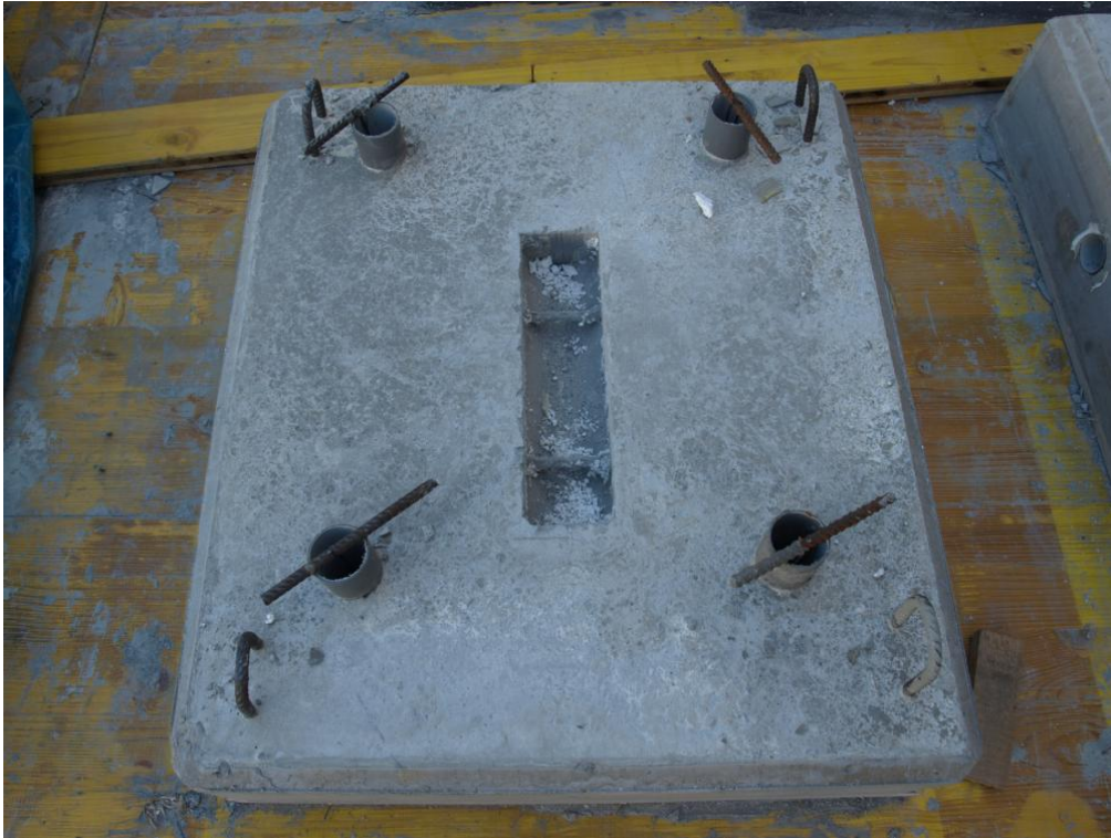
Figure 63. Detail of one horizontal panel after removal of the formworks and polystyrene.
