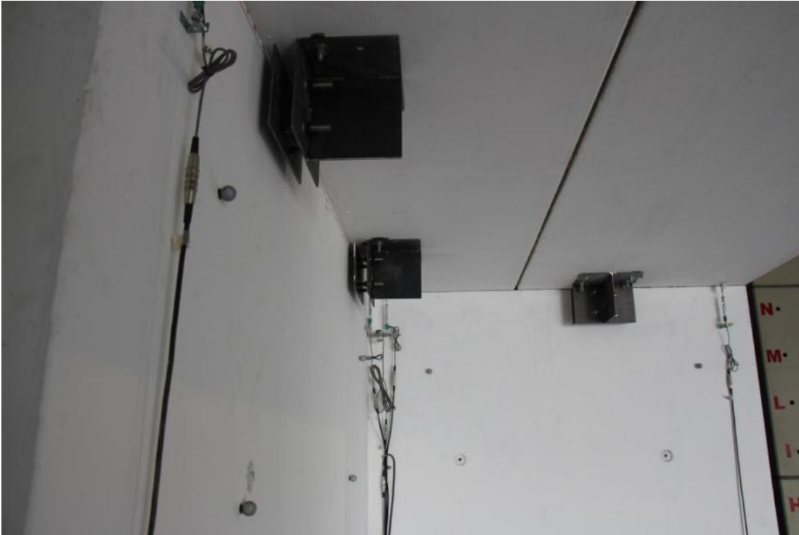
Figure 312. Damage of the mortar joint beneath the second-storey slab and accumulation of displacements.
