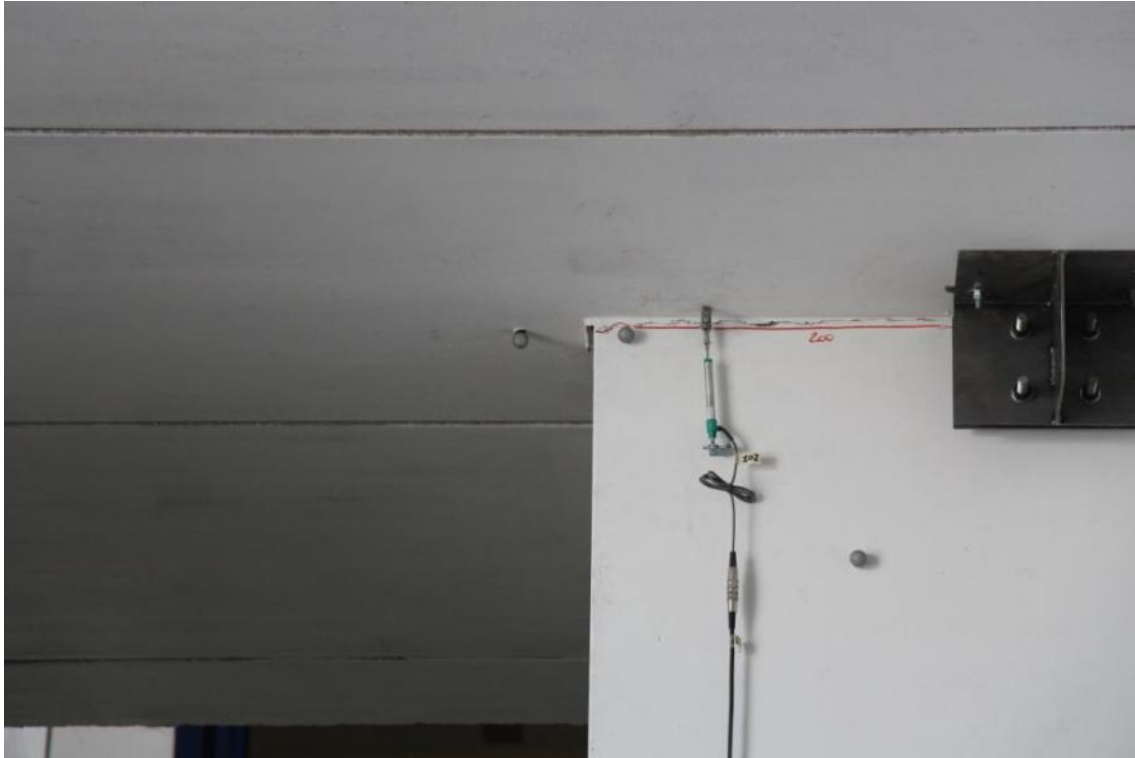
Figure 320. Detail of damage pattern in the mortar joint beneath the second-storey slab – West-side view.
