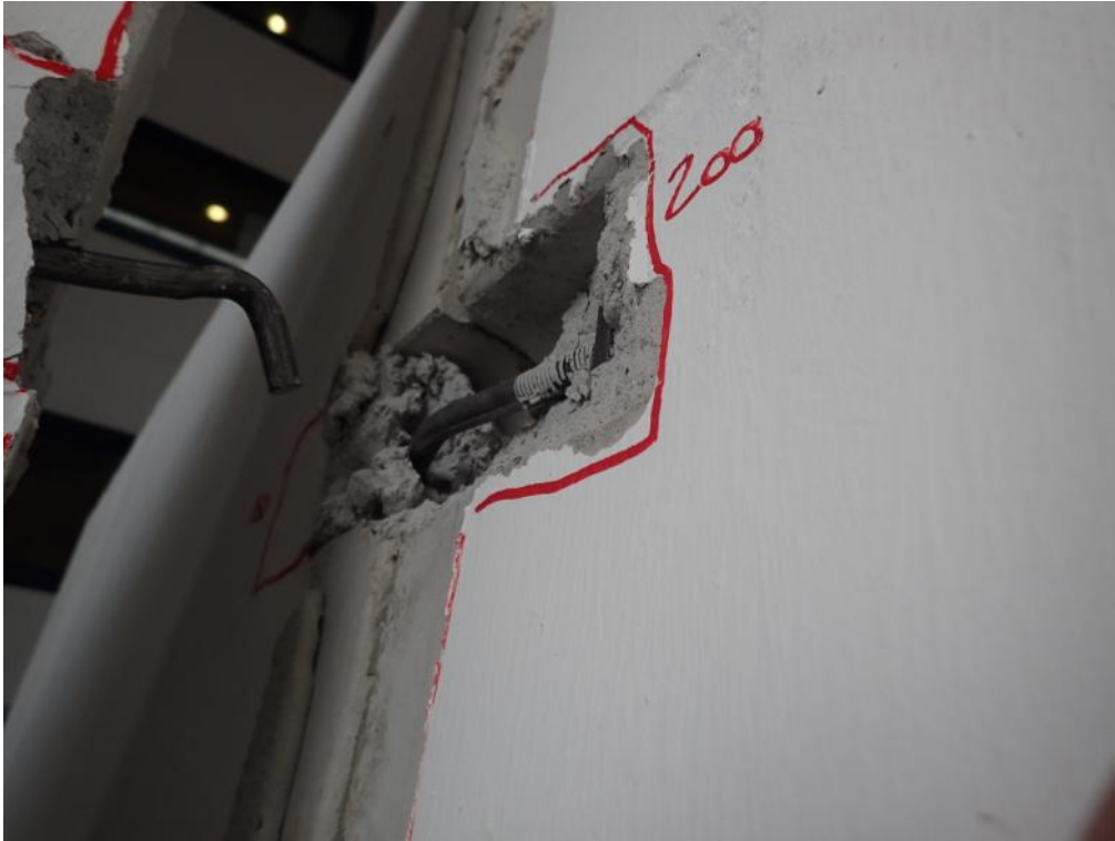
Figure 555. Bottom view of bent steel connectors between lateral and stability walls – Top connection.
