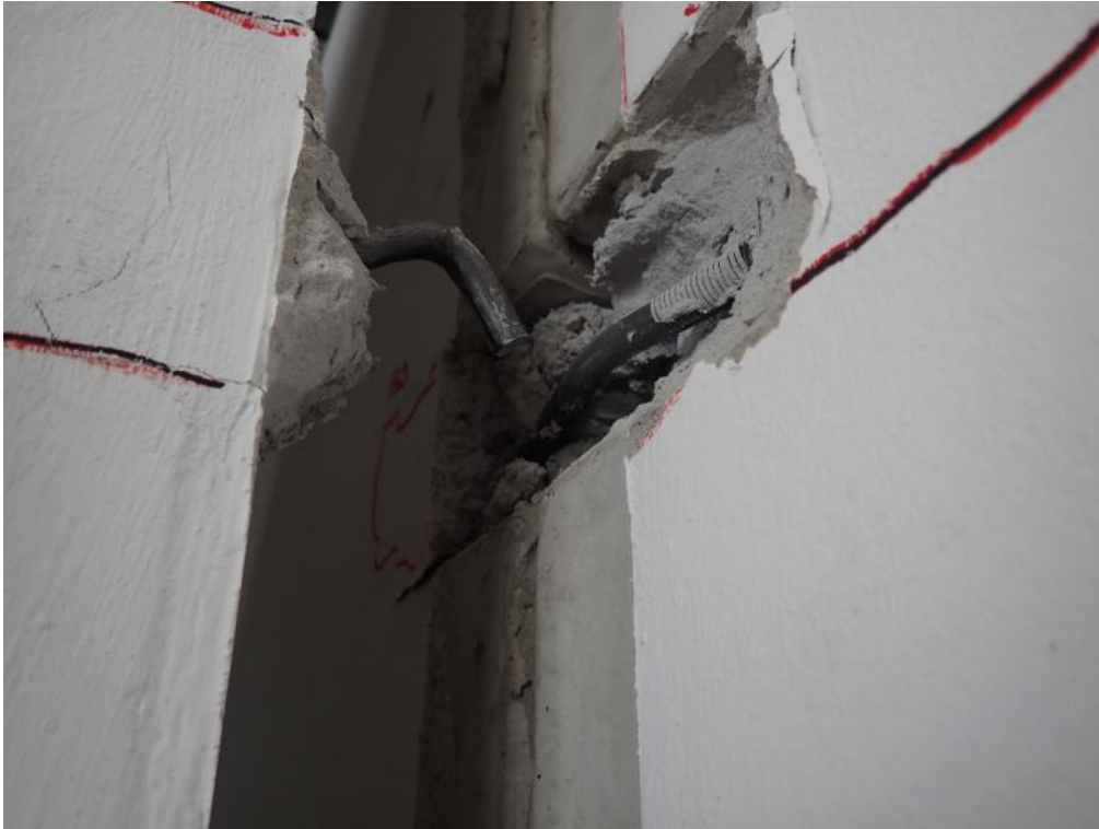
Figure 551. Outwardly-bent and upwardly-bent steel hooks of the second panel joint (from the base).
