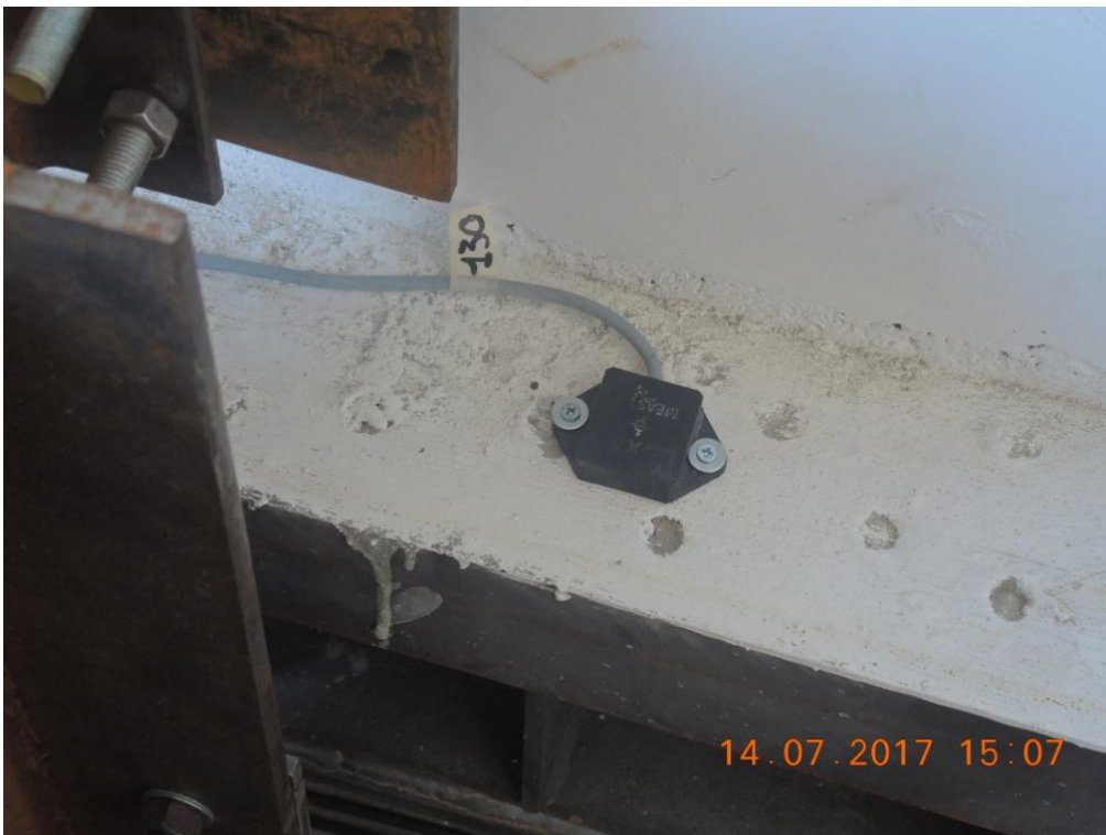
Figure 230. Detail of one of the two 1D accelerometers installed on the foundation of EUC-BUILD5 specimen.
