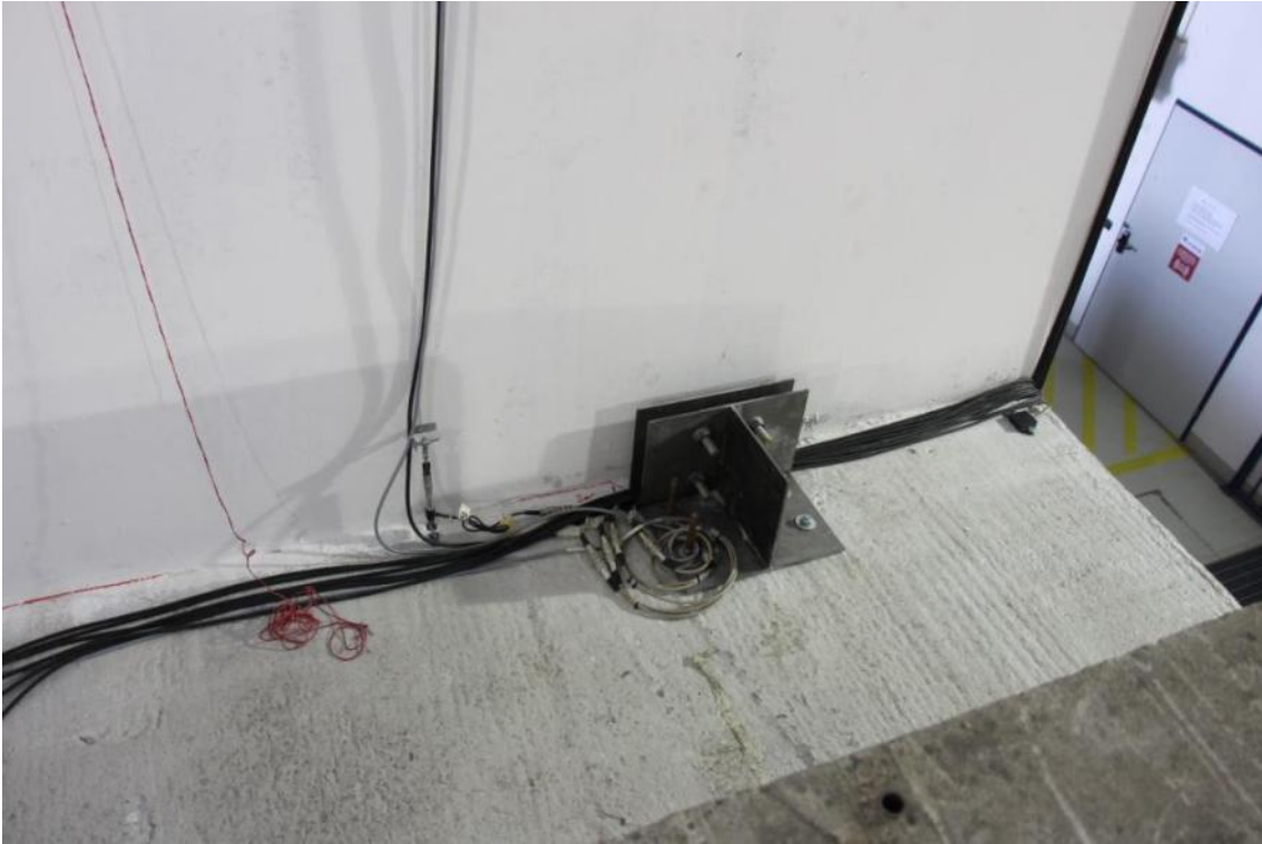
Figure 314. Development of a full-height vertical crack between adjacent lateral walls – North side.
