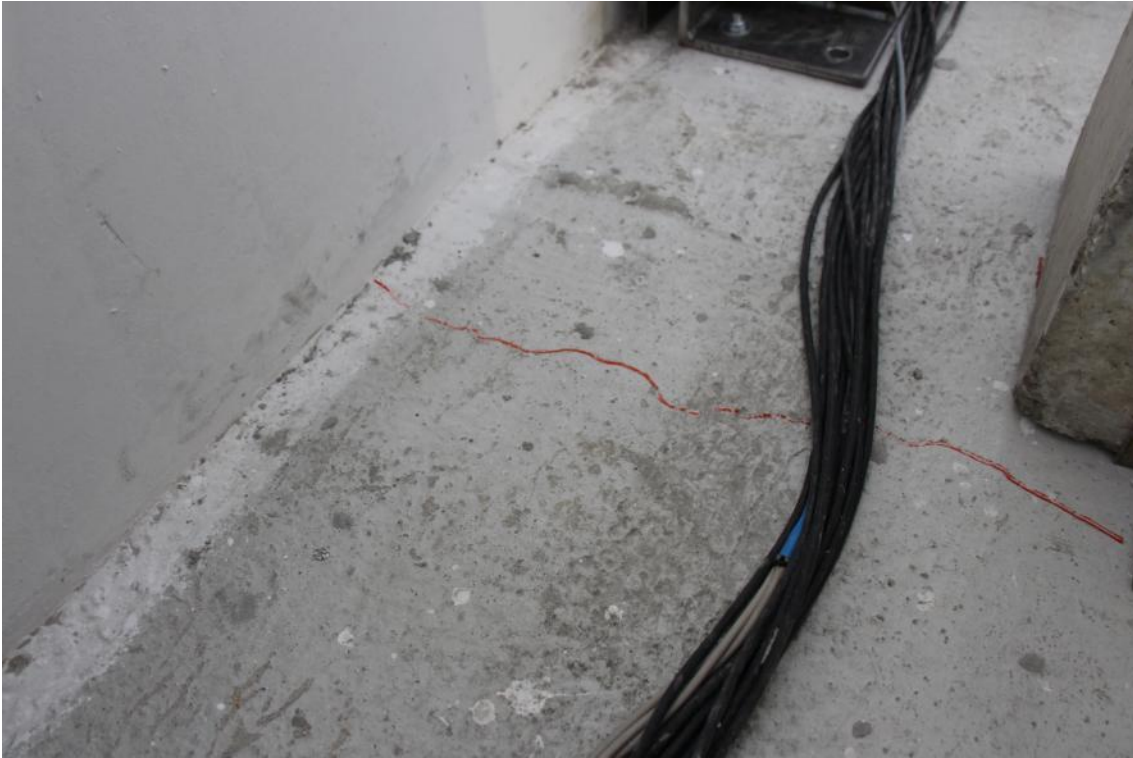
Figure 264. Crack running from the North edge of the second-storey stability wall – West wall face.
