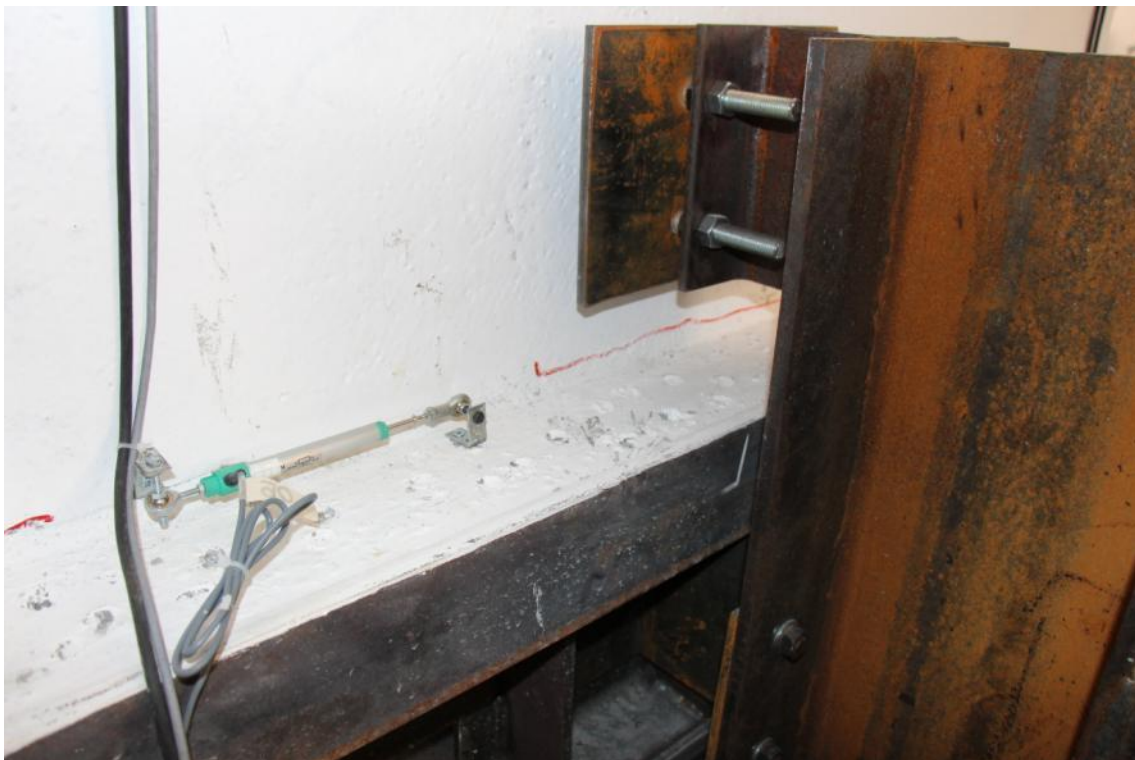
Figure 261. Detail of the crack at the base of the East face of the first-storey stability wall – South side.
