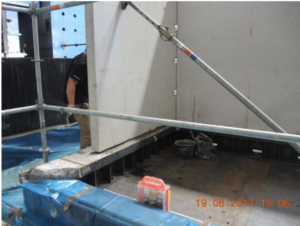
Figure 124. Detail of the first-storey stability and lateral walls installed on the steel foundation.
