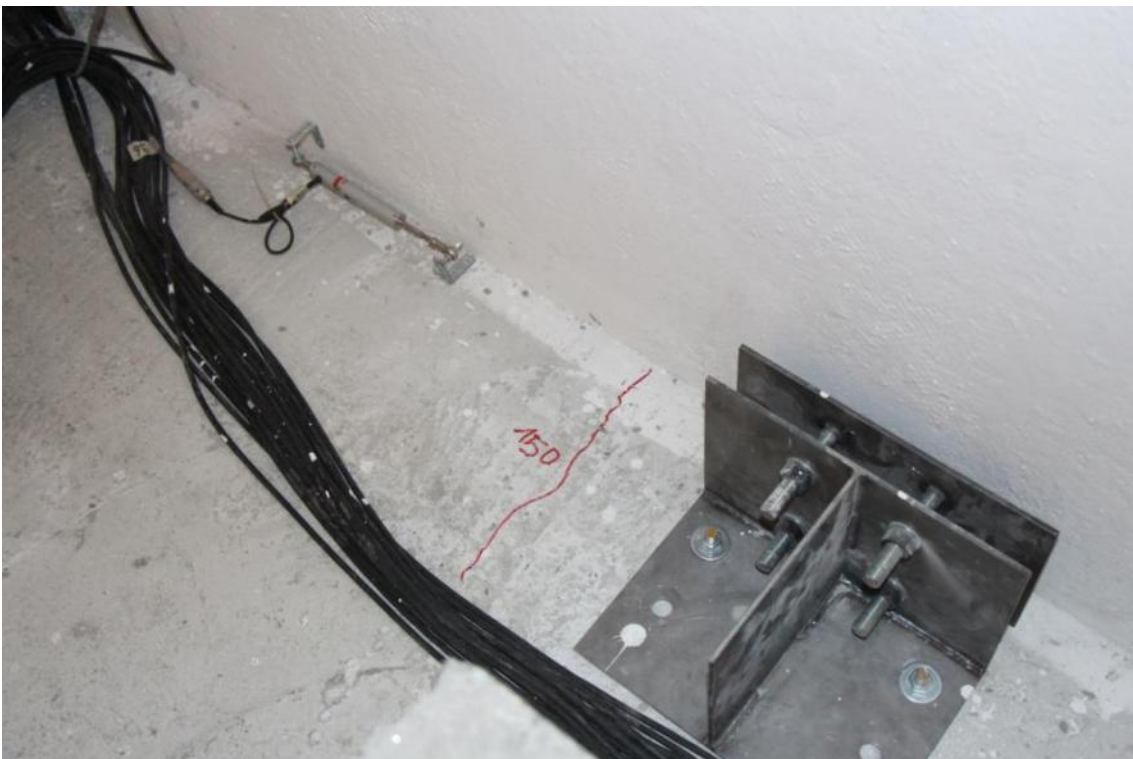
Figure 267. Crack running from the centre of the second-storey stability wall – East wall face.
