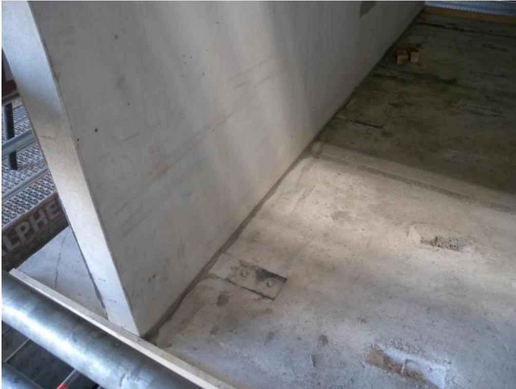
Figure 144. Panel-to-slab steel plate connectors after mortar filling grouting – North side, opposite wall face.
