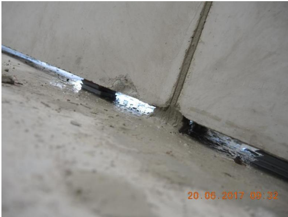
Figure 120. Key details – Installation of spacers underneath precast wall panels for grouting of mortar layer.
