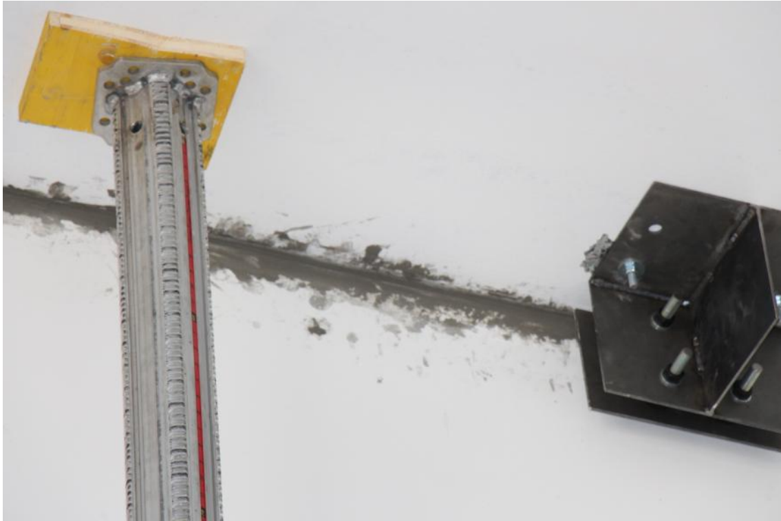
Figure 170. Mortar filling at the second-floor gap – Detailed view of the West-sided wall face.
