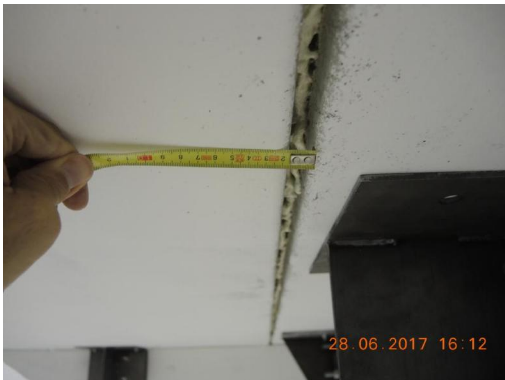
Figure 156. EUC-BUILD5 specimen after construction – Gap between slab panels.
