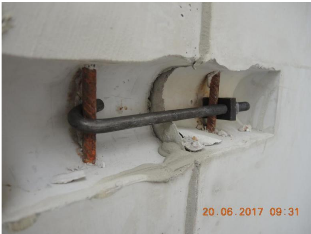
Figure 131. View of a two-way connection between the transversal walls of the specimen – Second storey.
