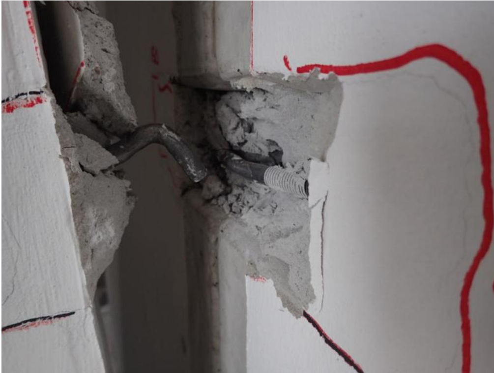
Figure 547. Enlarged view of steel hooks in lateral and stability walls – Third panel joint from the base.
