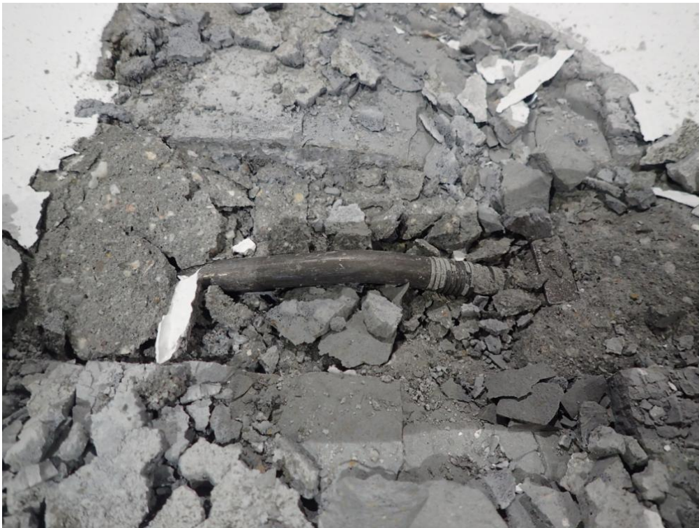
Figure 84. Bending of the steel connector in correspondence to the anchoring region of the hook.
