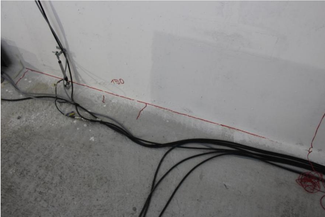
Figure 266. Development of flexural cracks at the base of the North-sided second-storey transversal walls.
