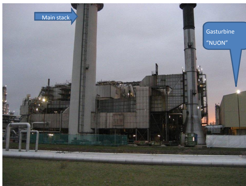
Figure 6.5: Analogue of boiler as would be required to generate 20 bcm/a of flue gas with low oxygen content from the Nuon power plant.
