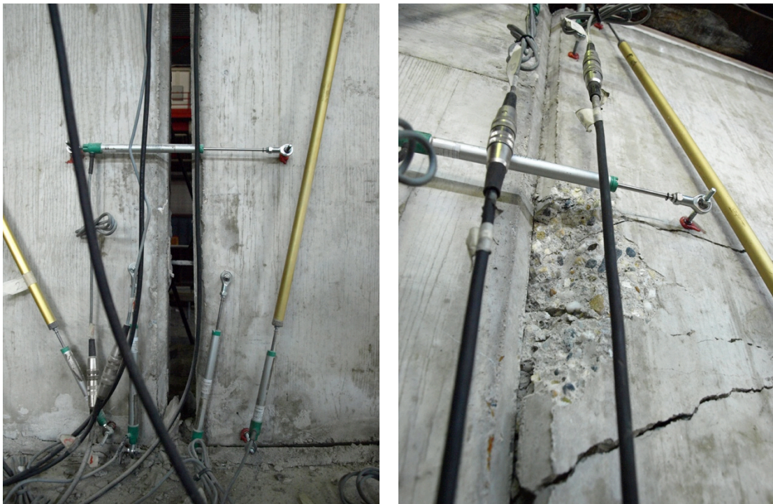
Figure 213: Detaching and pounding at the top and bottom connections – Specimen 08
