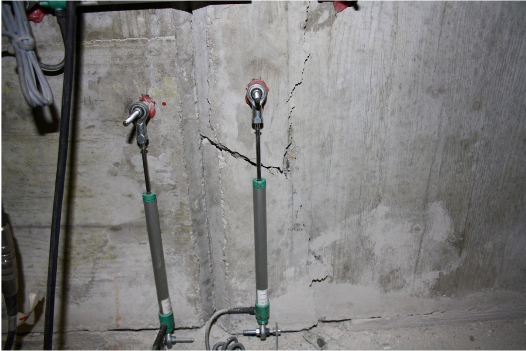
Figure 168: Crack pattern at the base of the wall – Specimen 02
