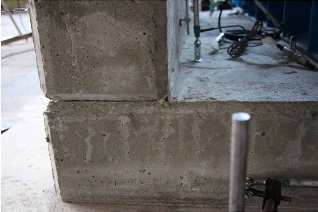
Figure 235: Detail of the crack at the connection level – Specimen 10
