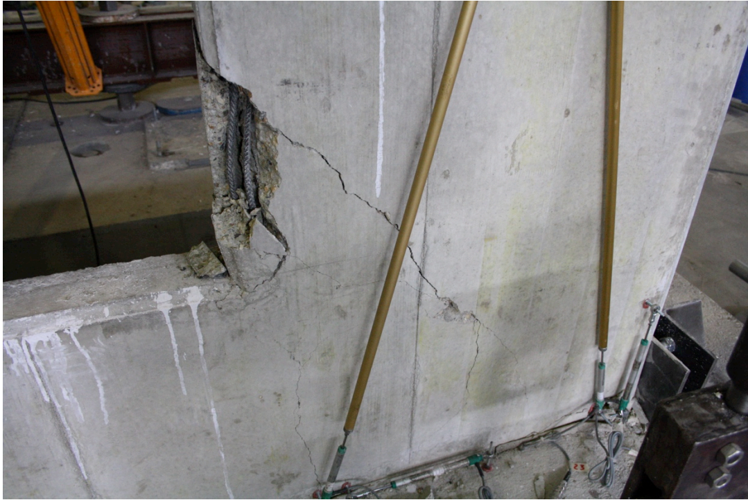
Figure 192: Crack pattern at the corners of the window and buckling of longitudinal bars – Specimen 06
