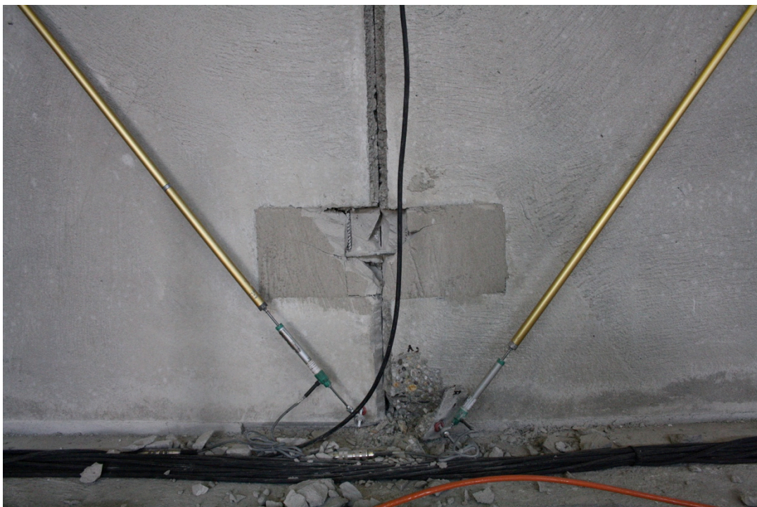
Figure 179: Damage mode at the base steel anchor location – Specimen 04
