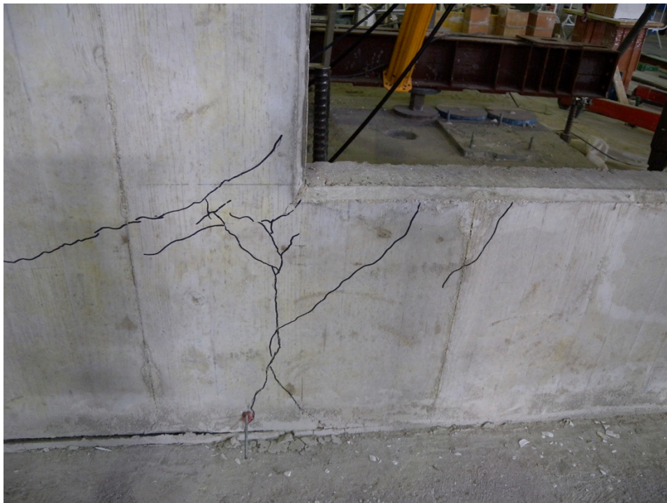
Figure 185: Cracking at the corners of the window in Specimen 05 – detail of the bottom left side
