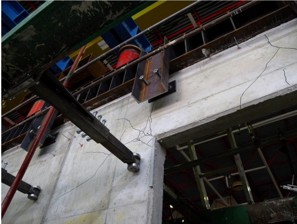
Figure 188: Cracking at the corners of the window in Specimen 05 – detail of the top left side
