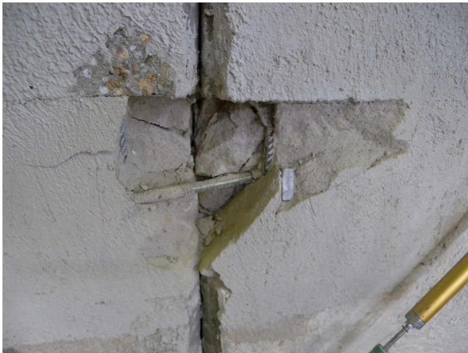
Figure 171: Damage of mortar at the panel anchor location– Specimen 03
