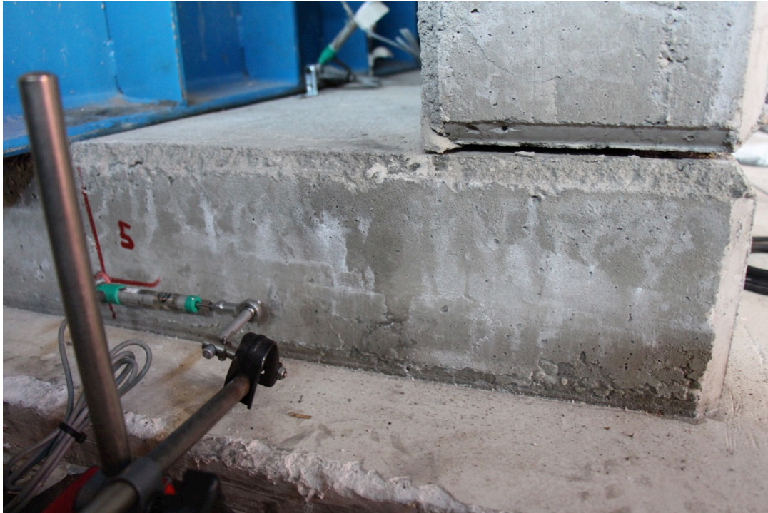
Figure 239: Detail of the crack at the base of panel assembly – Specimen 10
