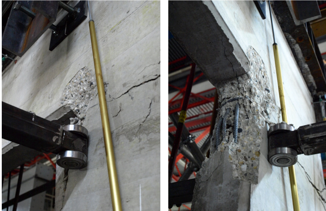
Figure 206: Concrete crushing and buckling of longitudinal bars – Specimen 07
