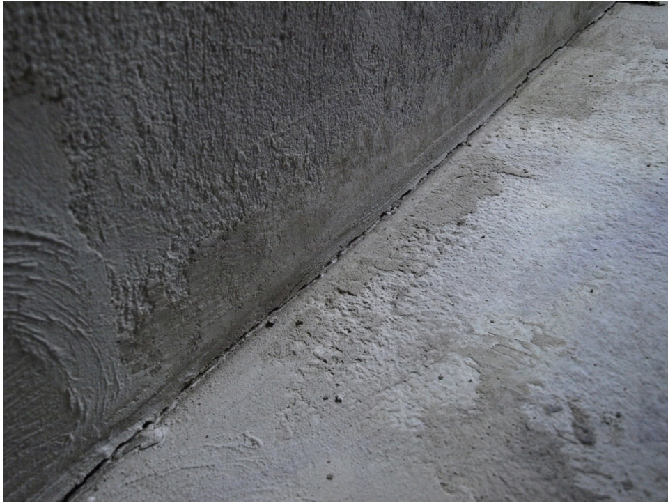
Figure 251: Crack opening at the connection level – propagation along the width of Specimen 12
