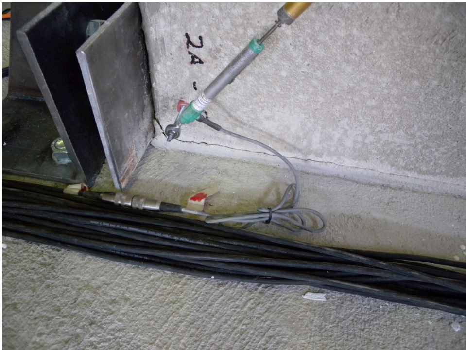
Figure 173: Crack at the corner of the panel due to rocking and base uplift– Specimen 03
