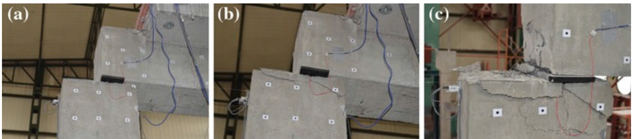
Fig. 25: Damage to the connection of specimen ST-4 (SS column) subjected to Petrovac earthquake in the horizontal direction: (a) after test with PGA = 0.60g; (b) after test with PGA = 0.65g; (c) after repetition of base motion with PGA = 0.65g
