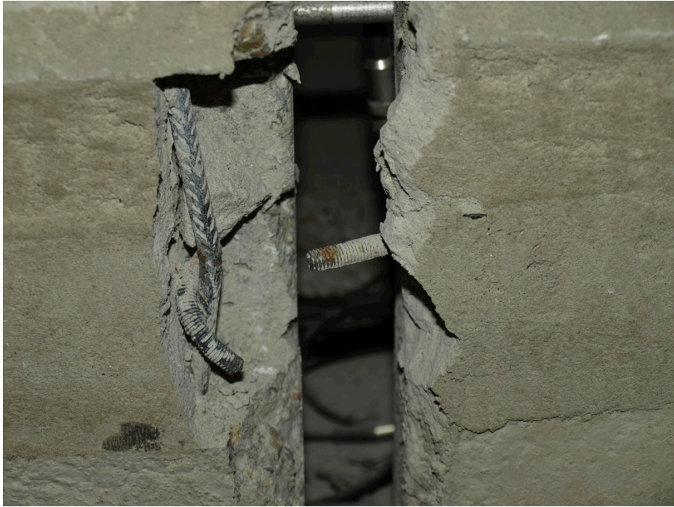
Figure 202: Detail of the anchors failure – Specimen 07
