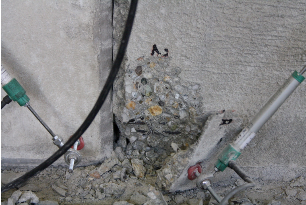
Figure 180: Concrete spalling at the base of the wall – Specimen 04
