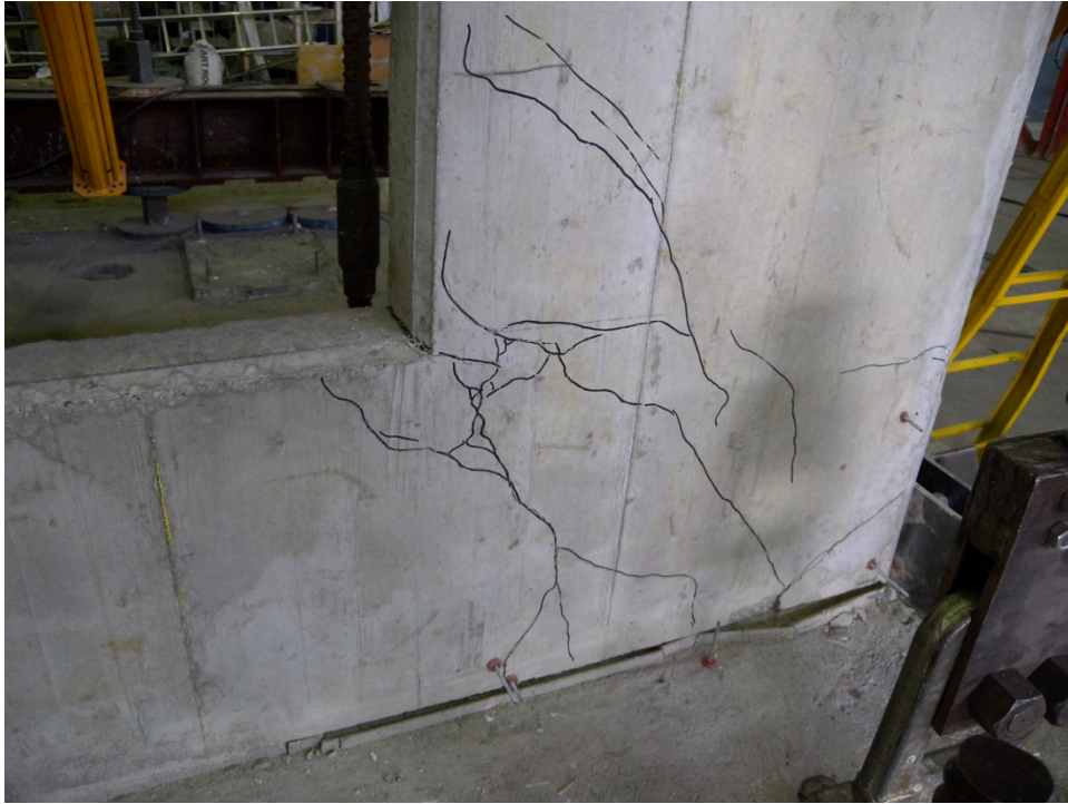
Figure 186: Cracking at the corners of the window in Specimen 05 – detail of the bottom right side
