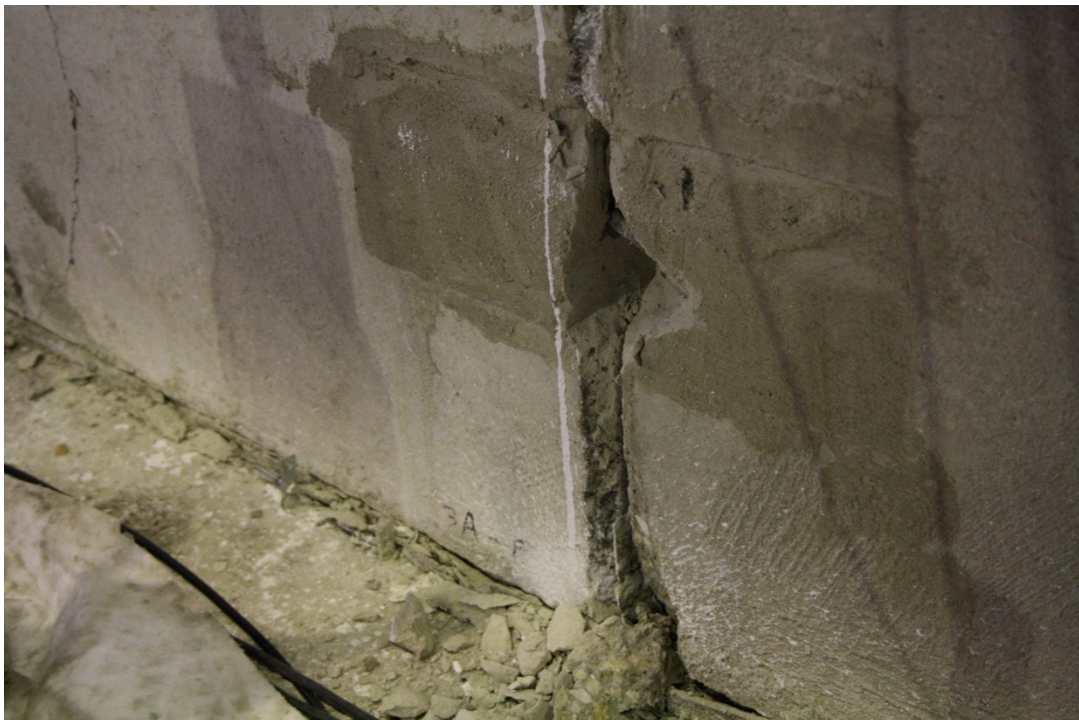
Figure 195: Out-of-plane misalignment and failure of the anchors – Specimen 06
