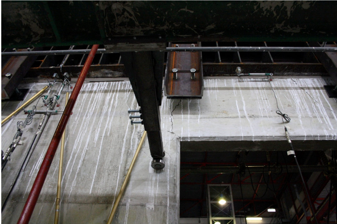
Figure 194: Vertical cracks at the top of the window – Specimen 06
