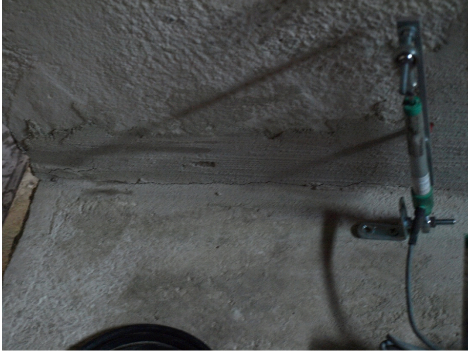
Figure 243: Propagation of the crack along the width of panel assembly – Specimen 11
