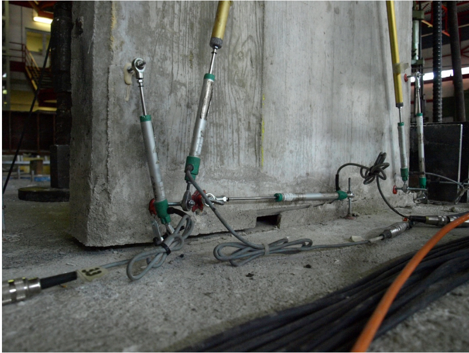
Figure 210: Base uplift in Specimen 08 – detail of the propagation along the entire pier
