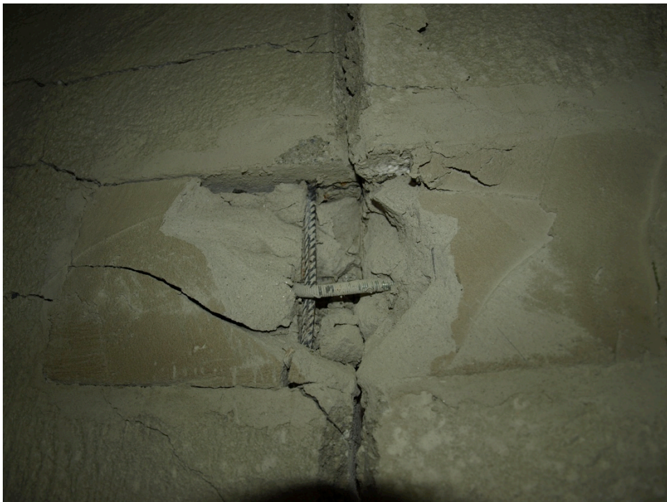
Figure 215: Failure of the anchors – detail of the connection at the top of Specimen 08
