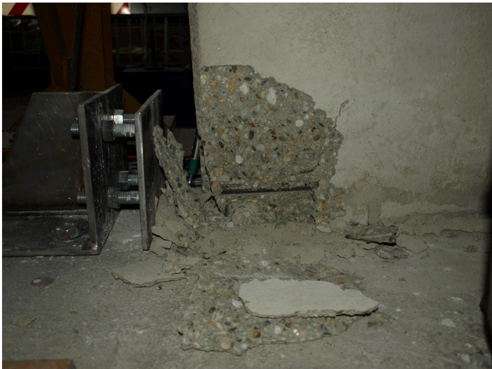
Figure 201: Concrete crushing and spalling at the base of the wall – Specimen 07
