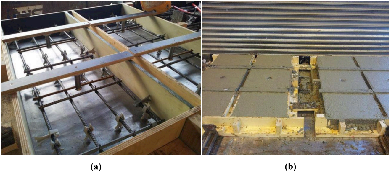
Fig. 28: Panel manufacture at precast yard: (a) Before concrete placement (b) After concrete placement
