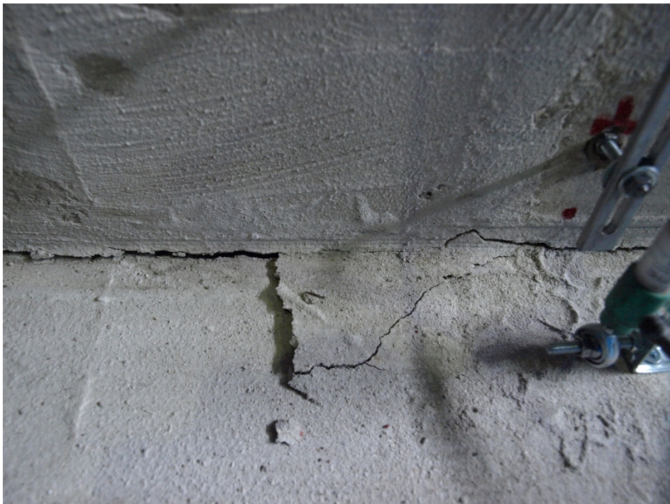
Figure 254: Minor propagation of cracks in the fixed panel of the assembly – Specimen 12
