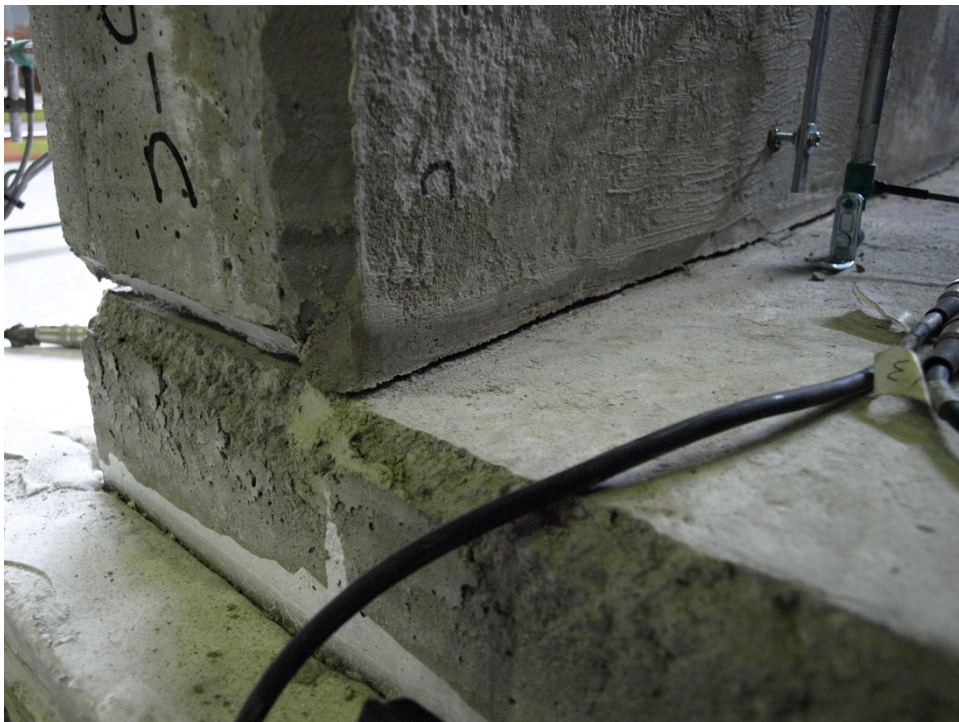
Figure 250: Detail of gap opening and propagation along the width of Specimen 12 – side view
