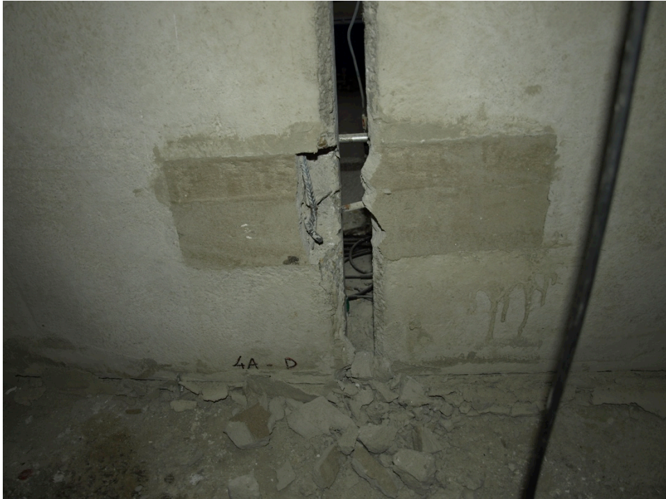
Figure 200: Failure of the anchors and detaching of the two panels – Specimen 07
