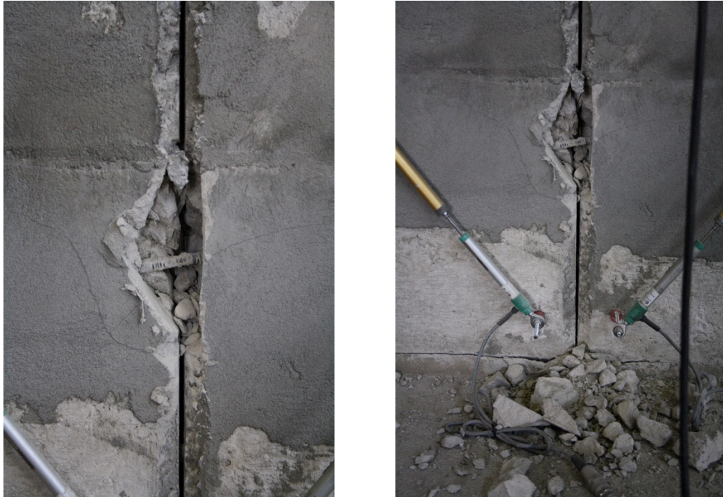
Figure 164: Damage pattern of the connection systems – Specimen 01
