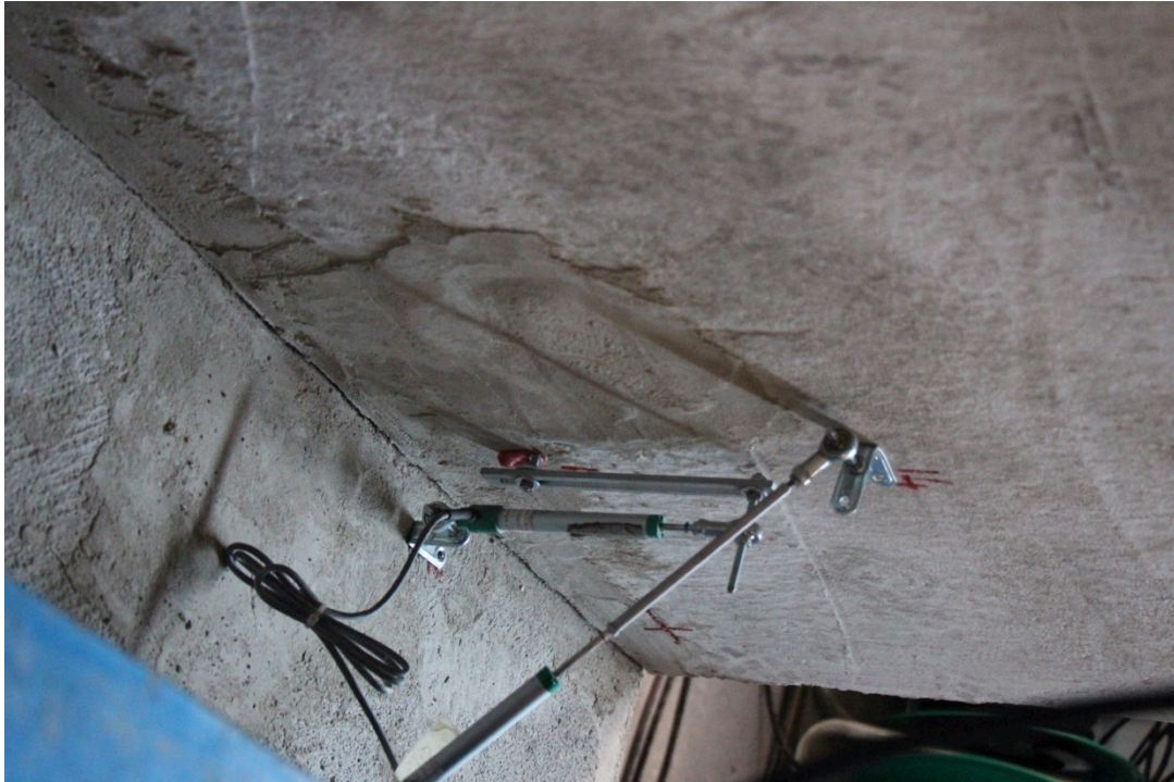
Figure 237: Propagation of the crack in correspondence to the connection – Specimen 10
