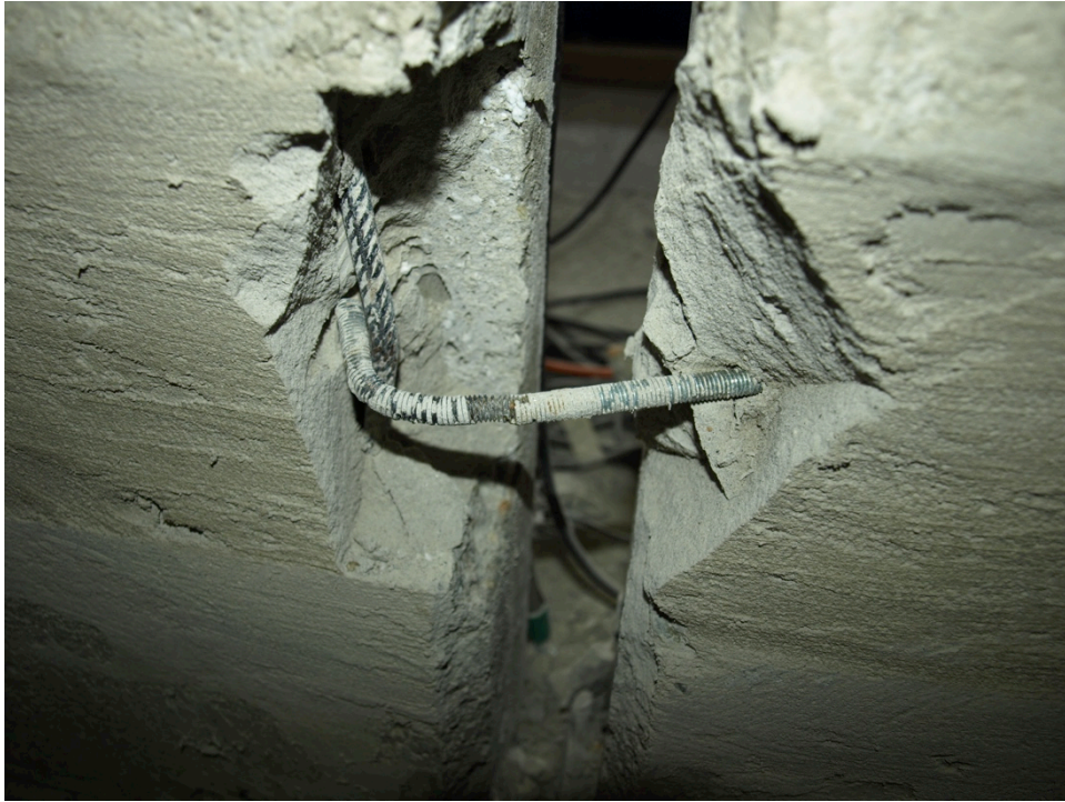
Figure 214: Failure of the anchors – detail of the connection at the bottom of Specimen 08
