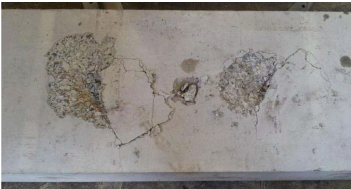
Fig. 31: Localized cracking after monotonic (left) and cyclic loading (right)
