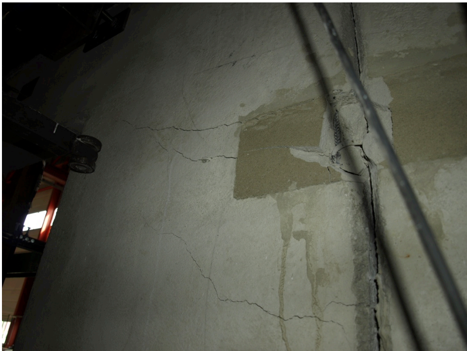
Figure 203: Crack and gap opening at the top connection – Specimen 07
