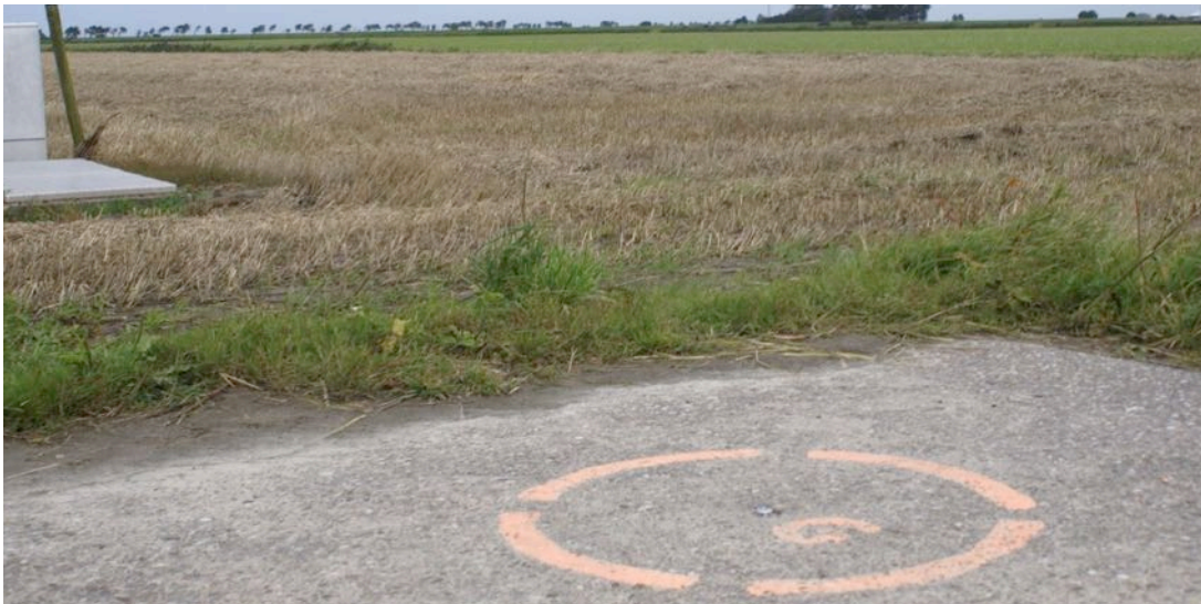
Figure 33: Nail in asphalt with painted red circle around (station 520).
