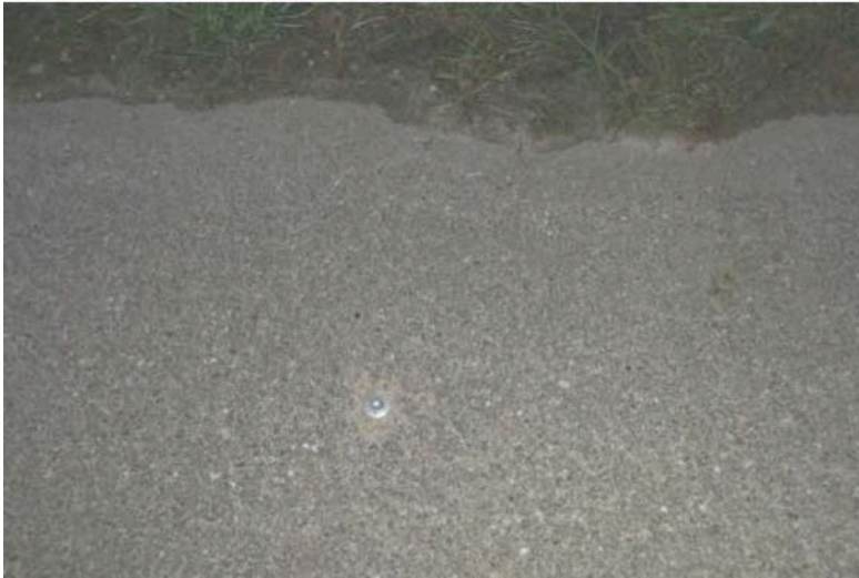
Figure 32: Nail in asphalt, without red painting around (station 521).
