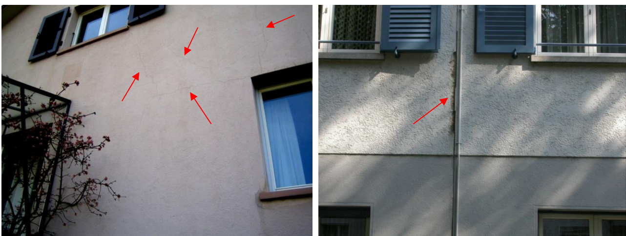
Figure A2.1.33. Hairline cracks in plaster (left). Minor plaster spalling (right).
