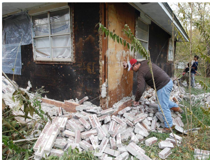
Figure A2.5.24. Façade bricks detached from the wood-frame structure of a house in Sparks
