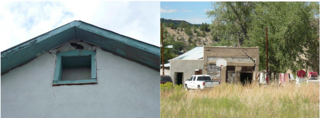
Figure A2.4.20. Major brick damage to a home in Segundo (left) and to a garage in Valdez (right) (Morgan & Morgan, 2011).
