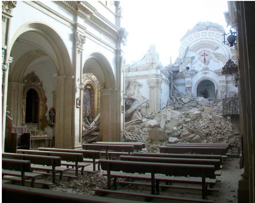
Figure A2.3.37. Collapse of the transept area of the Church of Santiago (Wikipedia).
