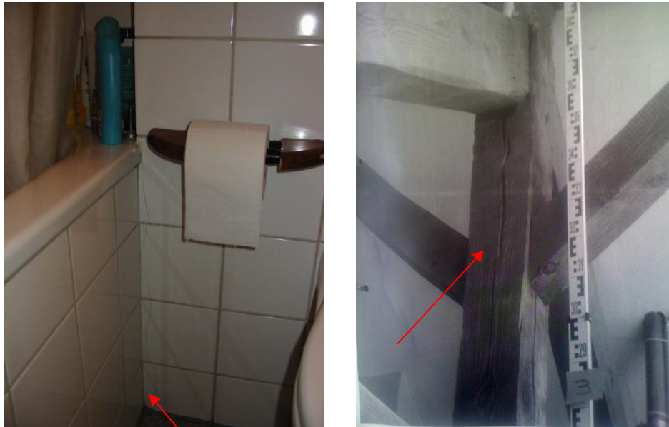
Figure A2.1.34. Crack in intersection of two perpendicular masonry elements (left). Crack parallel to the orientation of fibres in a timber element (right).
