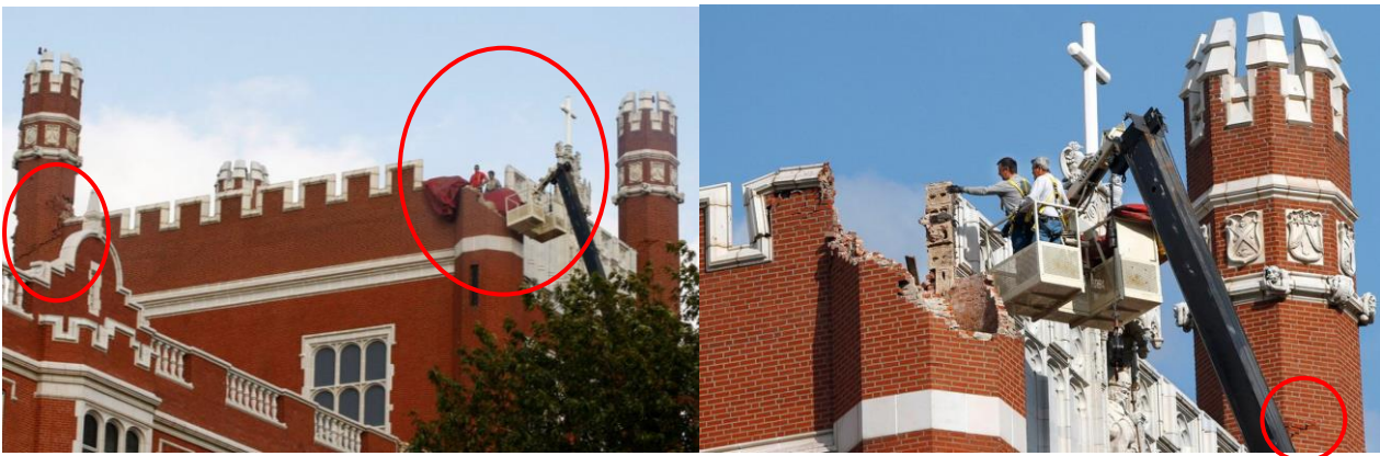
Figure A2.5.22. Damage to one of the towers of Benedictine Hall at St. Gregory's University in Shawnee. Photos by Jim Beckel, from http://newsok.com/gallery/articleid/3621379/pictures/1555036 .
