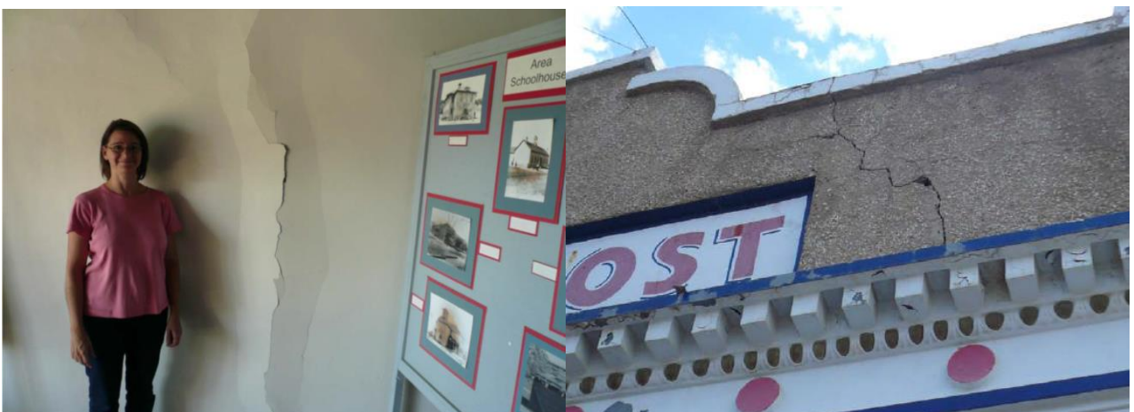
Figure A2.4.21. A 3 metres long vertical crack in the building of the Cokedale post office/city hall (left); cracked plaster on a façade in Segundo (Morgan & Morgan, 2011).
