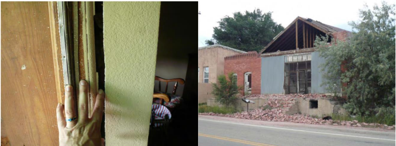
Figure A2.4.19. Damage observed at Segundo: on the left, the exterior wall pulled away approximately 2.5 cm from the interior wall; on the right, the front of this brick building collapsed (Morgan & Morgan, 2011).
