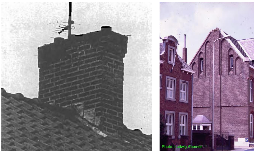
Figure A3.1.40. D2 (left) and D3 (right) damage to chimneys (Schwarz et al. , 2010).
