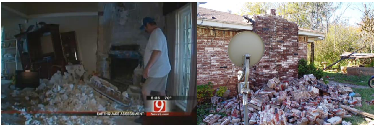
Figure A2.5.25. Complete collapse of a fireplace in the interior of a house in Sparks (left, News 9), and collapse of the top of a chimney of a house.
