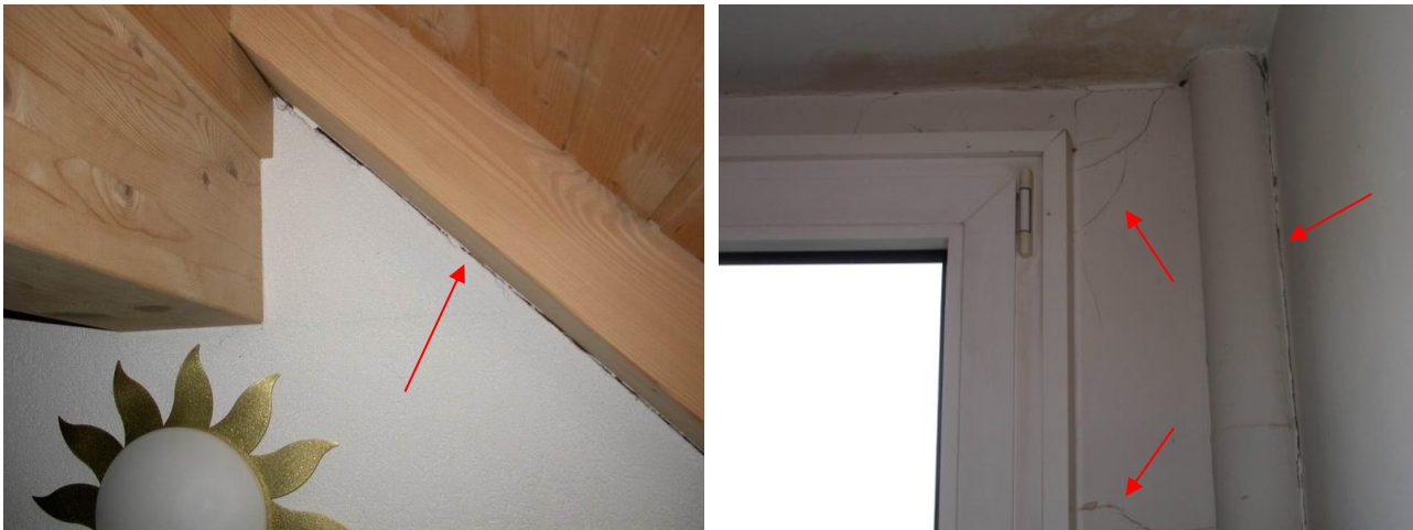
Figure A2.1.32. Crack in connection between wall and timber roof (left). Cracks in corner of a window (right).
