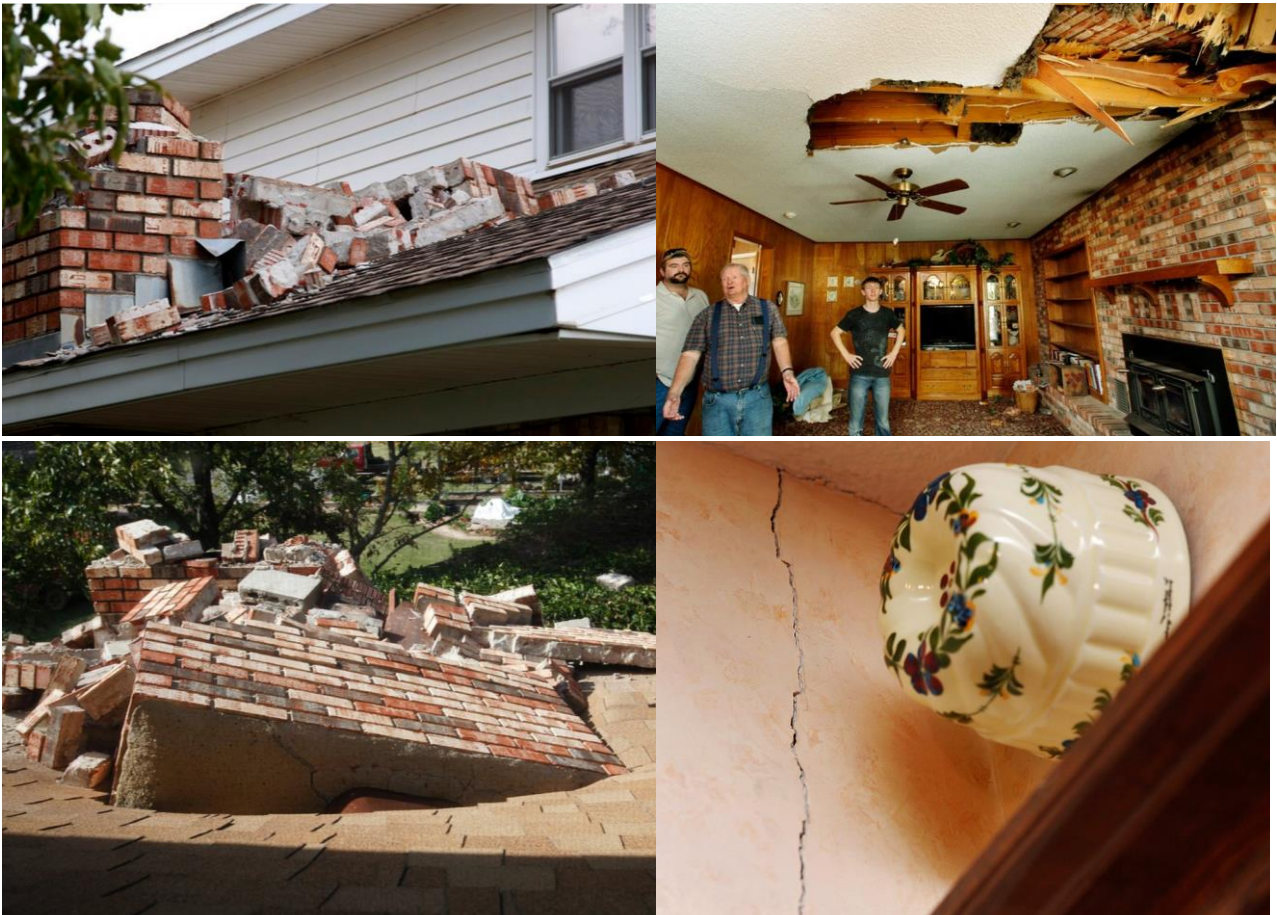
Figure A2.5.23. Damage to a house in Sparks. The chimney toppled over the roof. Photos by Sue Ogrocki(2015)
