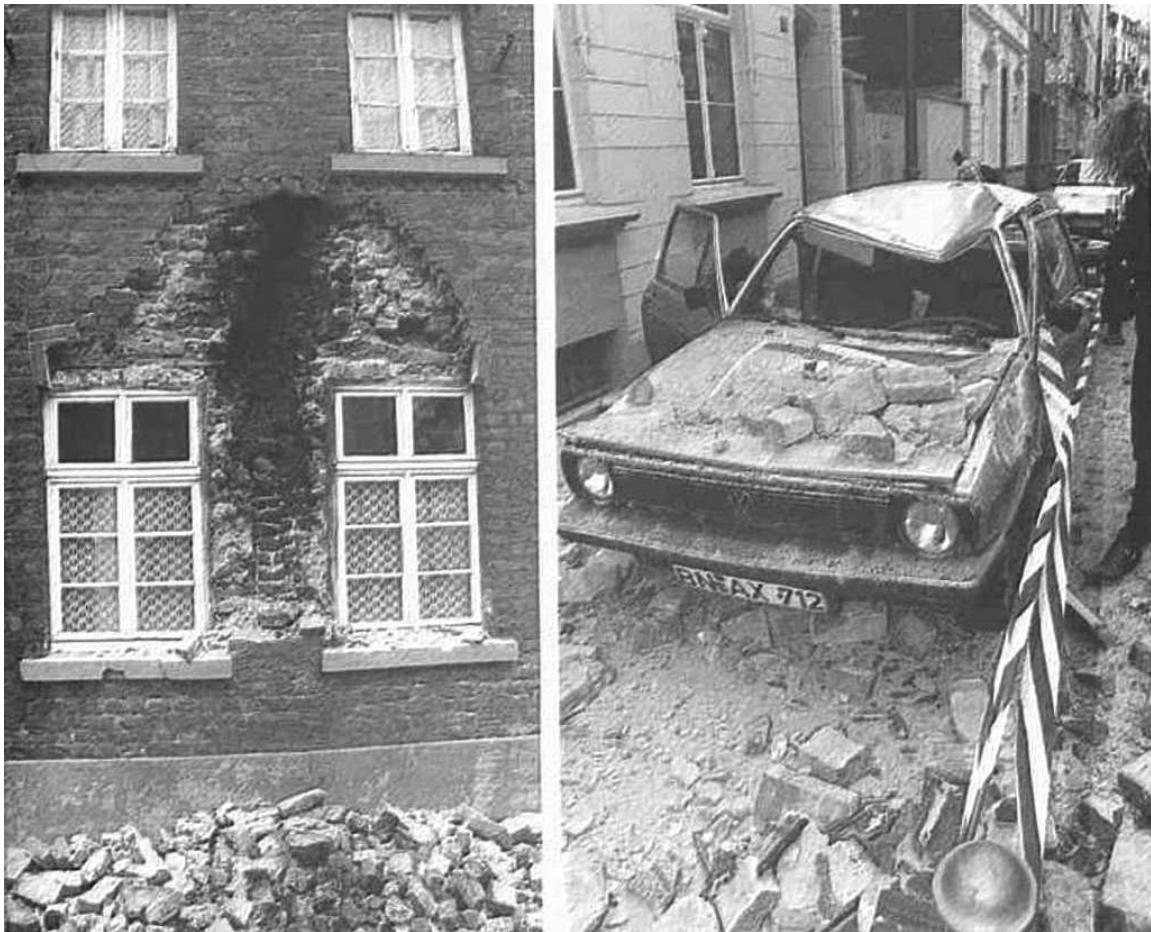
Figure A3.1.36. Damage to a residential house (left) and a car (right) in the city of Bonn (Germany). Photos copyright of Seismic Workgroup, St.-Michael-Gymnasium Monschau (2005)
