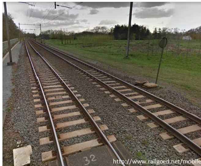
Figure 3. View of the at-grade railroad track, part of which was surveyed in this report.
