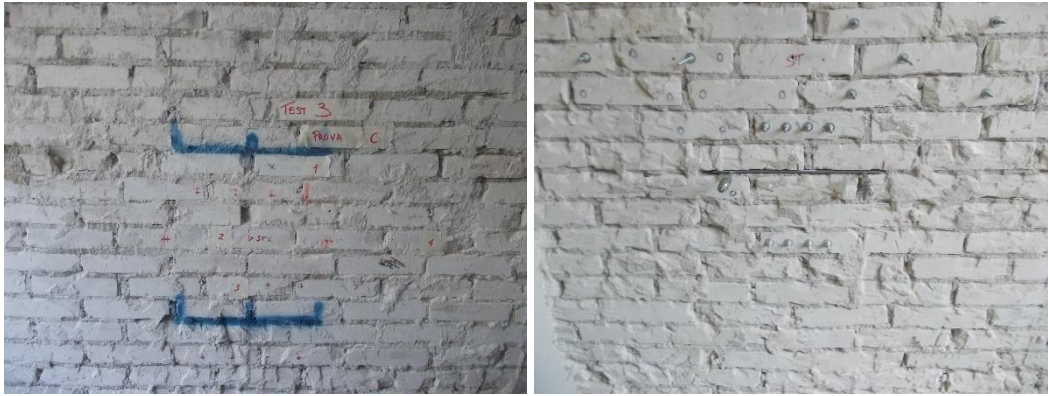
Figure 19. Example of Poor Quality masonry for the Calcium Silicate < 1985 typology.
