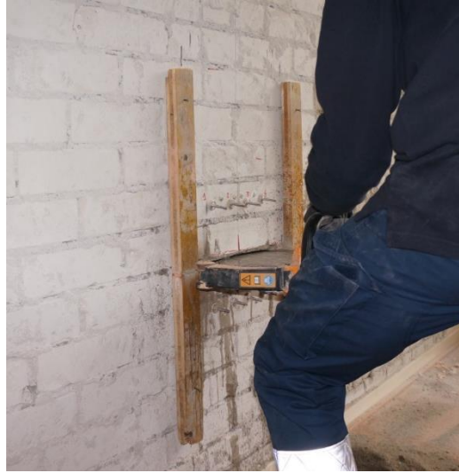
Figure 5. Single Flat Jack Test: cutting of the slot in the masonry wall.
