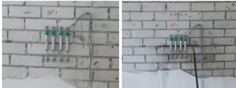
Figure 6. Single Flat Jack Test: measurement of the point distance (left) and performance of the test (right).
