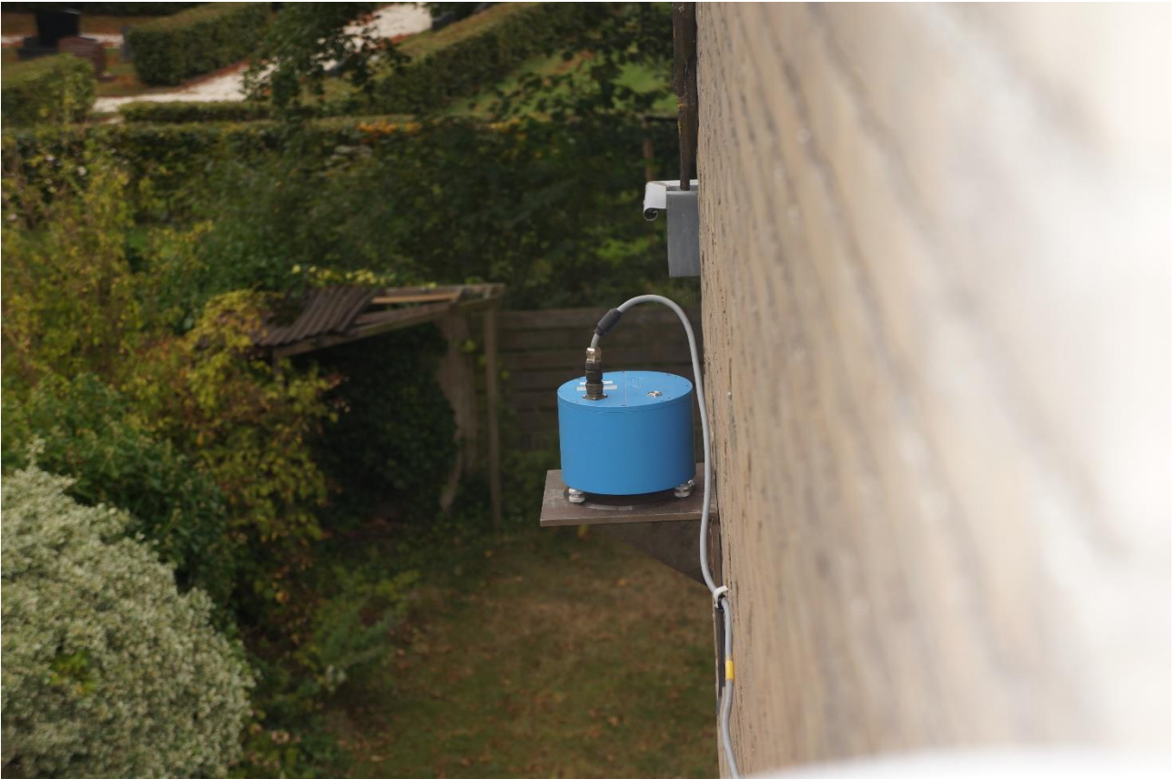
Figure 59. Geophone #7, 2 nd floor, configuration 3
