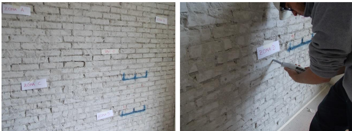
Figure 1. Rebound Hammer Test: identification of the 4 zones (left) and performance of the test (right).
