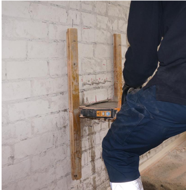
Figure 8. Single Flat Jack Test: cutting of the slot in the masonry wall.
