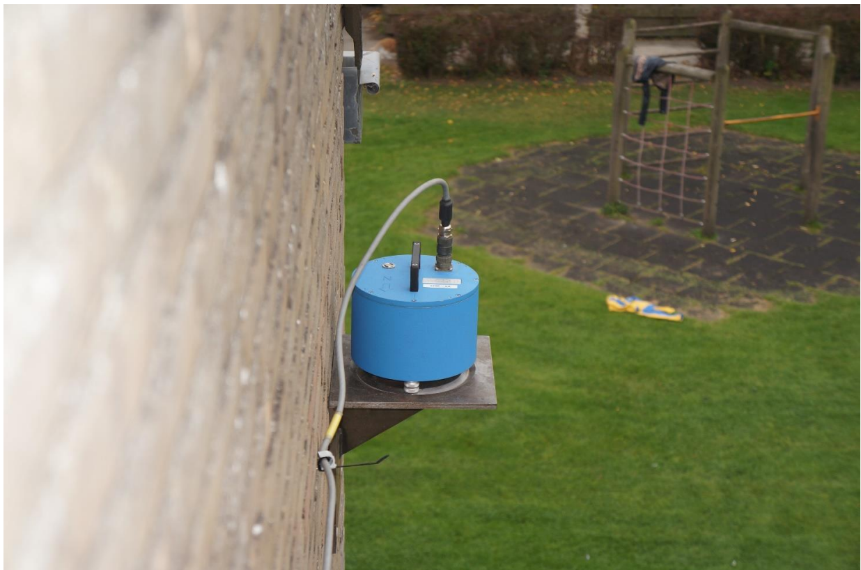
Figure 60. Geophone #9, 2 nd floor, configuration 3
