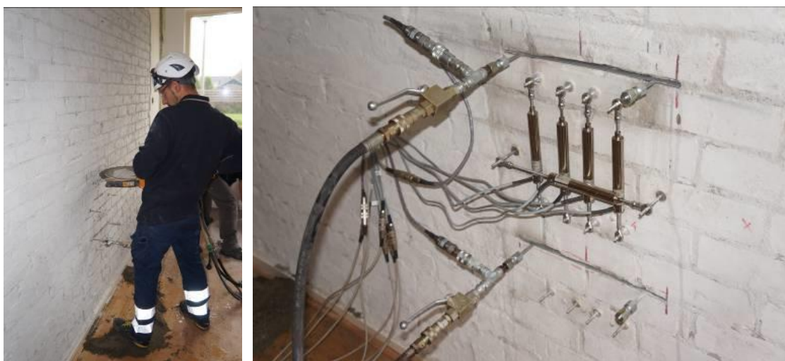
Figure 12. Double Flat Jack Test: cutting of the two slots (left) and test execution (right).
