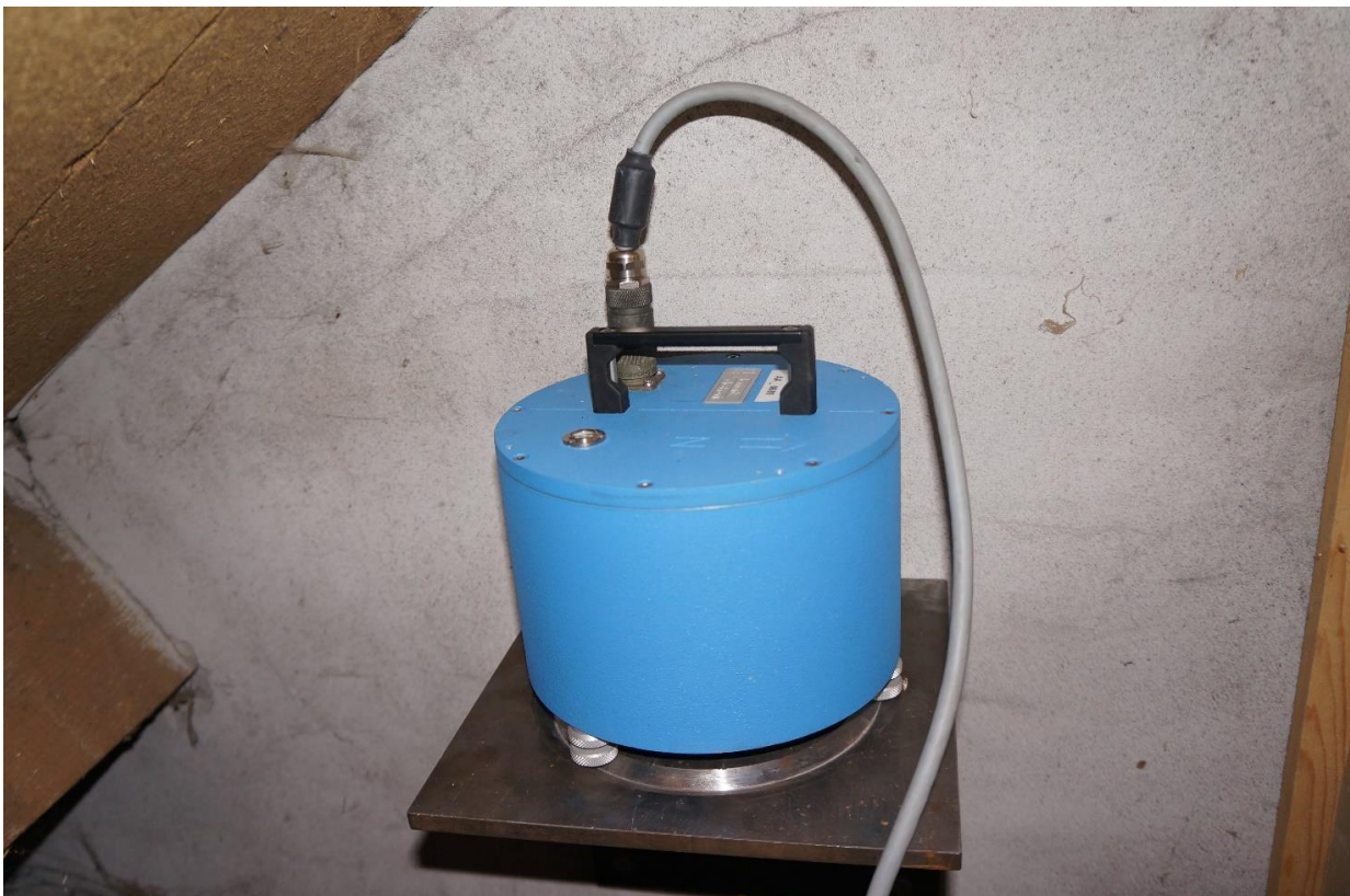
Figure 57. Geophone #9, 2 nd floor, configuration 2
