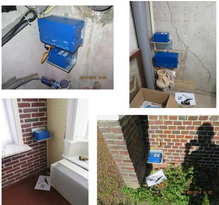
Figure 7.5. Examples of TNO instruments installed above ground level
