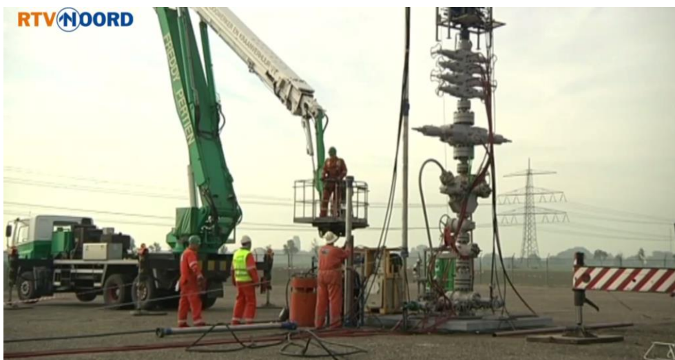
Figure 3.10 Installation of the temporary deep geophone string in well Stedum-1. .
